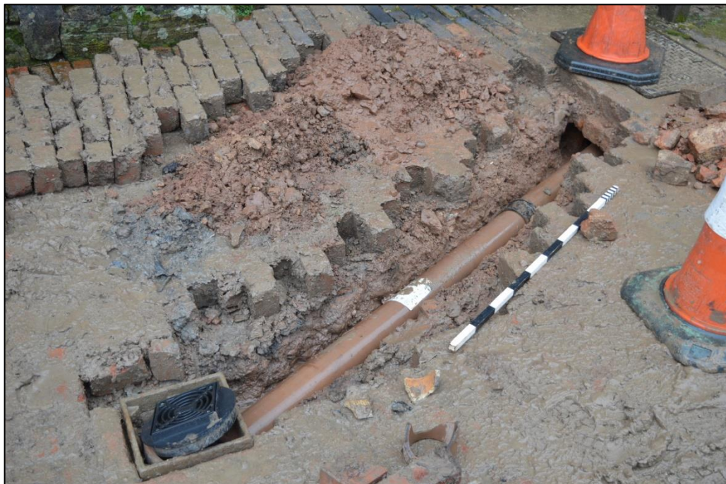
Fig. 4 View of the groundworks from the west following installation of the pipework. Photo CPAT 4607-0007
