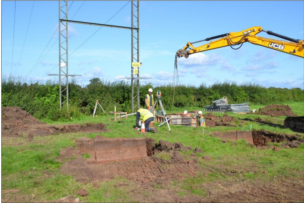
Fig. 7 The location of the new terminal tower, adjacent to tower BH29. Photo CPAT 4700-0021
