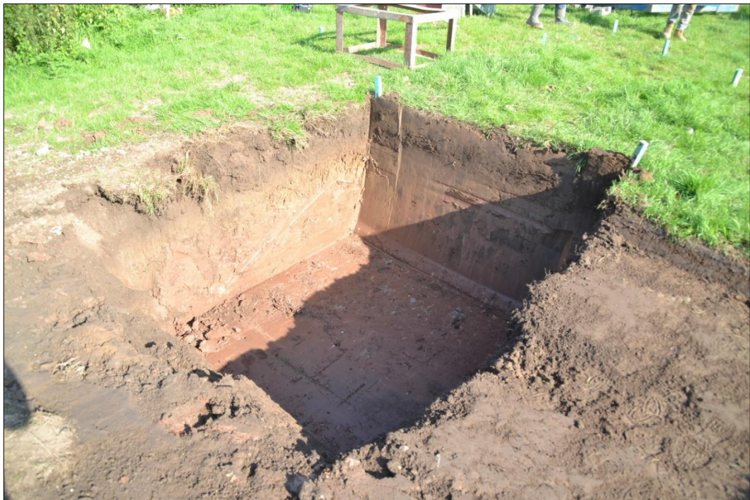
Fig. 6 One of four foundation trenches for the new terminal tower. Photo CPAT 4700-0016
