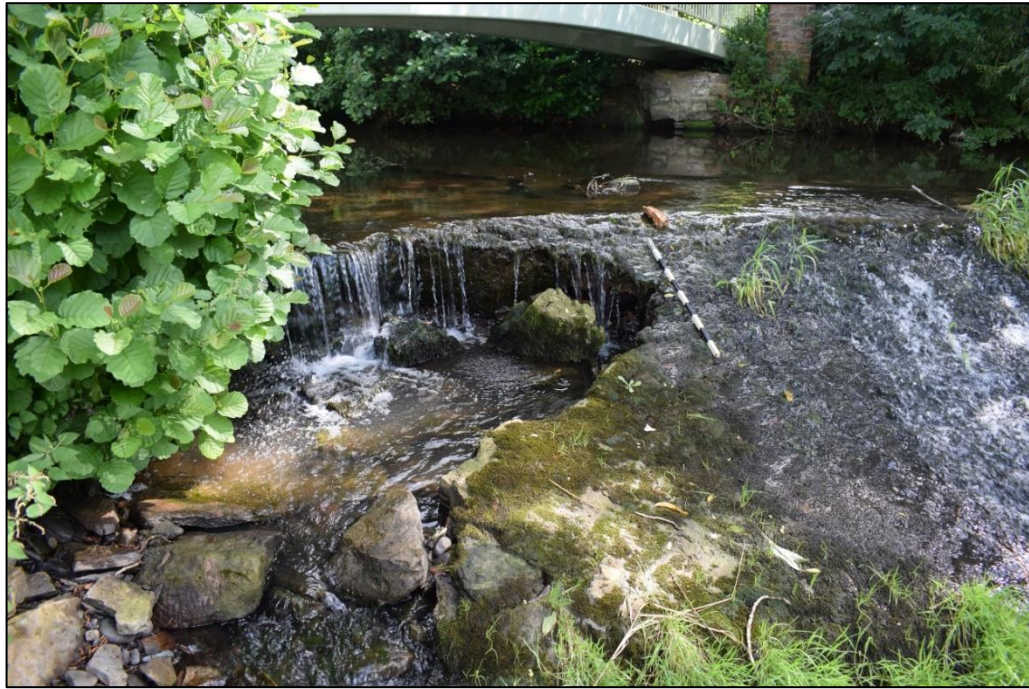
Fig. 5 Damage to the structure of the north-east end of the weir Photo CPAT 4684-004
