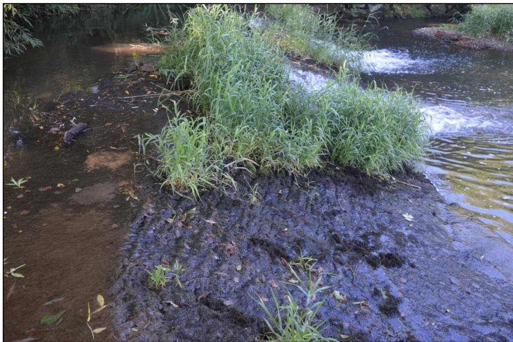
Fig. 4 Detail of the setts used to construct the weir ramp Photo CPAT 4684-074
