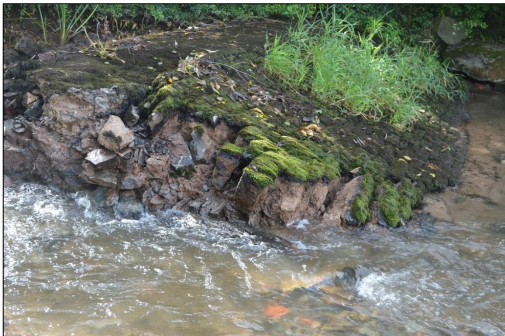
Fig. 11 View from the north-east showing the construction of the weir ramp Photo CPAT 4684-082
