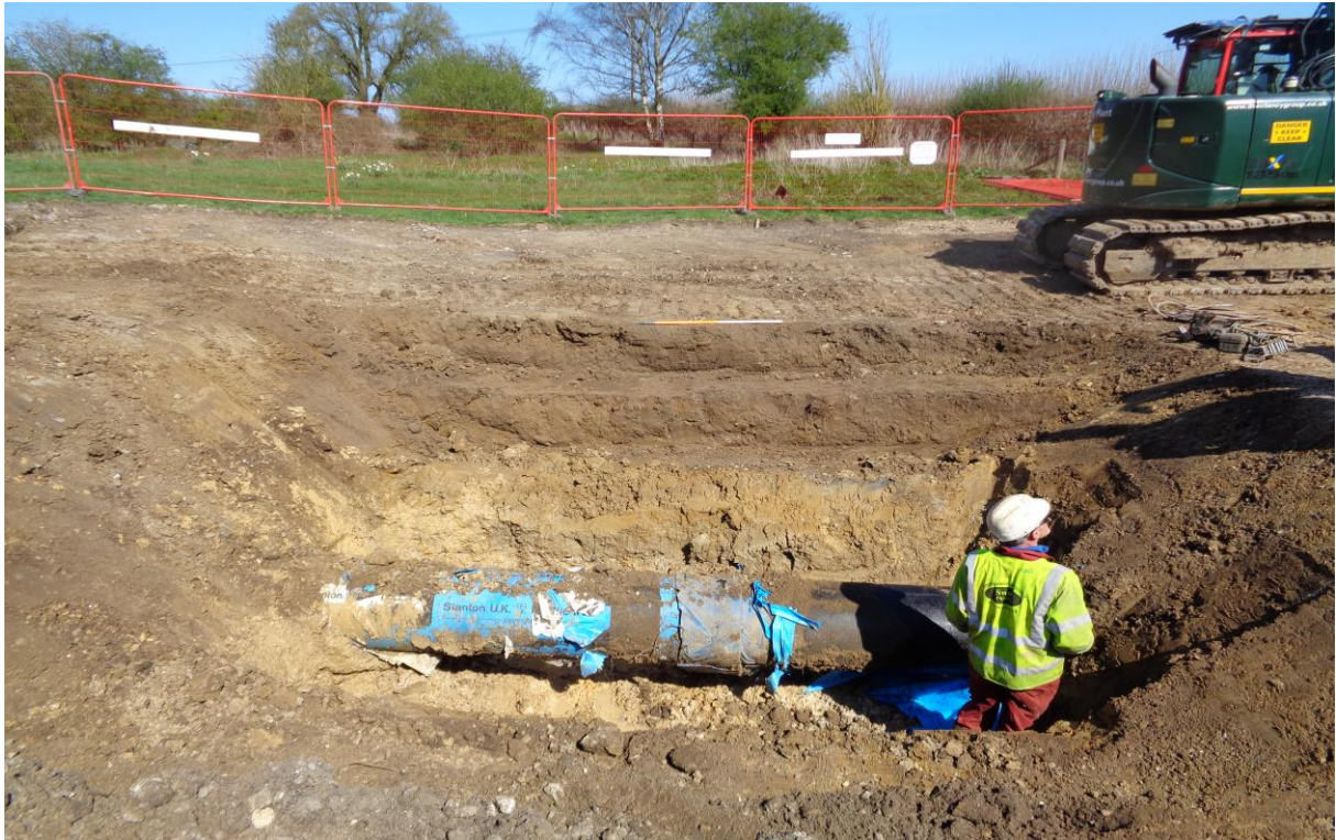
Plate 3: West-facing section of trial hole 2, Trench 002, showing original water mains pipe looking east (1m scale)
