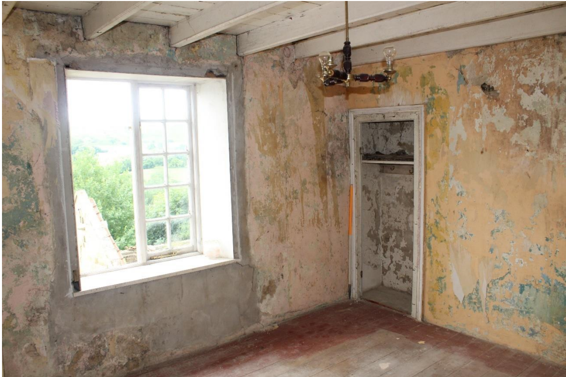
Plate 65: Internal view SW of 1 st floor bedroom showing two light casement window in N wall– Building No.1
