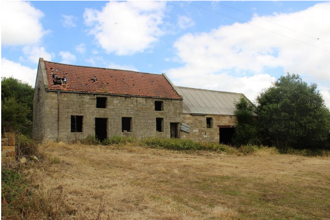
Plate 117: External oblique view NNE of the principal S facing elevation and W-facing elevation of Building No.4
