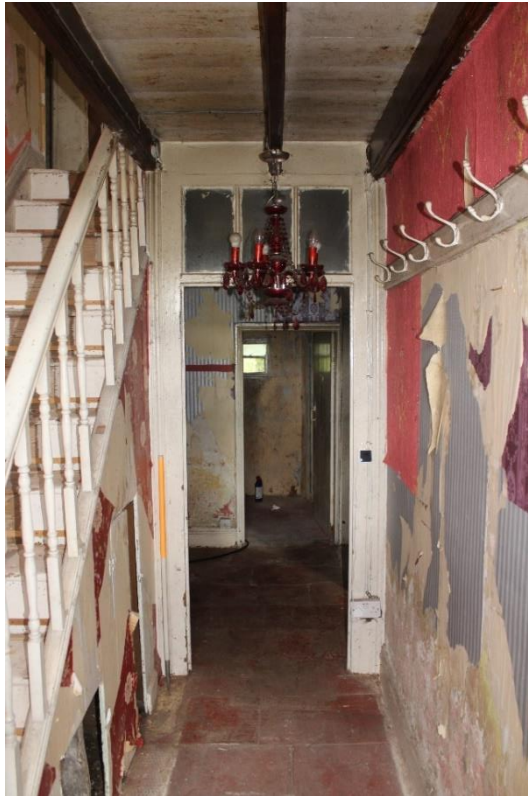
Plate 13: Internal view NNW along the ground floor central hall of the farmhouse – Building No. 1
