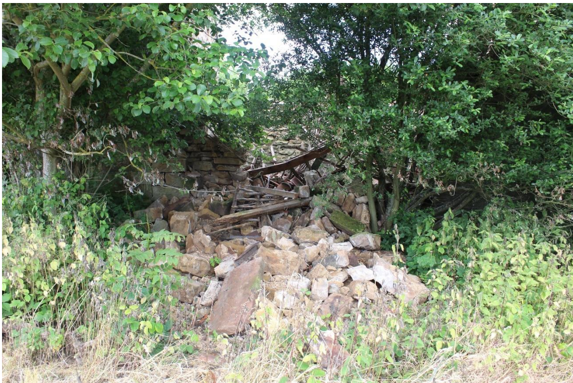
Plate 122: External views N of the collapsed third section of the S-facing principal elevation
