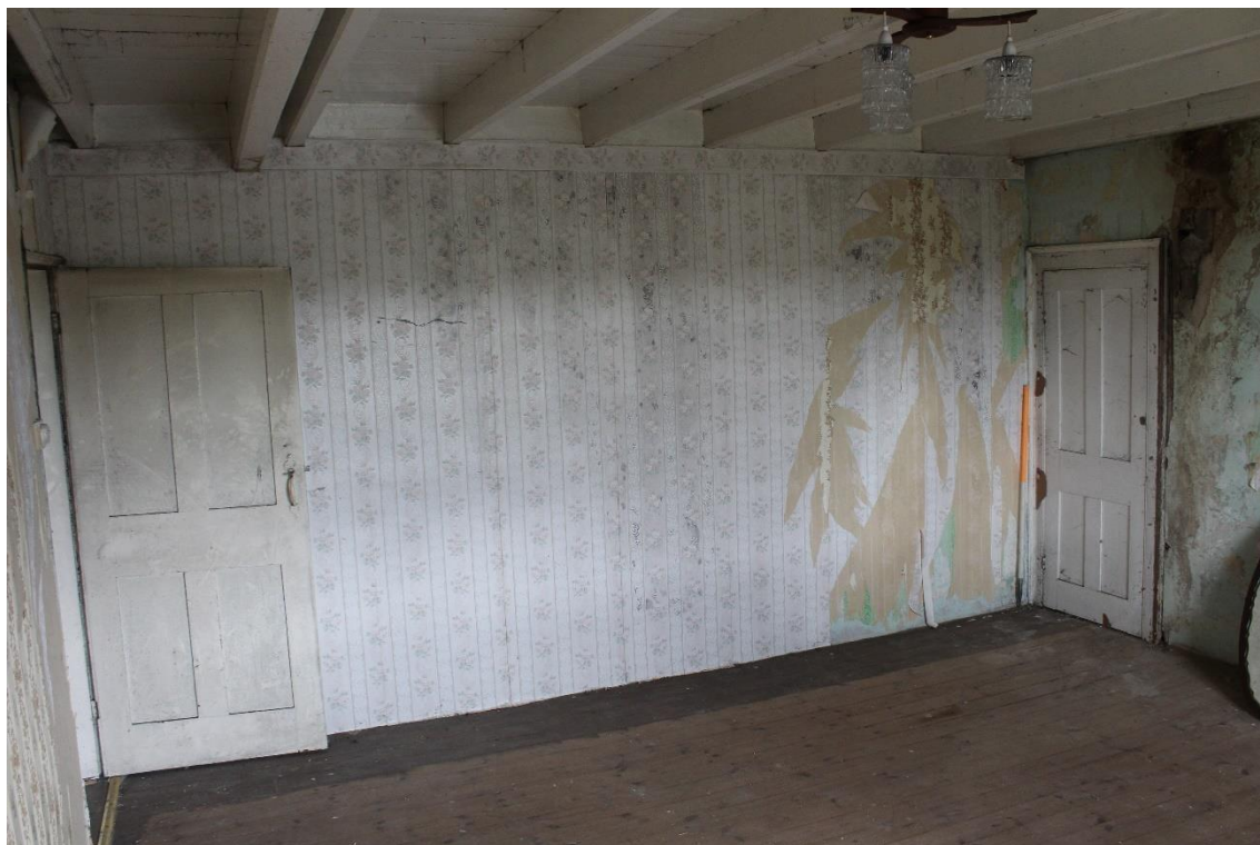
Plate 83: Internal view NNE of 1 st floor fourth bedroom showing locked storage alcove – Building No.1
