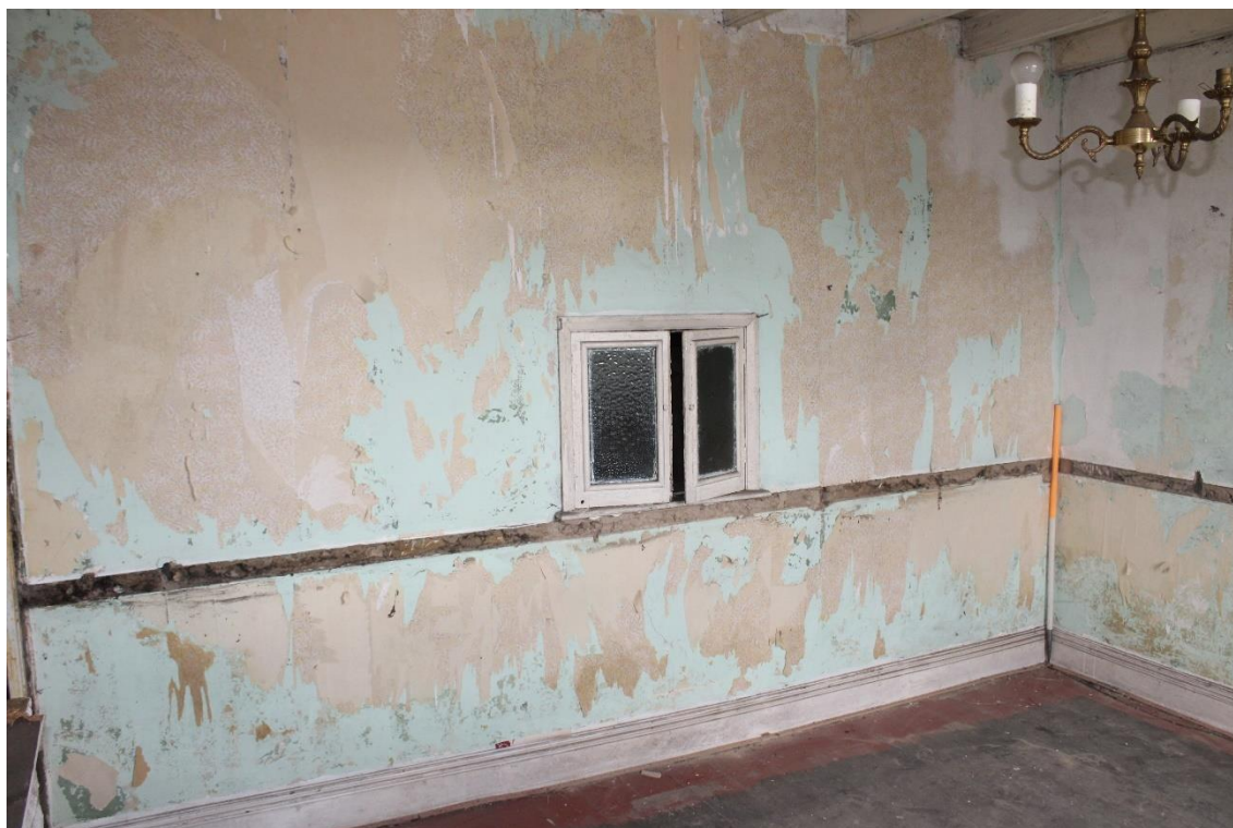
Plate 22: internal view ESE within ground floor living room showing service hatch through to the kitchen – Building No. 1
