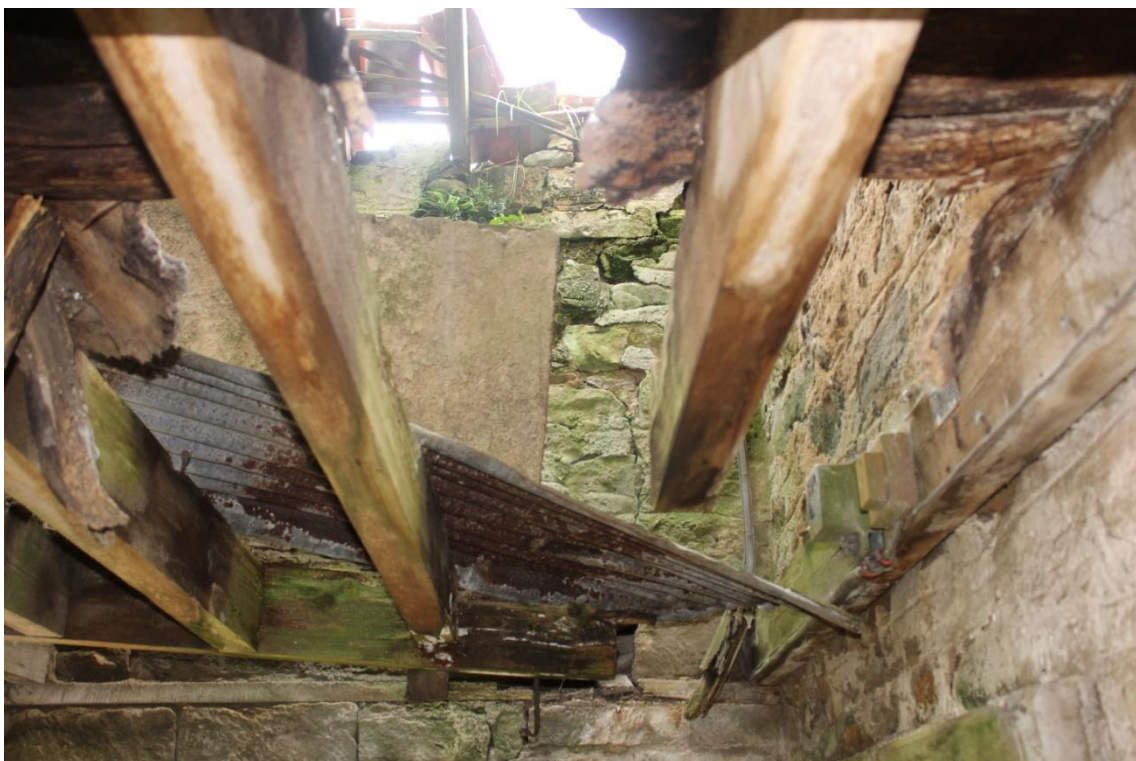
Plate 132: Internal view S of rotten ceiling timbers within the first compartment of Building No.4
