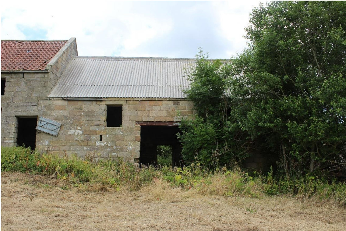
Plate 121: External views N of the second section of the S-facing principal elevation
