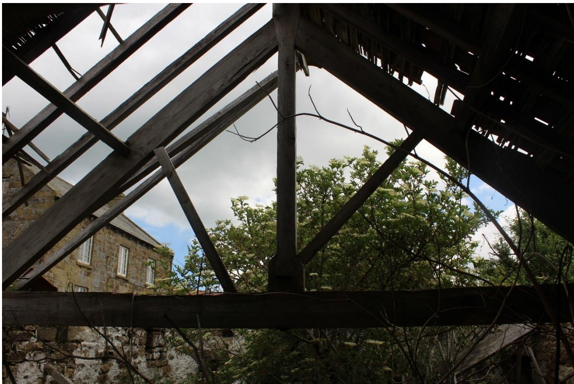
Plate 108: Internal view ENE of surviving king post truss with W compartment of Building No. 2
