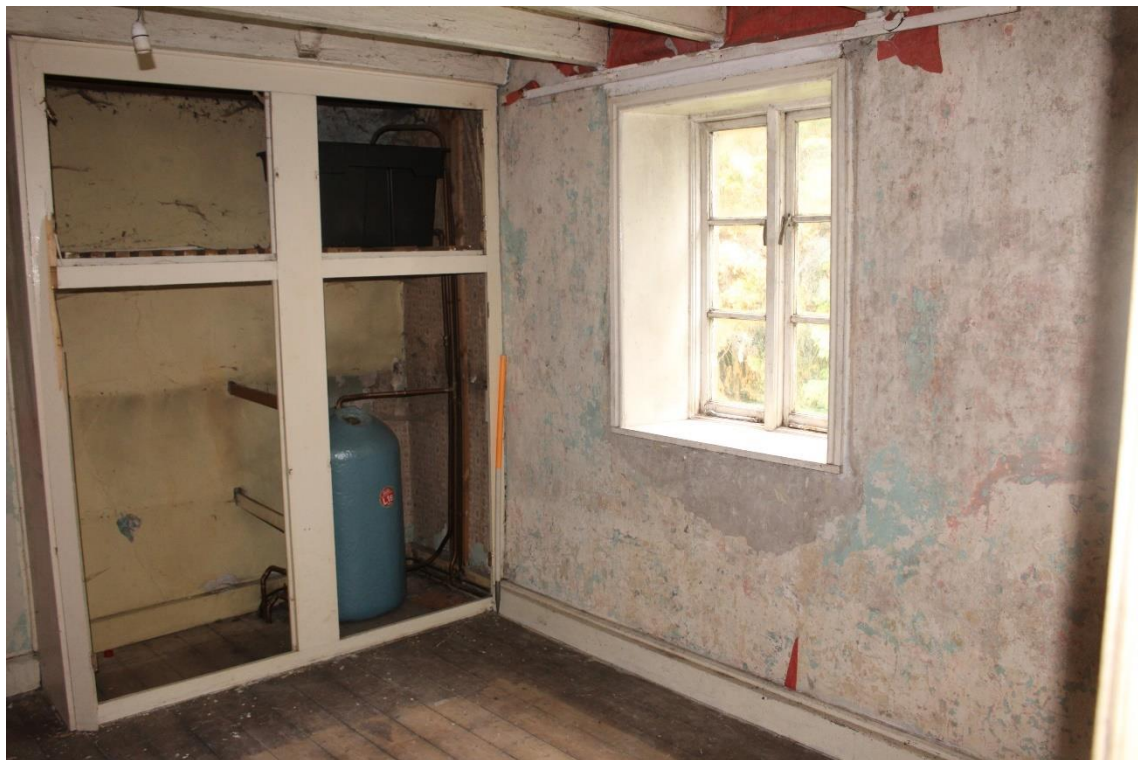
Plate 72: Internal view SW of 1 st floor second bedroom showing two light casement window within N wall – Building No.1
