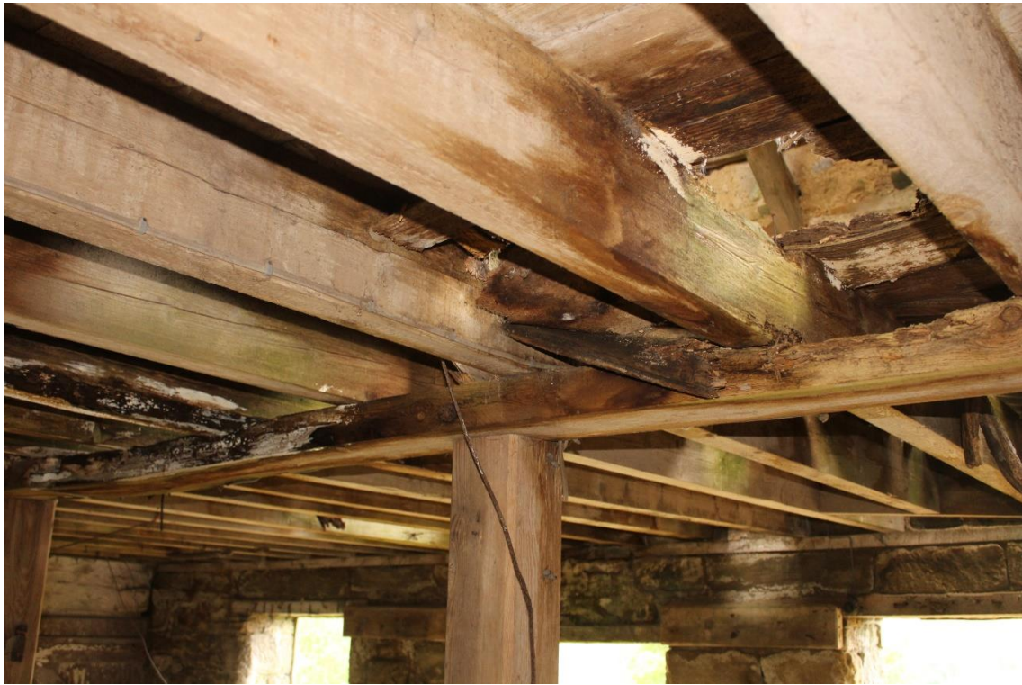
Plate 131: Internal view ESE of rotten ceiling timbers within the first compartment of Building No.4
