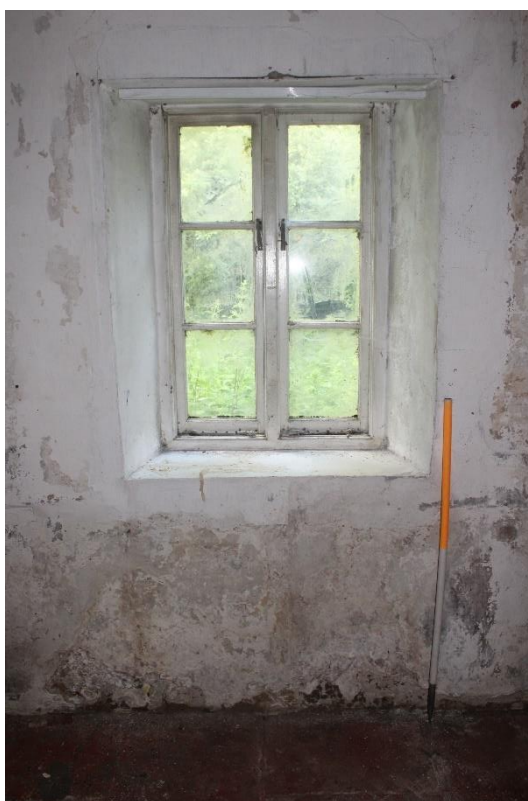
Plate 36: internal view NNW within ground floor storage room showing casement window within N wall— Building No. 1
