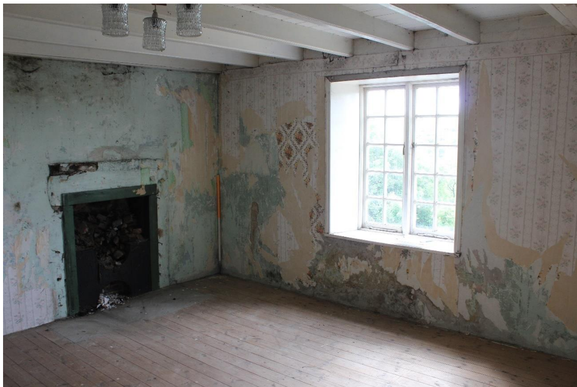
Plate 81: Internal view SE of 1 st floor fourth bedroom showing two light casement window with S wall – Building No.1
