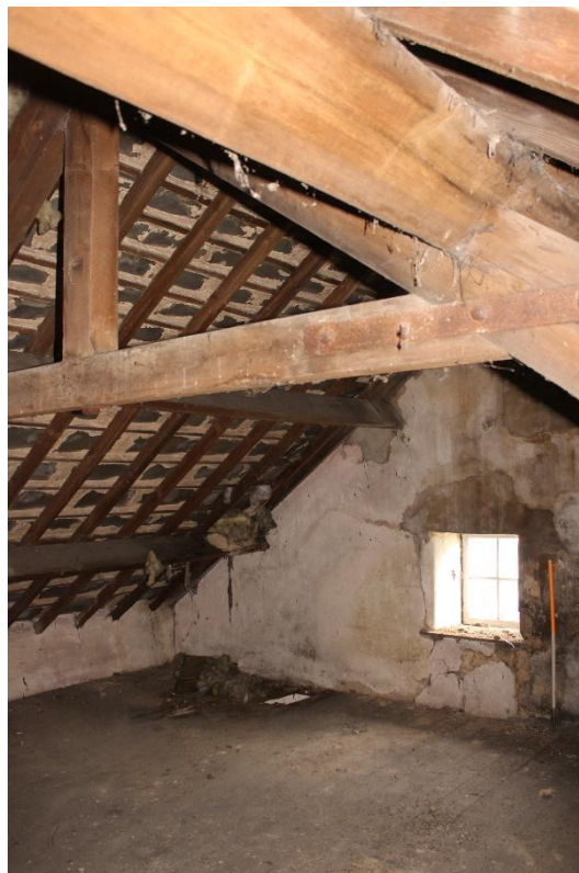
Plate 94: Internal oblique view SSW of attic/roof space showing single light casement window – Building No.1
