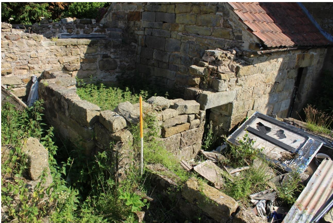
Plate 58: internal view NNE of pigsties E partition – showing half height door opening onto yard Building No. 1
