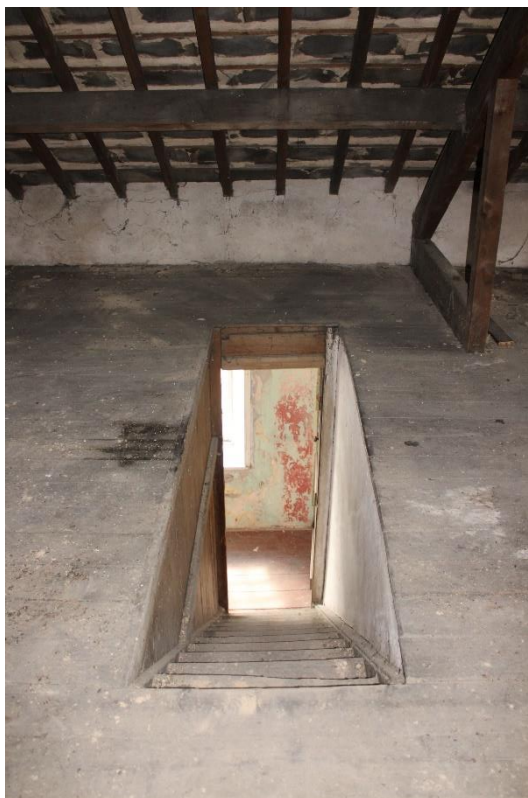
Plate 88: Internal view SSE of stair case leading to the 1 st floor from the attic/roof space – Building No.1
