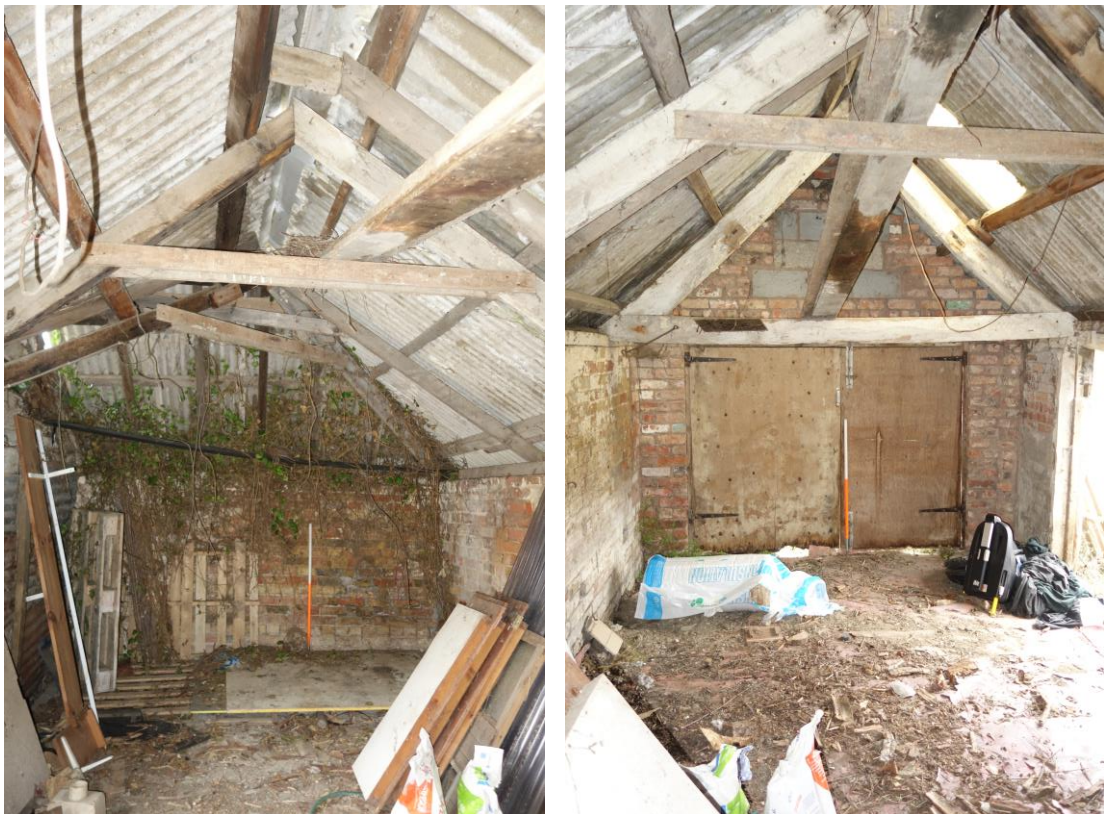
Plate 25: Internal view SE showing southeastern portion of two-bay range and roof trusses
