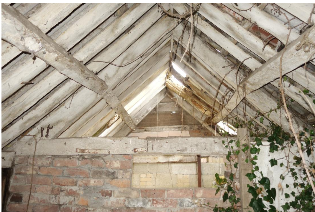
Plate 21: View looking NE showing detail of roof truss at NE end of two-bay compartment
