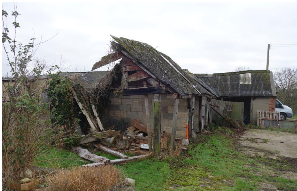
Plate 3: View looking SSW towards the collapsed NE-gable end of the L-plan outbuilding at Brickhouse Farm
