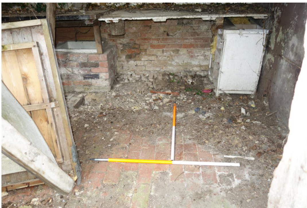
Plate 24: Internal view looking SE showing detail of brick paved floor with area of disturbed stone cobbling against rear wall
