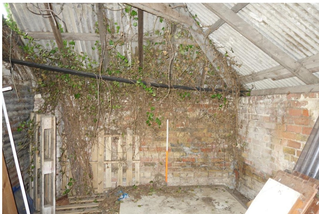
Plate 29: Internal view showing SE end of two-bay range with whitewashed walls and concrete screed floor
