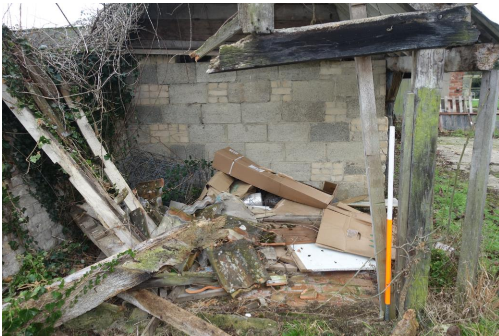
Plate 11: View looking SW showing detail of collapsed NE compartment of four-bay range with brick paved floor
