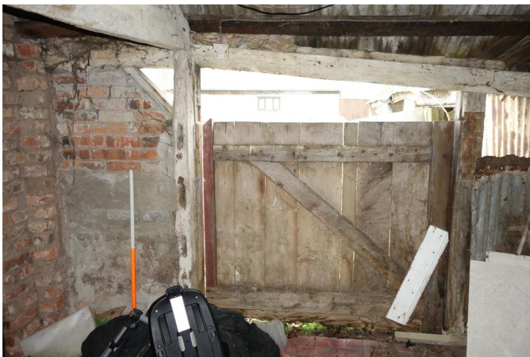
Plate 32: Internal view NE showing stall door in NE wall of two bay range with section of brick walling to left of picture
