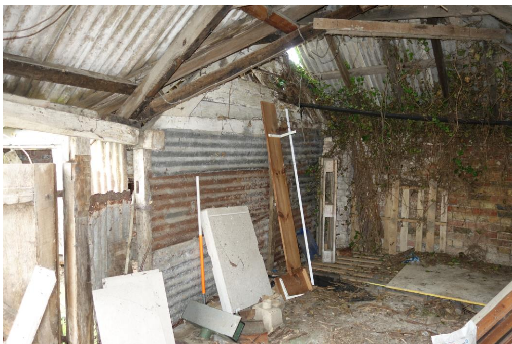
Plate 27: Internal view E showing juncture between SW gable end of four-bay range and two-bay structure
