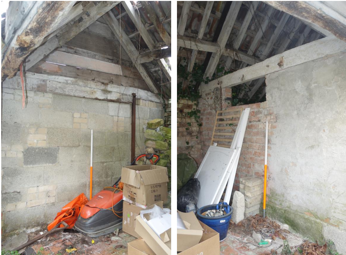
Plate 12: Internal view looking ENE showing concrete breeze block wall and roof trusses in second compartment at NE end of four-bay range
