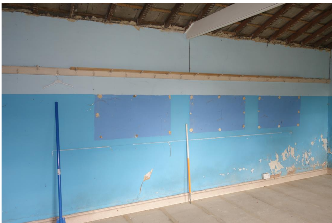
Plate 42: Internal view looking NE showing detail of rear wall of former schoolroom with coat rack with hooks attached to wall
