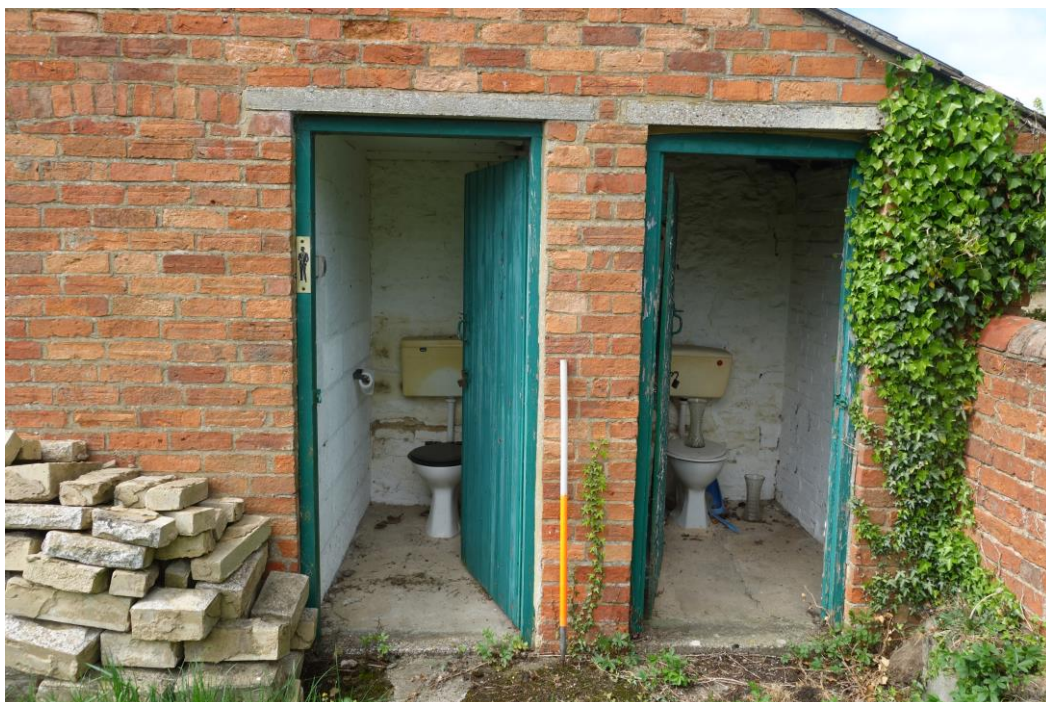
Plate 15: View looking SW showing detail of modern doors inserted for toilet compartments at NE end of schoolroom
