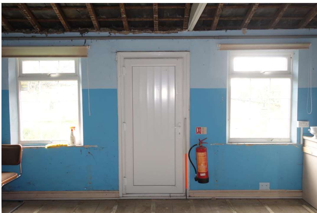
Plate 40: Internal view looking SE showing modern uPVC door and casement windows in SE wall of former schoolroom
