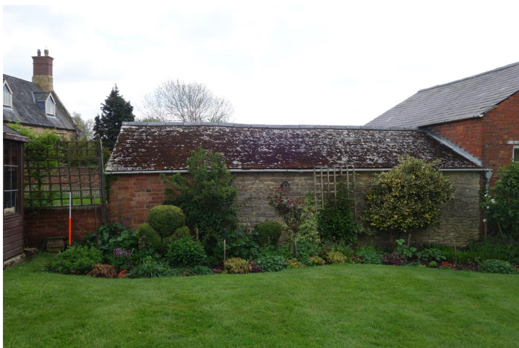
Plate 16: View looking SE showing rear (NW-facing) elevation of schoolroom annexe, constructed of roughly coursed rubble masonry with later brick extension to left of picture
