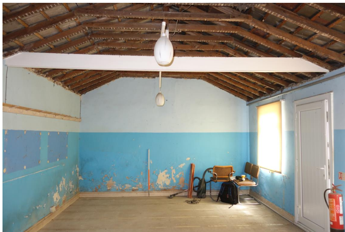
Plate 35: Internal view of hall (former schoolroom) looking NE showing boarded floor and roof trusses
