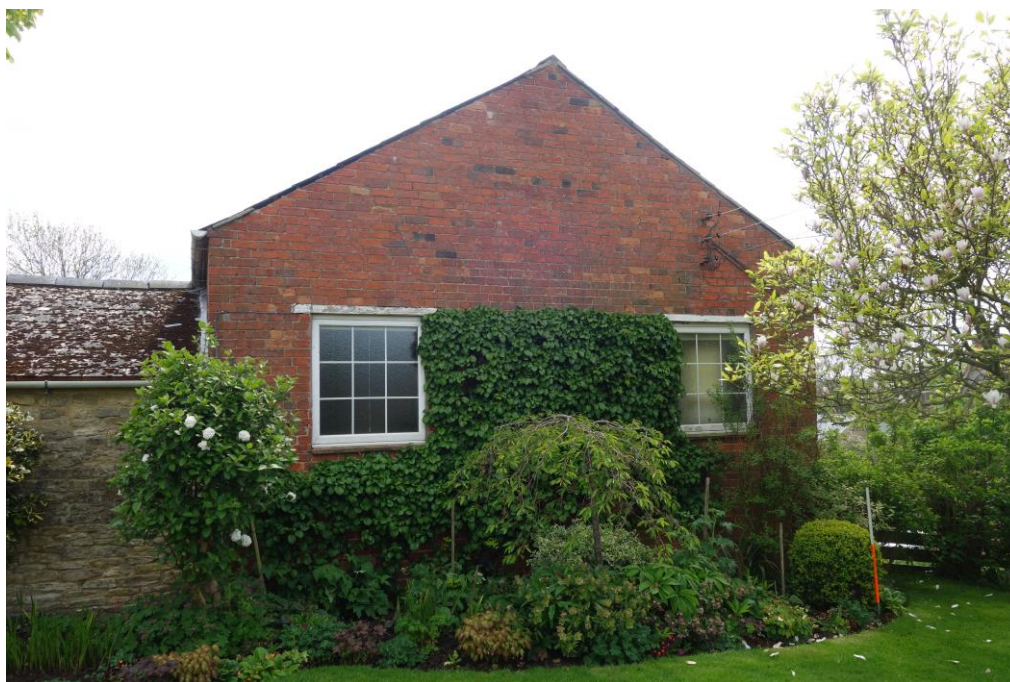
Plate 11: View looking SE showing rear (NW-facing) elevation of chapel with casement windows
