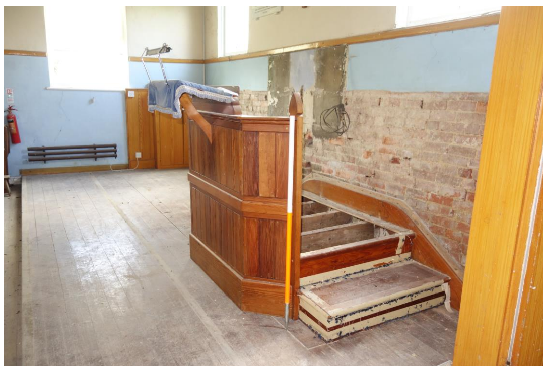
Plate 25: View looking WNW showing detail of pulpit at NW end of chapel
