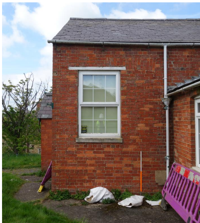
Plate 9: View looking WSW showing NE facing elevation of chapel with blocked window to left of modern glazed casement
