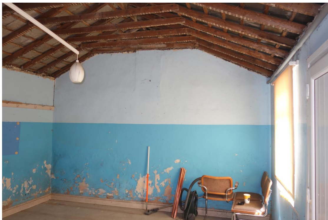
Plate 39: Internal view looking NE towards NE end of former schoolroom showing outline of former chimneystack in wall
