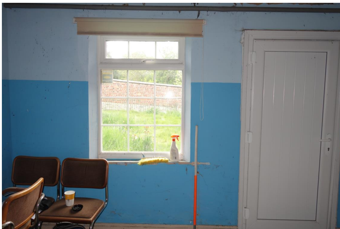
Plate 41: Internal view looking SE showing detail of casement window to left of door in SE wall of former schoolroom
