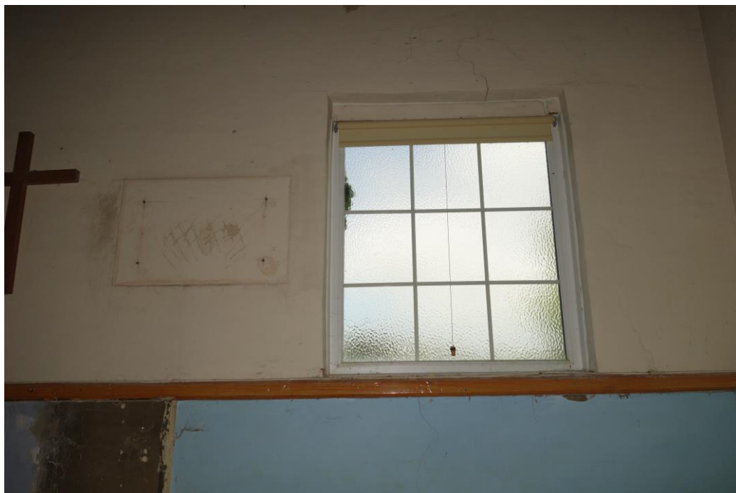
Plate 28: View NW showing detail of casement window in right hand corner of NW wall of chapel
