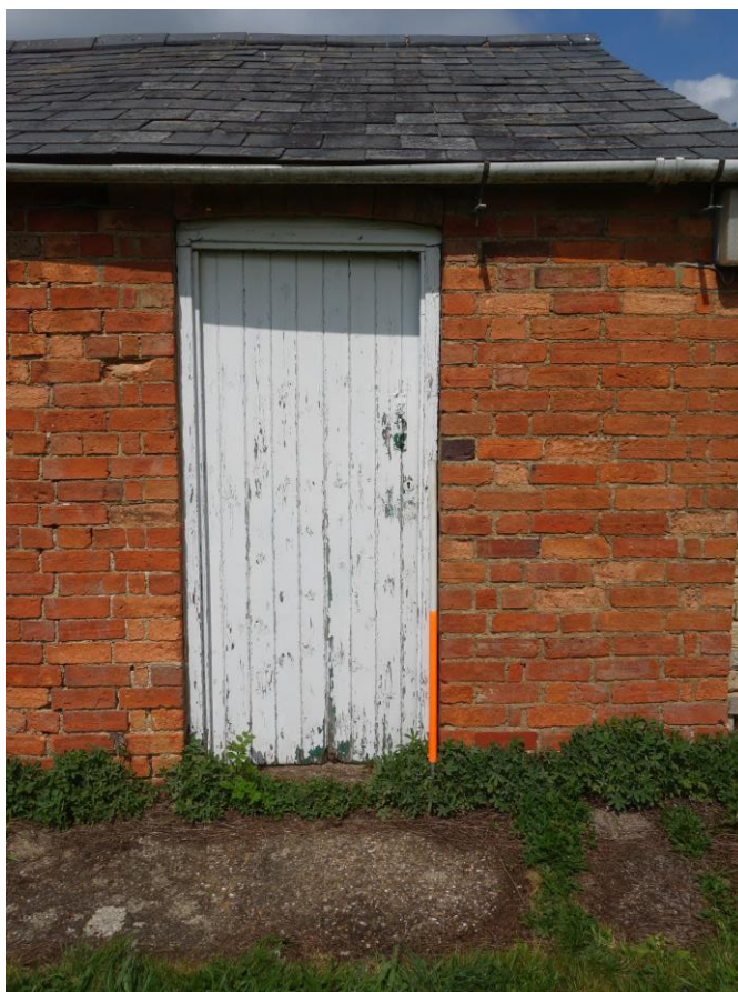
Plate 13: View looking NW showing detail of doorway at NE end of front elevation of schoolroom, with construction break visible to left of doorway
