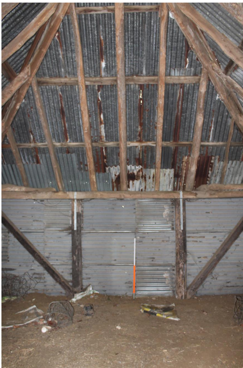
Plate 15: View looking NW showing detail of timber-framing and roof structure at NW end of shed
