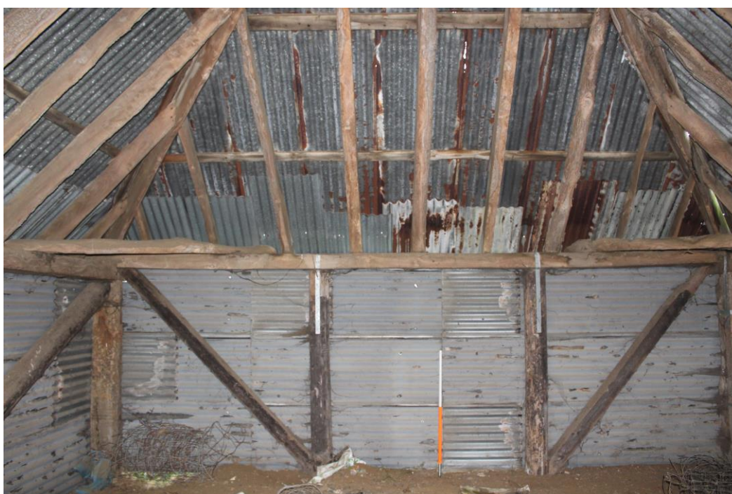
Plate 14: View looking NW towards NW end of shed showing diagonal wall braces with metal straps with horizontal angled timbers linking the wallplates
