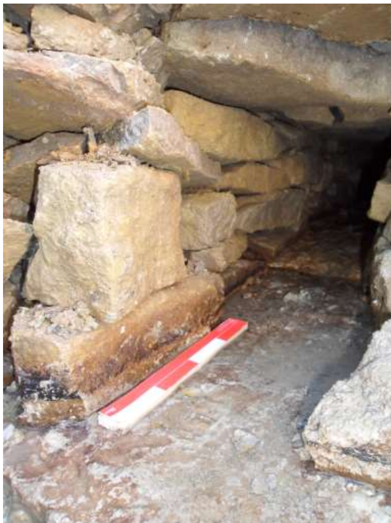
Plate 32: View S showing internal E wall construction of masonry culvert (20cm scale)
