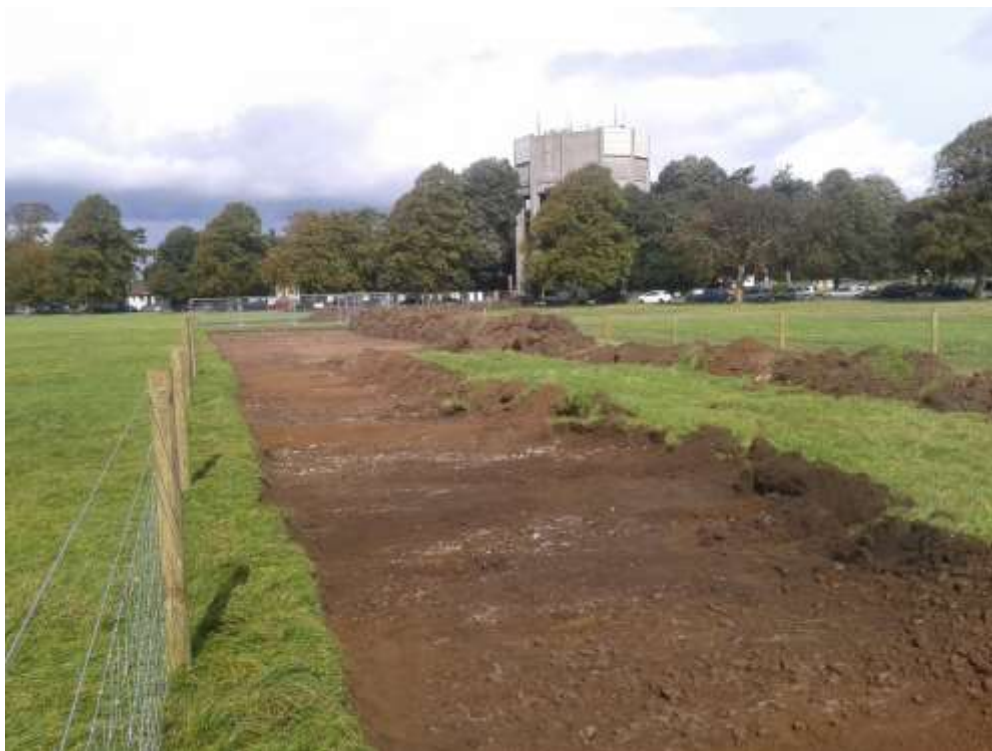
Plate 44: View NW towards Stoke Road and the Water Tower showing topsoil strip on Clifton Down
