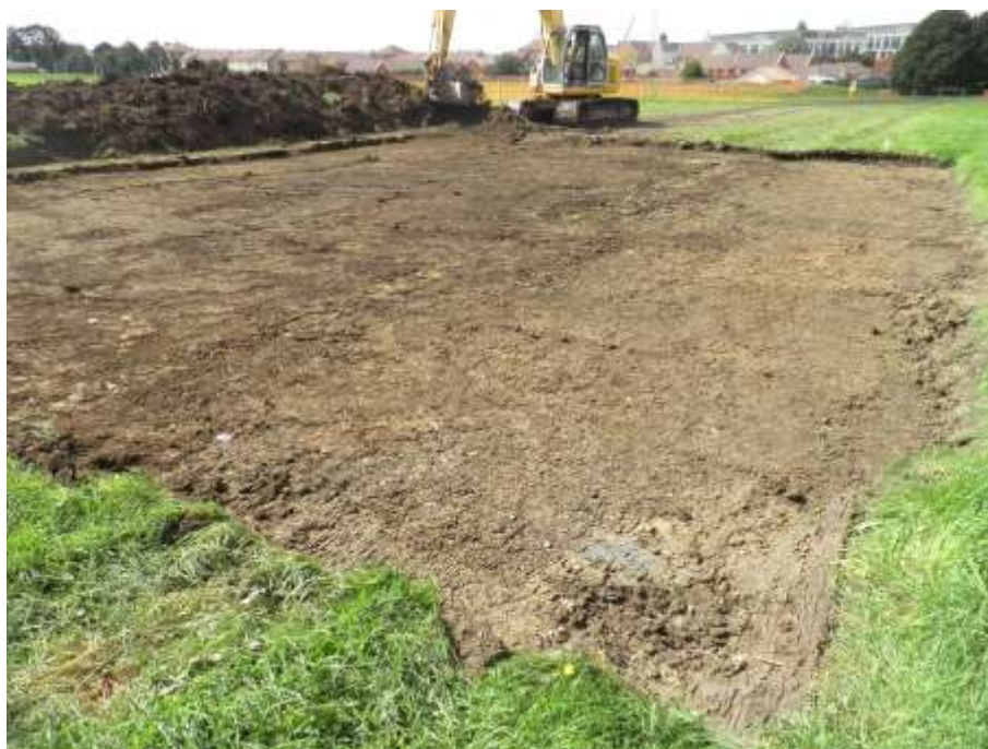
Plate 33: View SW showing initial topsoil strip in the NE corner of the playing fields. Clean turf and thin topsoil (101) removed to reveal layer (102) (old loam/subsoil & 19 th century debris)
