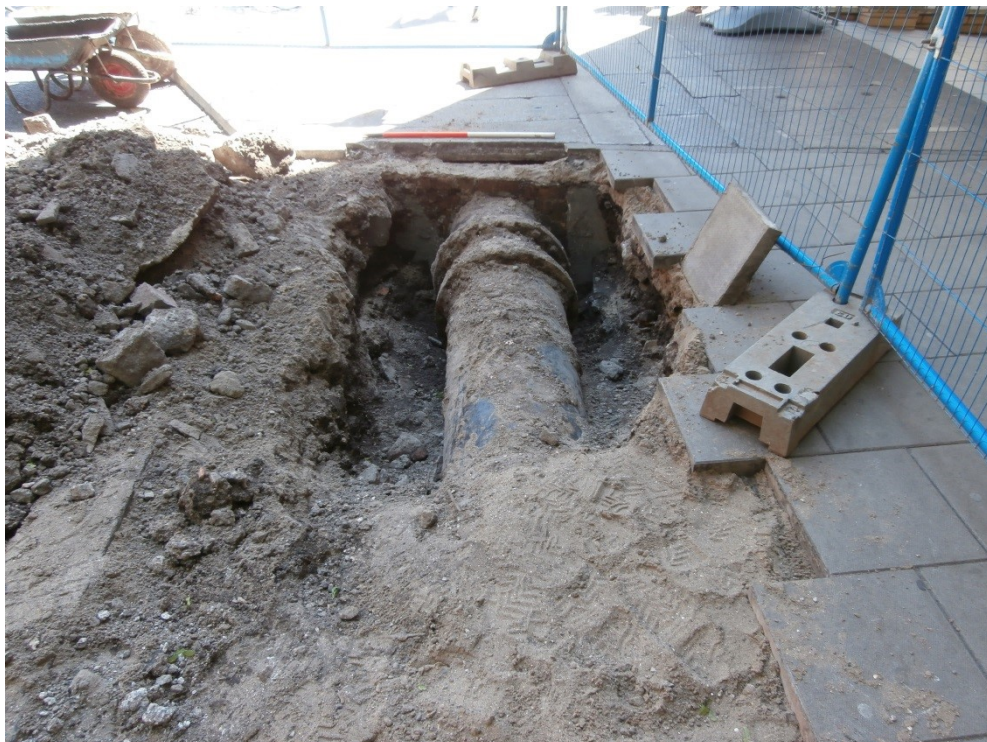
Plate 28: View to the S of Trench 11 showing the exposed 19 th -century water main
