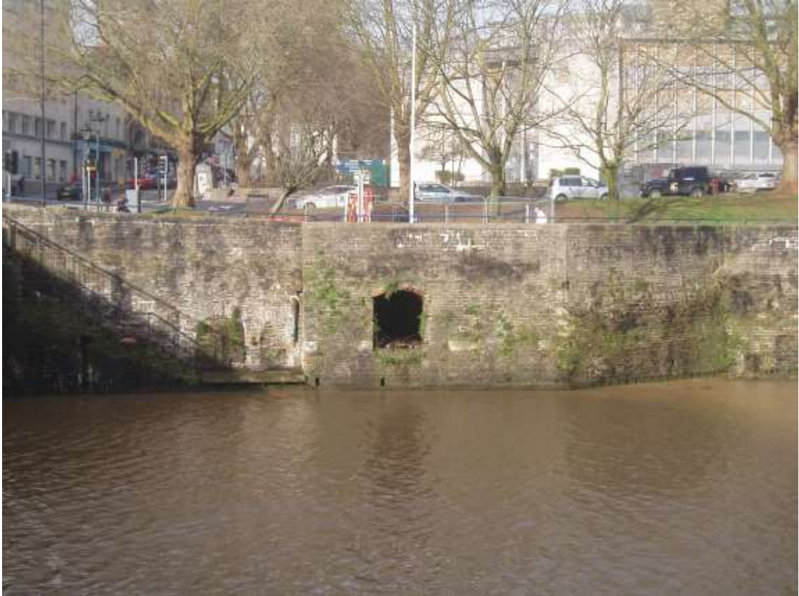
Plate 4: View looking N showing segmental-headed archway leading to chamber set into the thickness of the early 19 th century harbour walls
