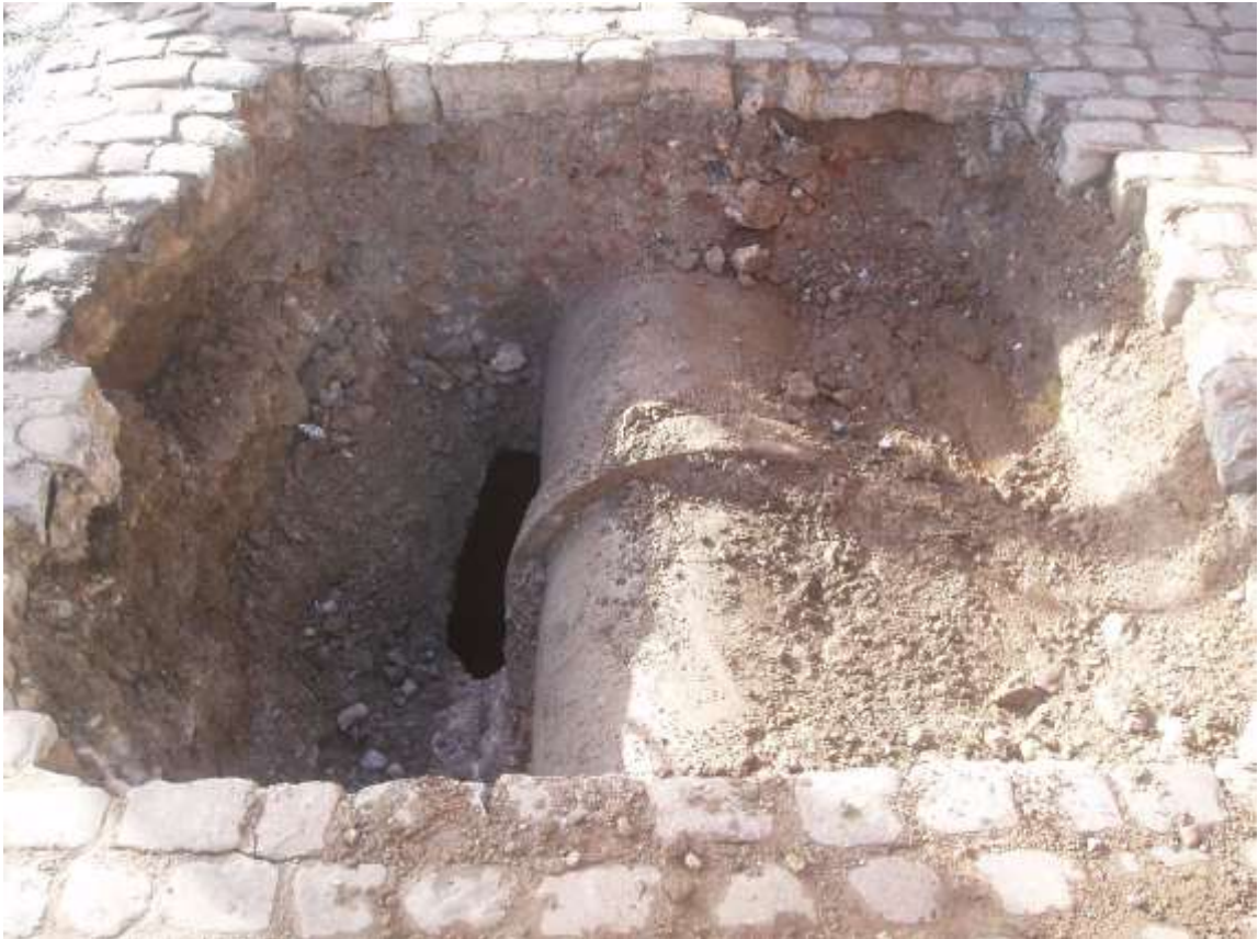
Plate 3: View looking NE showing void in Pit 2 beneath 1885 water main
