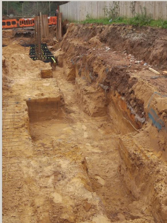
Plate 3: View SSE of pile-pit trenching along the SW extent of site, showing the depths attained during the second stage of ground works
