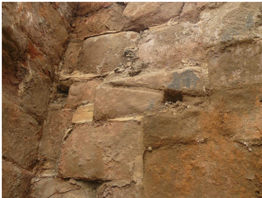
Plate 5: Detail of Town Wall showing squared indentations in the masonry, possibly putlog holes
