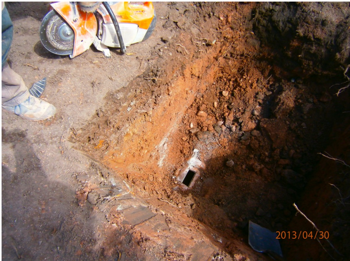
Plate 1: Facing North-East: the unmapped sewer, surrounding stratigraphy largely still the disturbed backfill of the original service trench.
