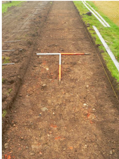
Plate 3: View E of levelling (008) adjacent to N elevation of wall and gardener's cottage
