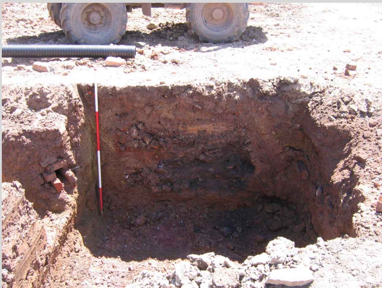
Plate 6: North-facing section of Manhole 1 (trench depth 1.85m) showing the remains of a possible brick kiln [212] and associated fill (211) consisting of charcoal, stone and CBM, possibly the source of spread (188). Note also the small brick feature [215] to the left of the ranging rod which appeared to be the remains of a 19 th century drain
