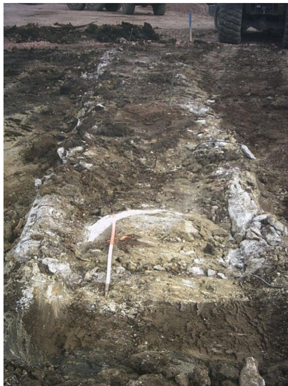
Plate 7: View SE showing steel reinforced base of possible boundary fence in SW 'turning' area
