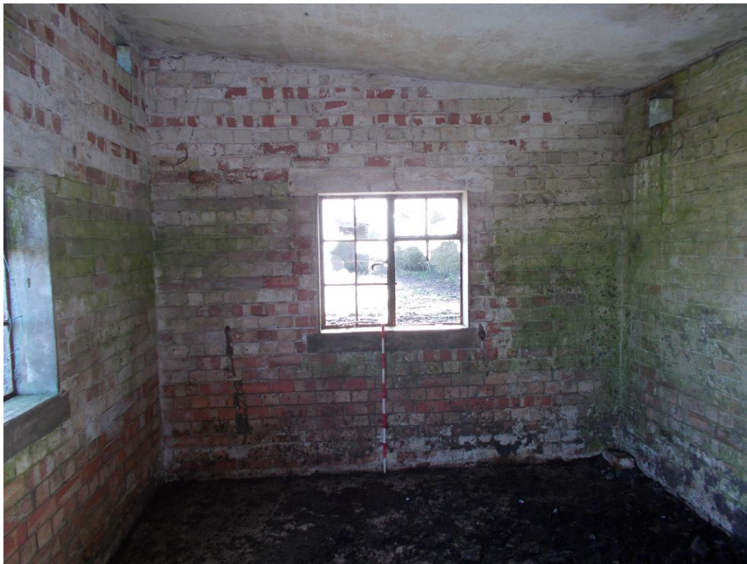
Plate 9: Internal view looking SE within compartment at SE end of Building A
