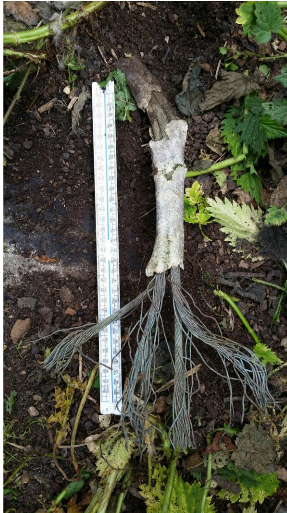
Plate 20: Detail showing heavy copper cabling projecting from plinth of Building D
