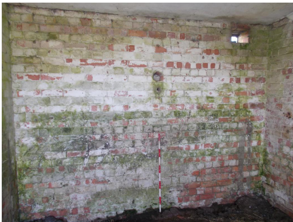
Plate 14: Internal view looking SW showing circular hole in centre of NE-facing wall of NW compartment of Building A
