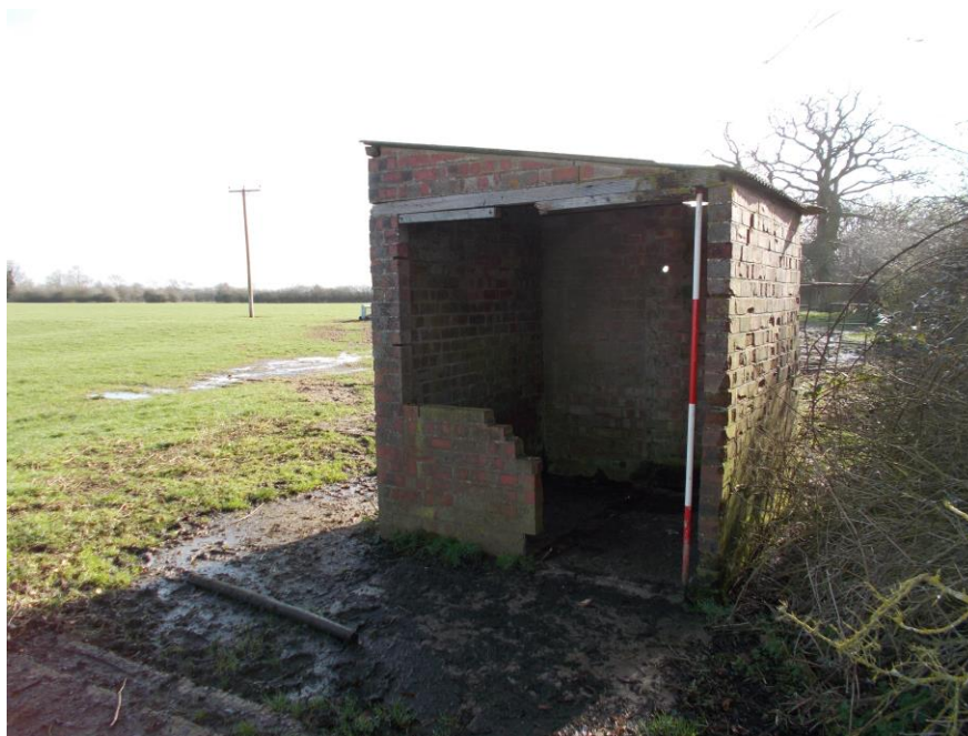
Plate 24: View NE showing NW-facing elevation of Building G, with concrete plinth for prefabricated hut in background to rear
