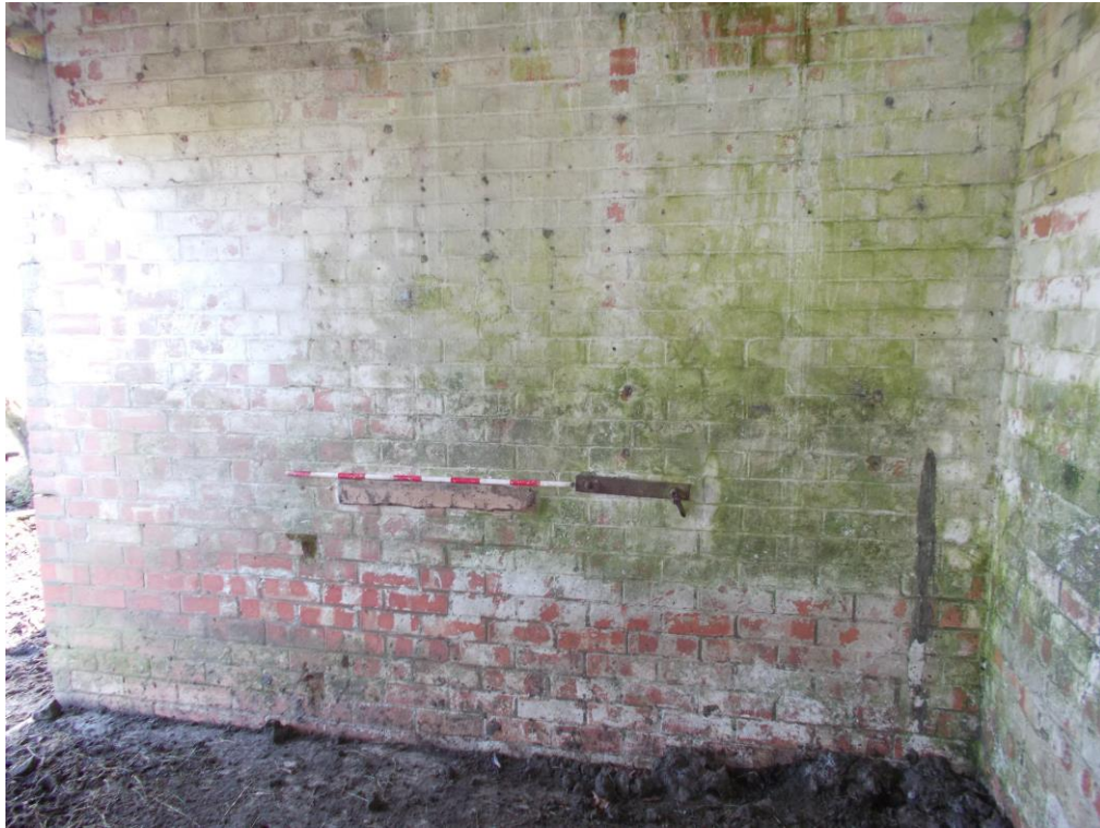
Plate 12: Internal view looking SE showing whitewashed wall with iron wall tie within NW compartment of Building A
