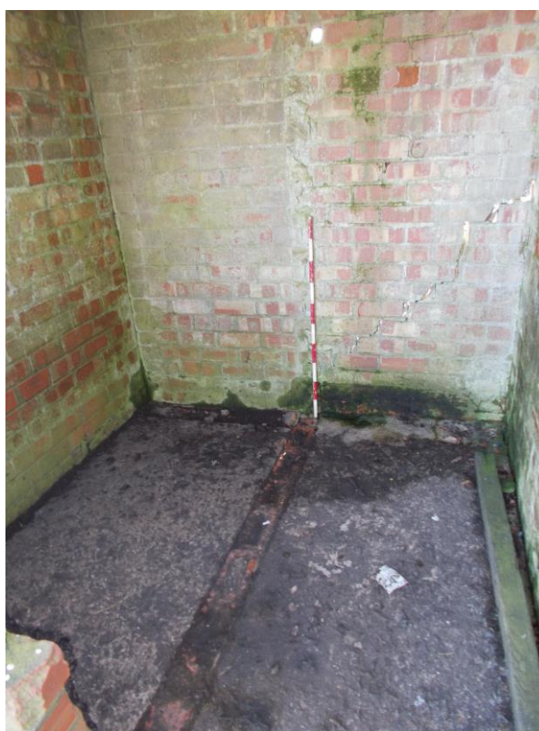
Plate 25: Internal view looking SE showing interior of Building G with evidence of brick partition
