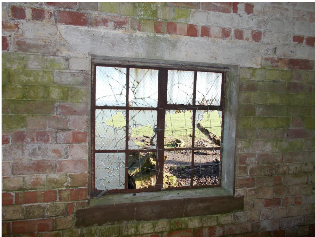
Plate 11: Detail showing 12-paned casement window with reinforced frosted glass within SE compartment of Building A
