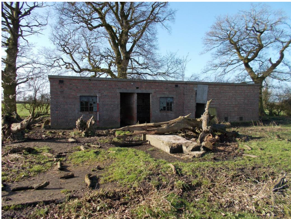
Plate 19: View SW showing foundation plinth for Building D in foreground with concrete base visible to right of picture
