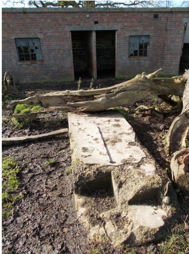
Plate 18: View looking SW showing detail of concrete machine base in Building D
