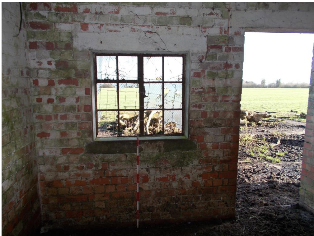
Plate 13: Internal view looking NE showing 12-paned casement window in NW compartment of Building A
