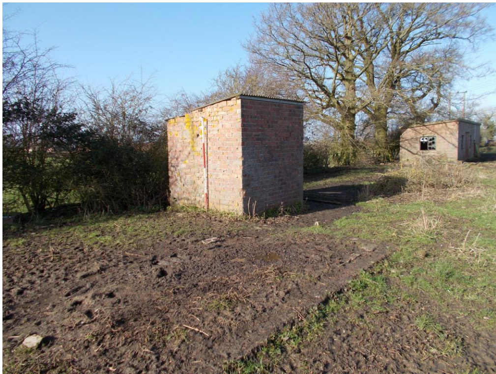
Plate 26: View WSW showing SE-facing elevation of Building G and a concrete foundation plinth for a prefabricated hut to the SE
