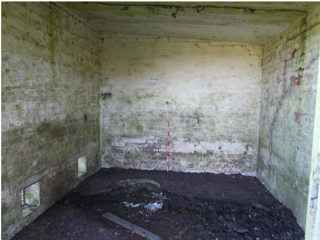
Plate 16: View looking SE showing whitewashed interior of large compartment at NW end of Building B with ventilation slots visible to left of picture
