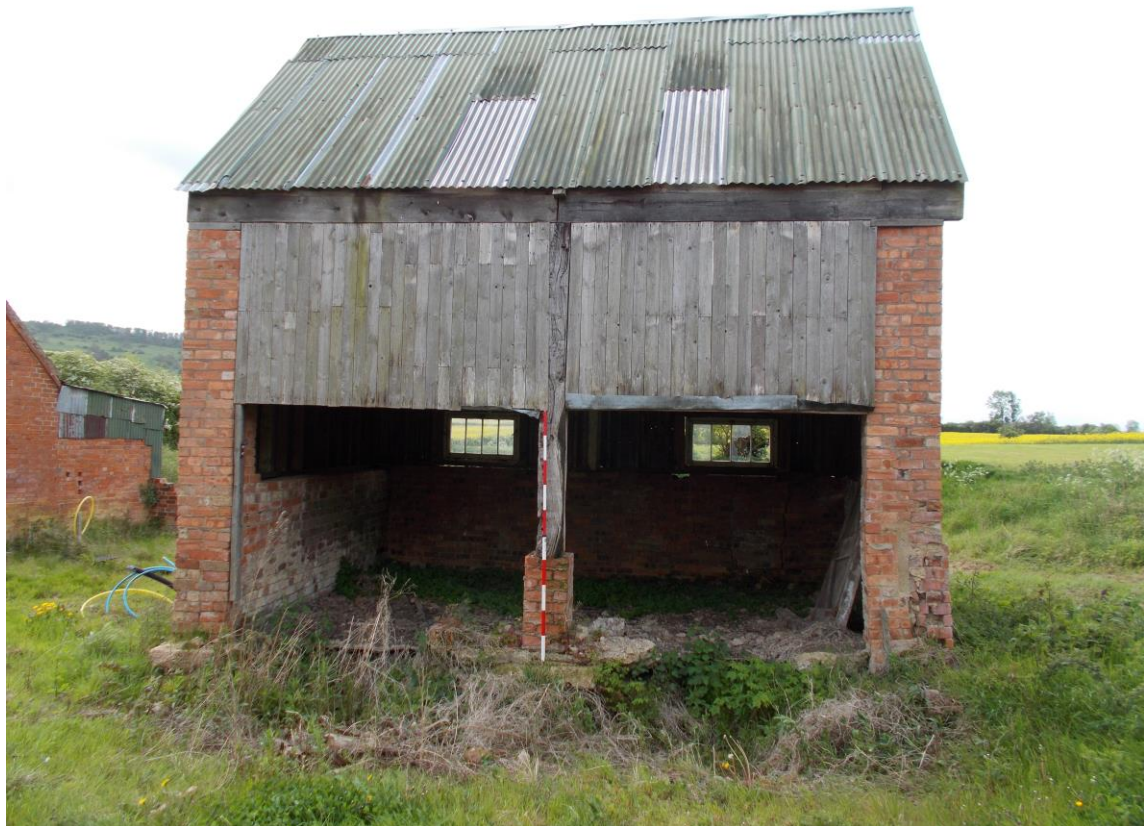
Plate 15: View looking south showing north-facing elevation of Building B with weatherboarded upper storey
