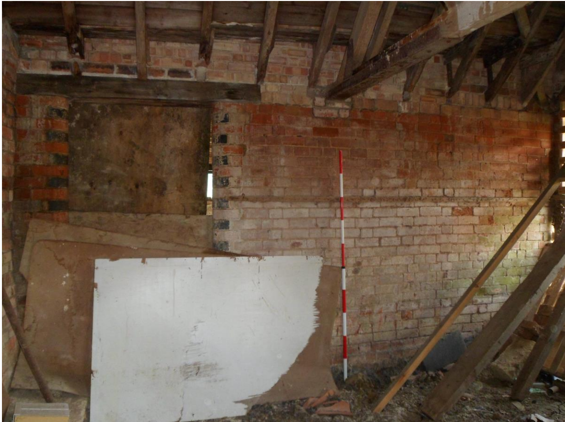
Plate 21: Interior view of Building C looking west showing modern flat arched door opening leading to Building D
