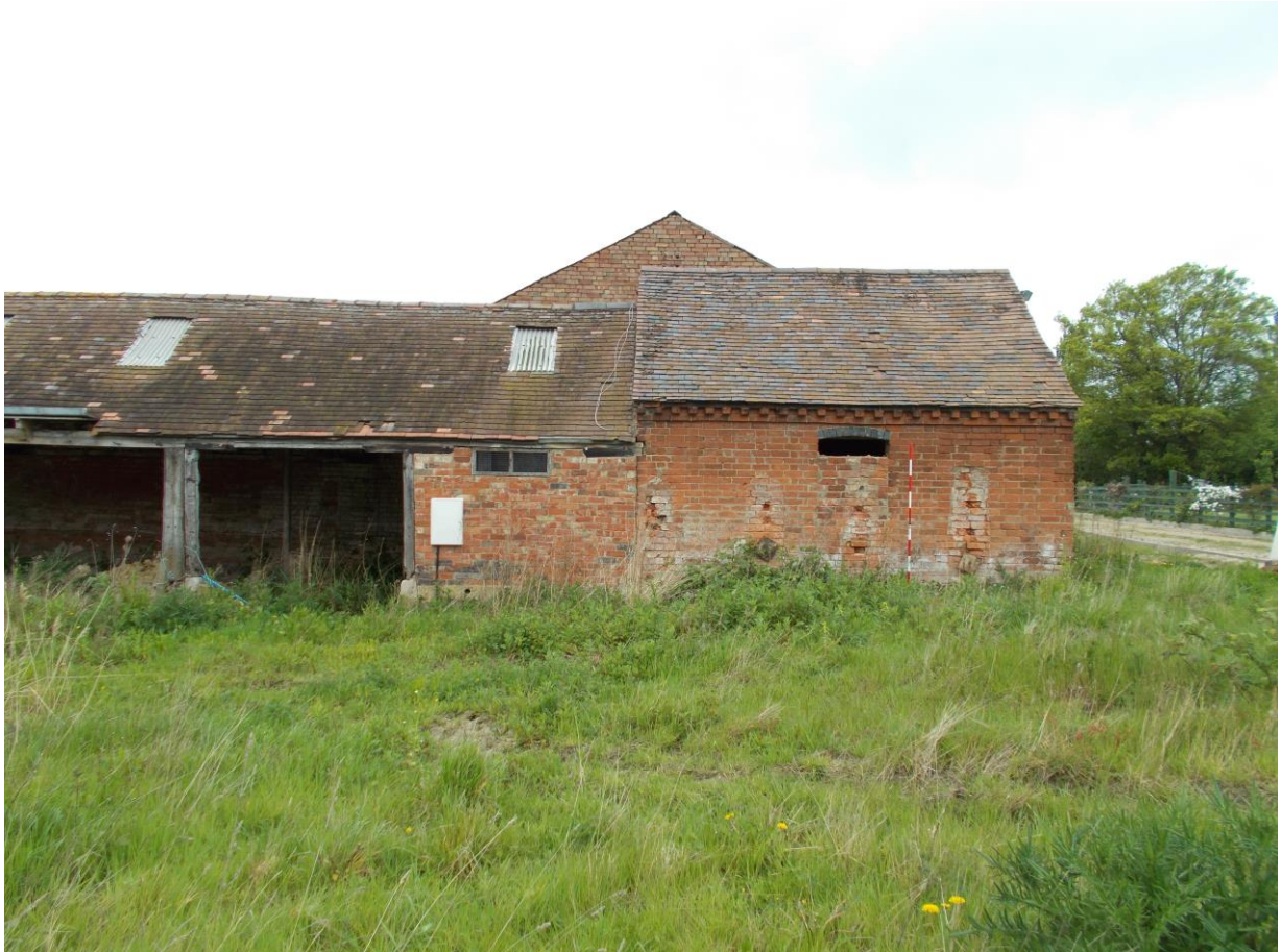
Plate 18: View looking west showing east-facing elevation of Building C with blocked up door opening in centre of elevation with an open fronted animal shelter to south (the northernmost bay having been blocked in at a later date)
