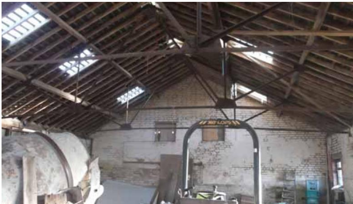
Plate 25: Interior view of Building D showing details of roof construction with timber roof supported by steel trusses
