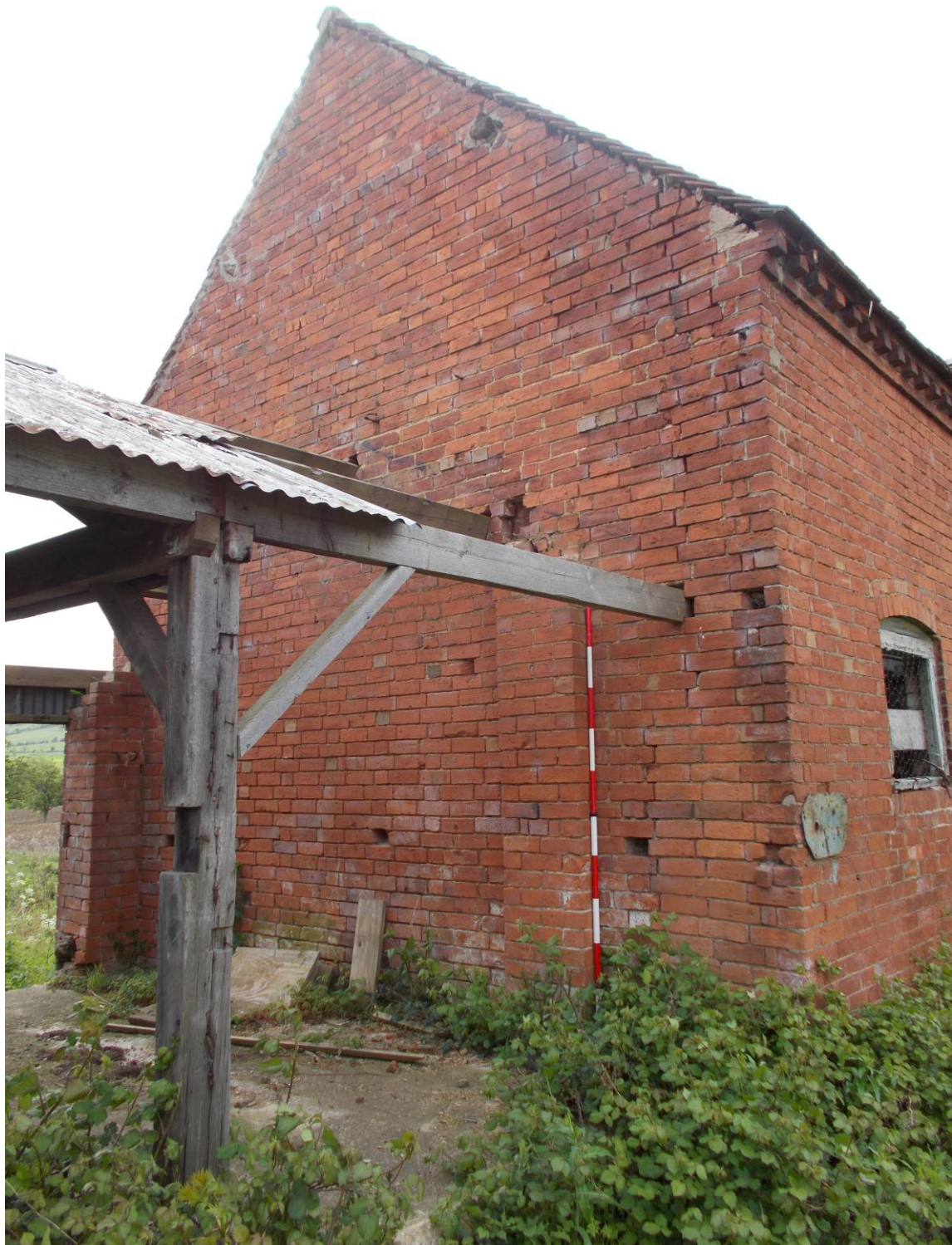
Plate 5: View looking southeast showing north-facing gable end of Building A with adjoining modern lean-to structure with corrugated metal roof
