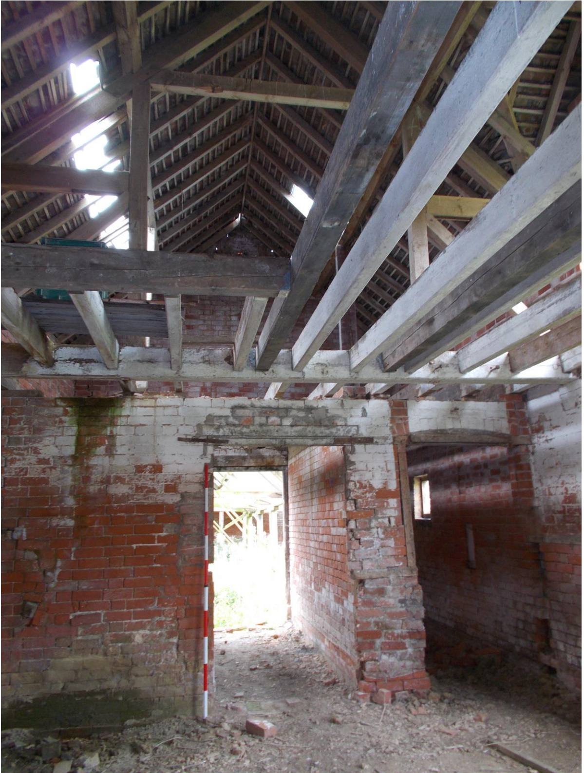
Plate 7: Interior view of Building A looking south showing detail of open truss roof structure and internal partition walls
