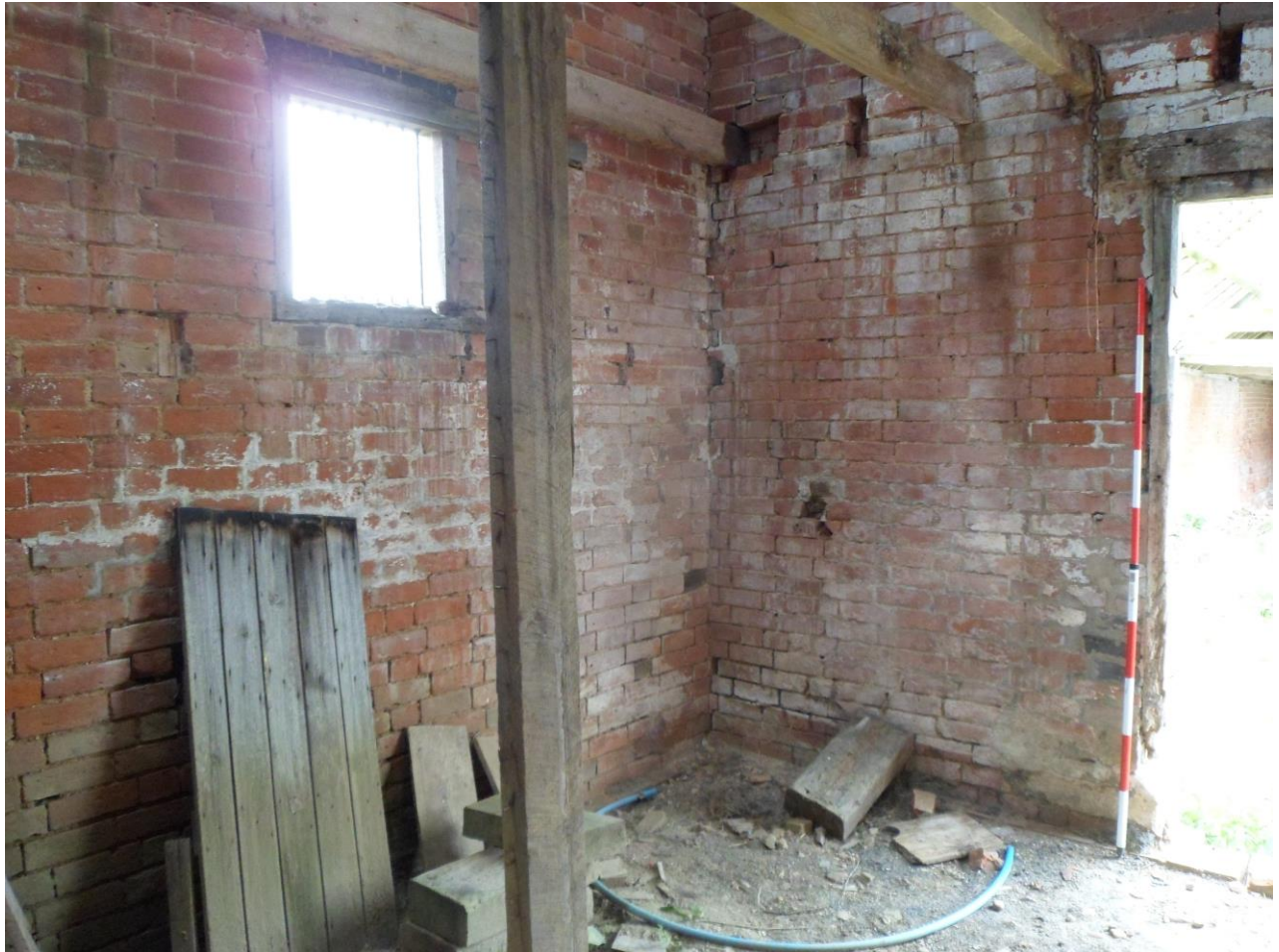
Plate 10: Interior view looking southwest showing the larger of the two compartments in the southern part of Building A
