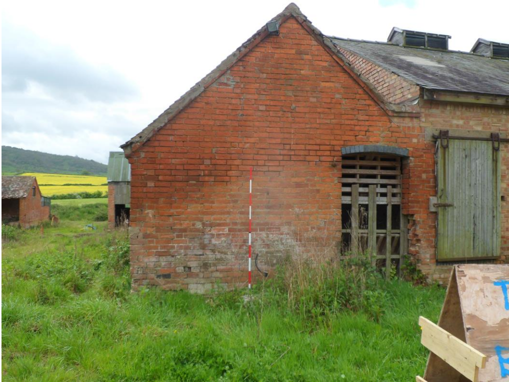
Plate 19: View looking south showing north-facing gable end of Building C with later doorway inserted (to right of picture)
