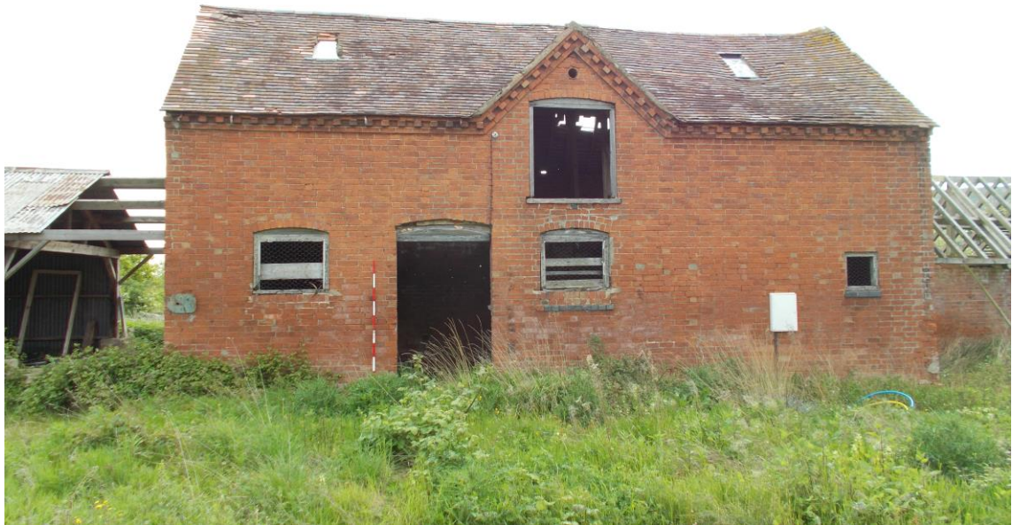
Plate 1: View looking east showing west-facing elevation of two storey gabled main block (Building A), with central loading bay and dentilled eaves cornice
