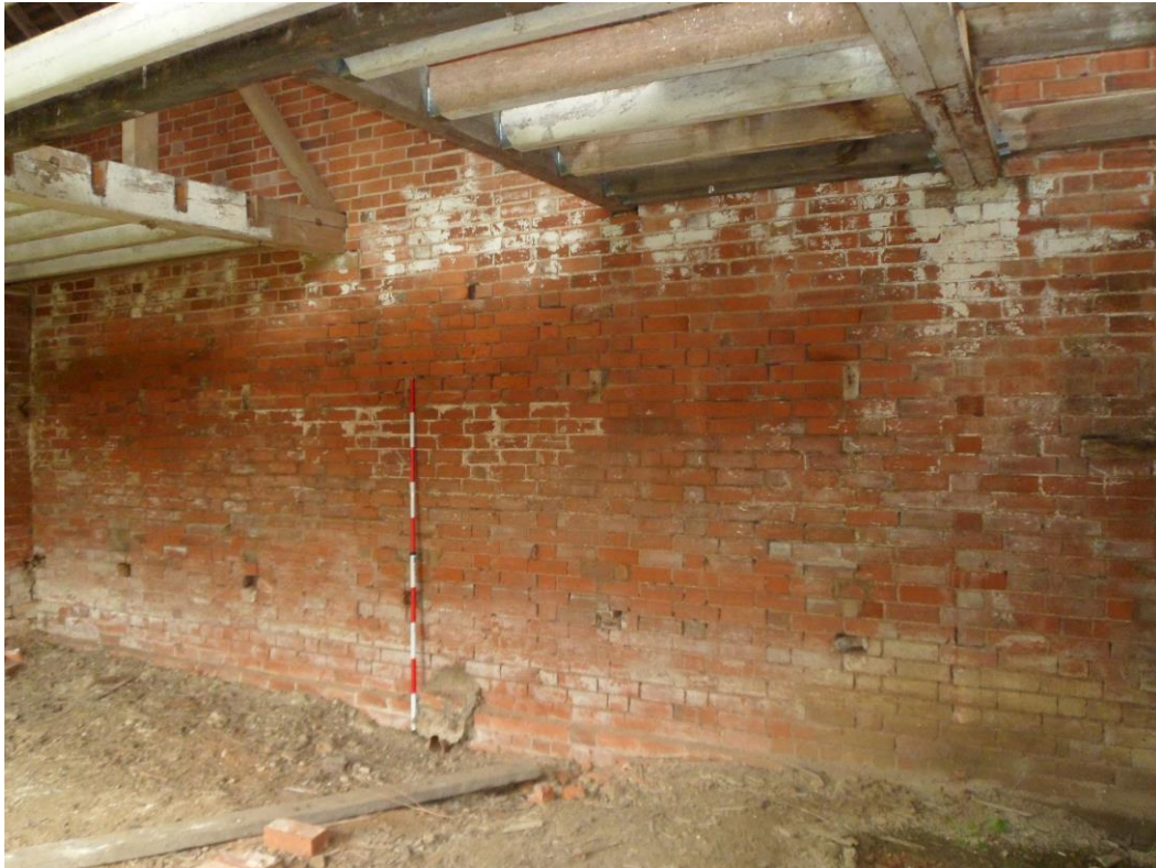
Plate 8: Interior view looking northeast showing west-facing internal elevation of barn with two horizontal rows of slots (some with timber stubs) for wooden racks or mangers
