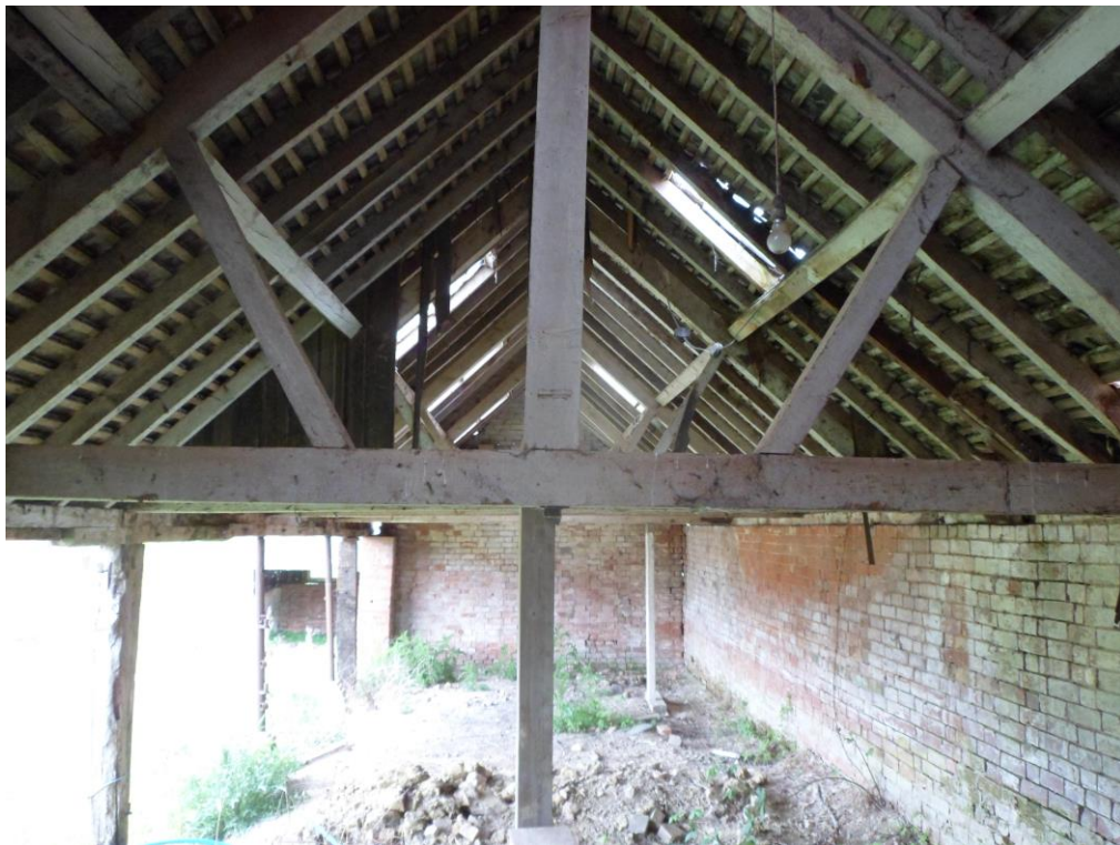
Plate 20: View looking south showing kingpost roof construction of animal shelter attached to Building C
