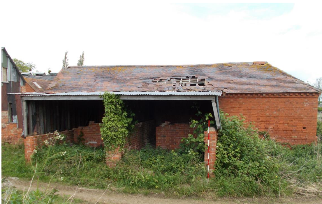
Plate 14: View looking north showing brick pigstys attached to south elevation of L-shaped range (Building A)
