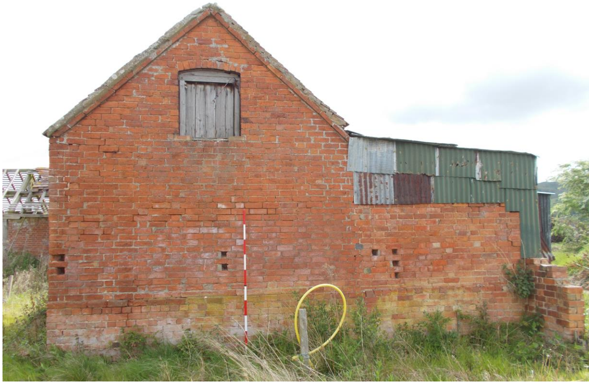
Plate 13: View looking east showing west-facing gable end of L-shaped range (Building A) with segmental arched window opening in upper storey and later brick pigstys to right of picture
