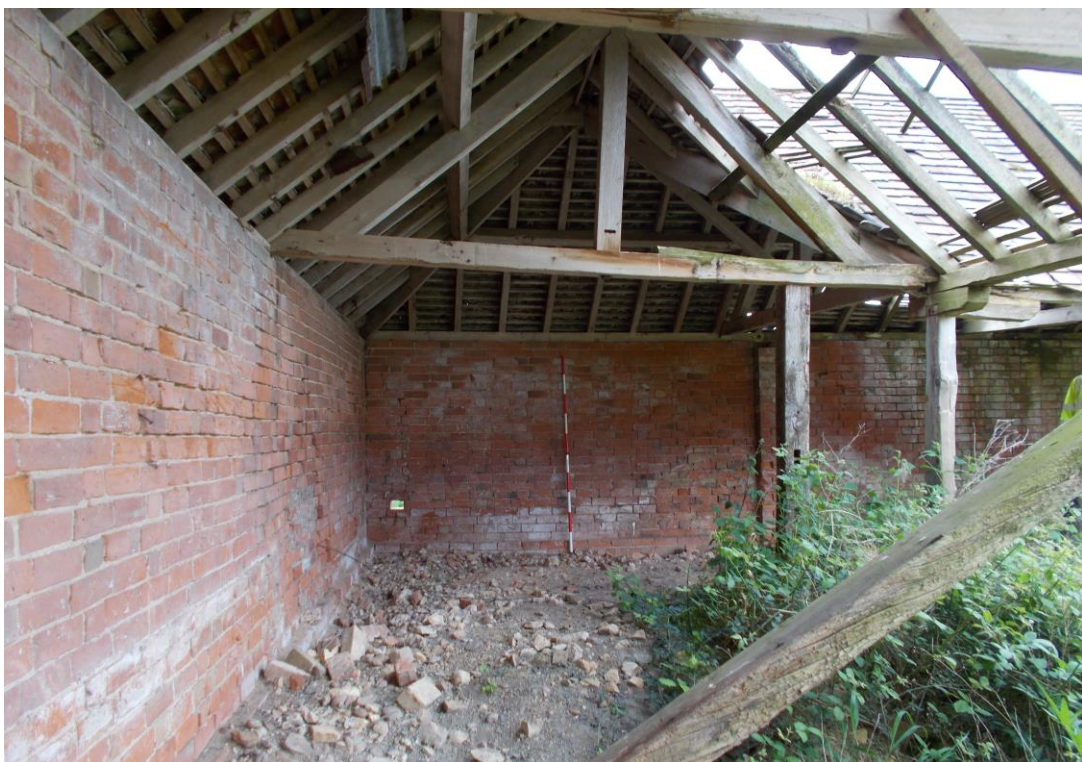
Plate 12: View looking south along southern arm of open fronted animal shelter adjoining Building A showing post and truss roof construction
