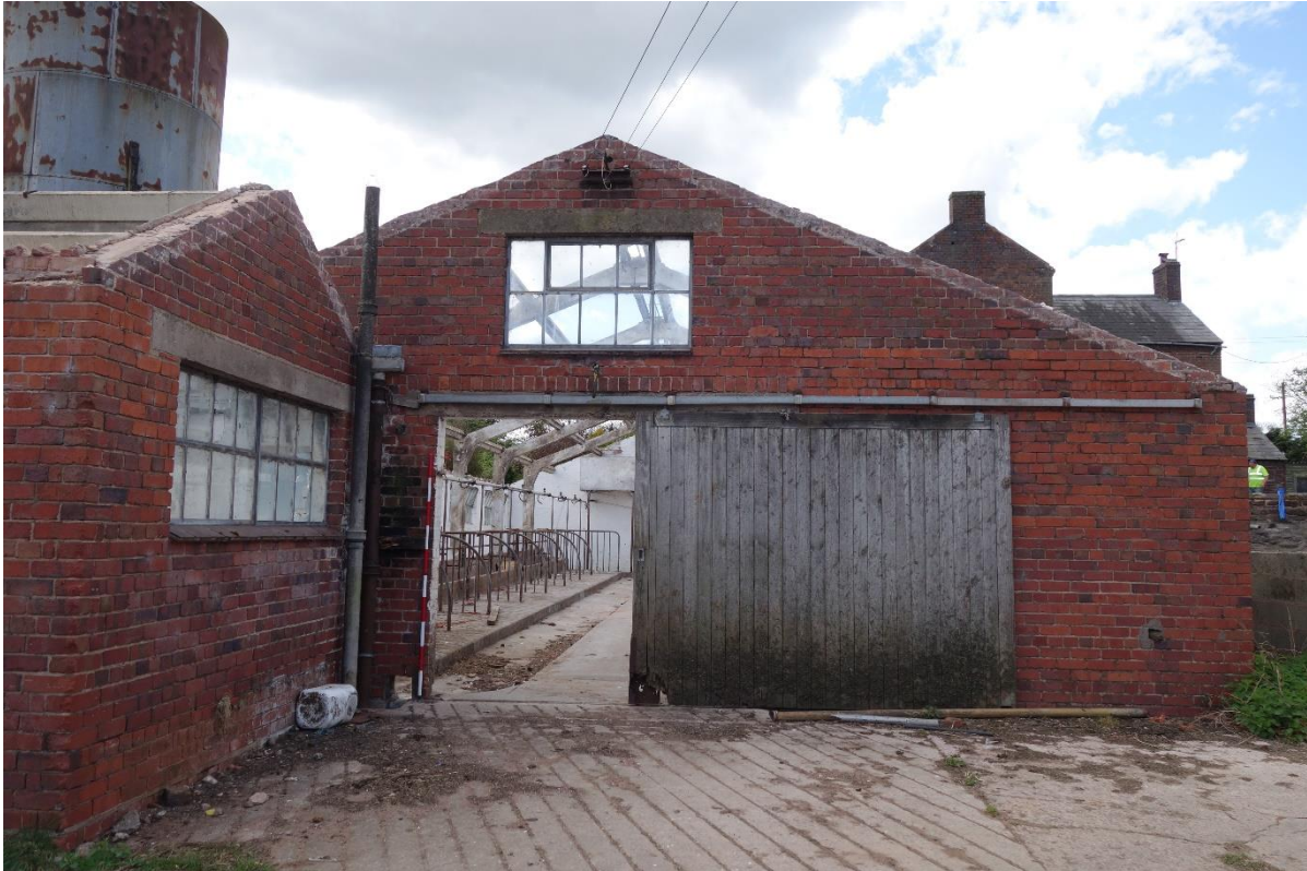
Plate 26: View looking SW showing NE -facing elevation of milking parlour (Building D), with adjoining block to left of picture
