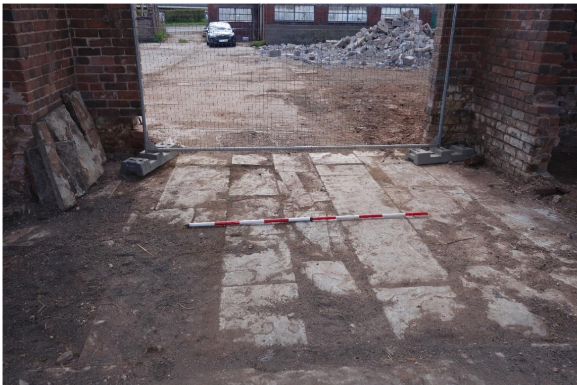
Plate 5: Internal view looking SE showing the partially intact stone flagged threshing floor at the NE end of Building A
