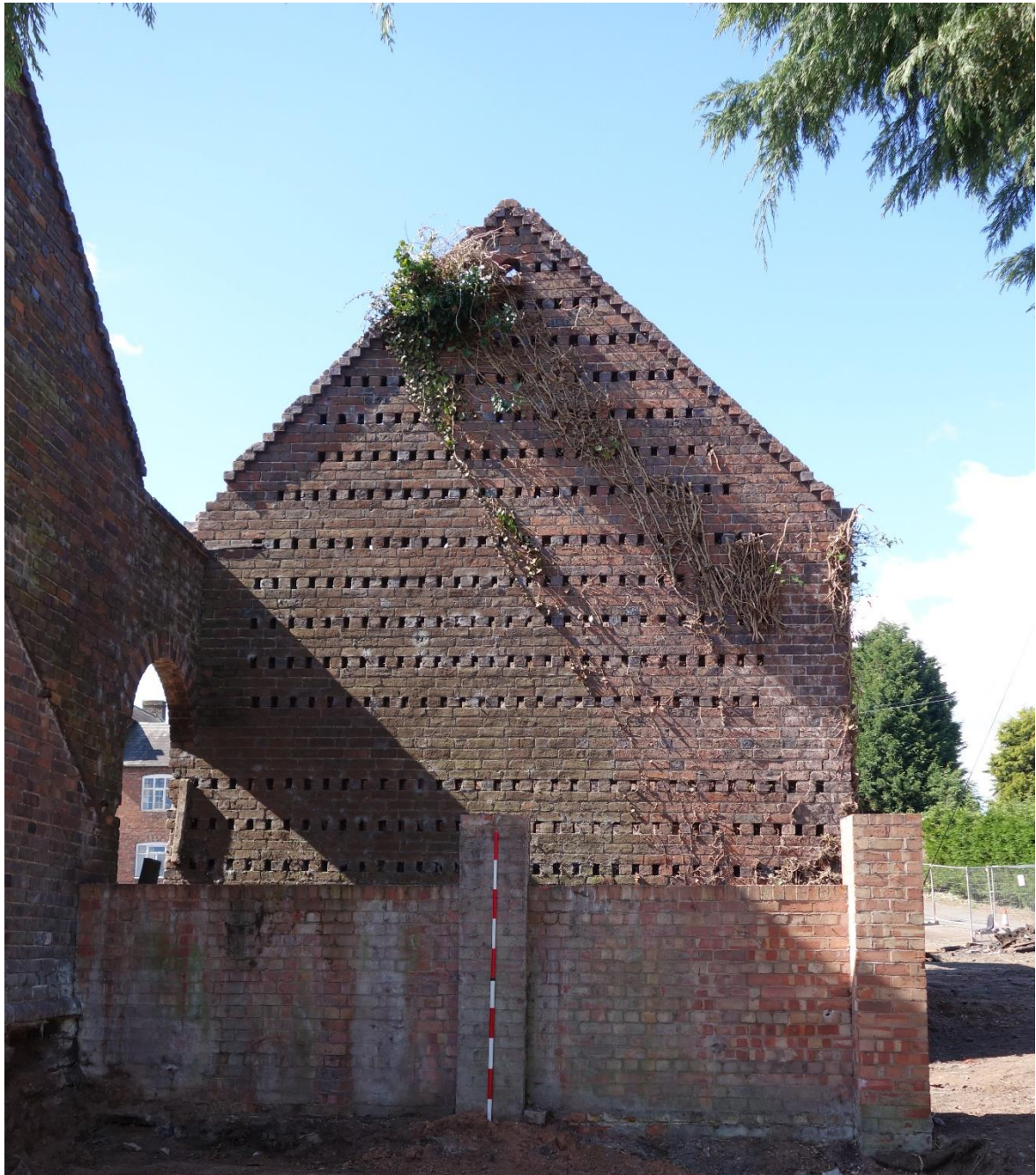
Plate 3: View showing the NE gable end of the threshing barn (Building A) with ventilation slots extending up to the apex of the gable, to the left of which is a section of wall with a round-headed door opening connecting Buildings A & B
