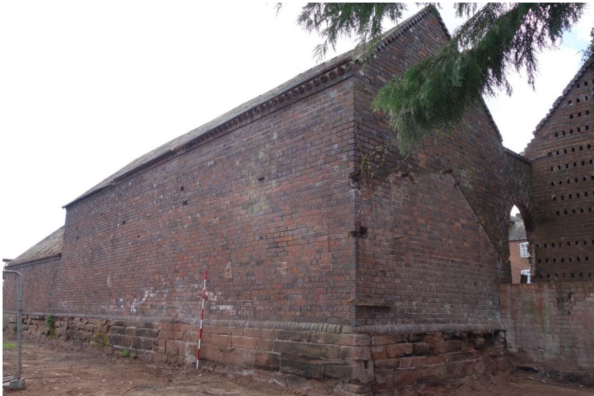
Plate 12: View looking S showing the NE walls and NW-facing gable end of stable block (Building B) resting on a roughly coursed masonry plinth, with evidence for demolished structures adjoining both elevations
