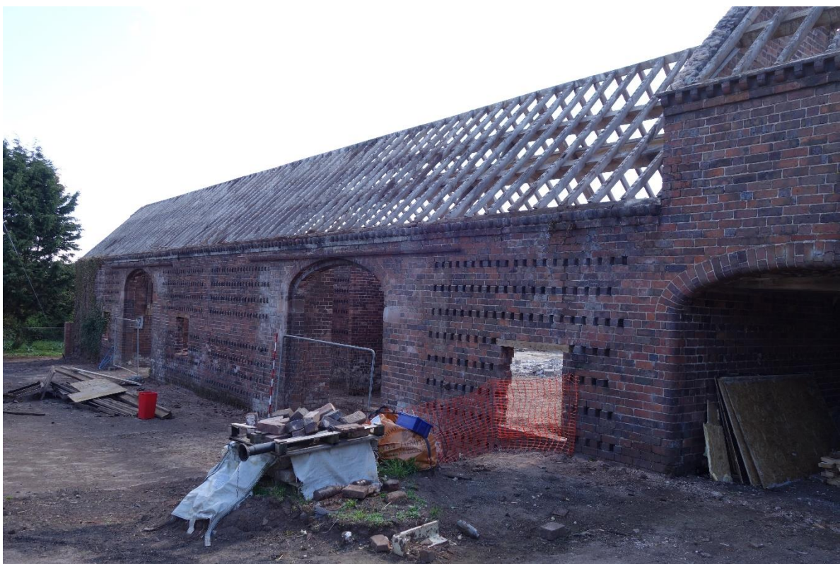
Plate 2: View looking ENE showing NW-facing elevation of Building A, with the granary and cartshed to right of picture
