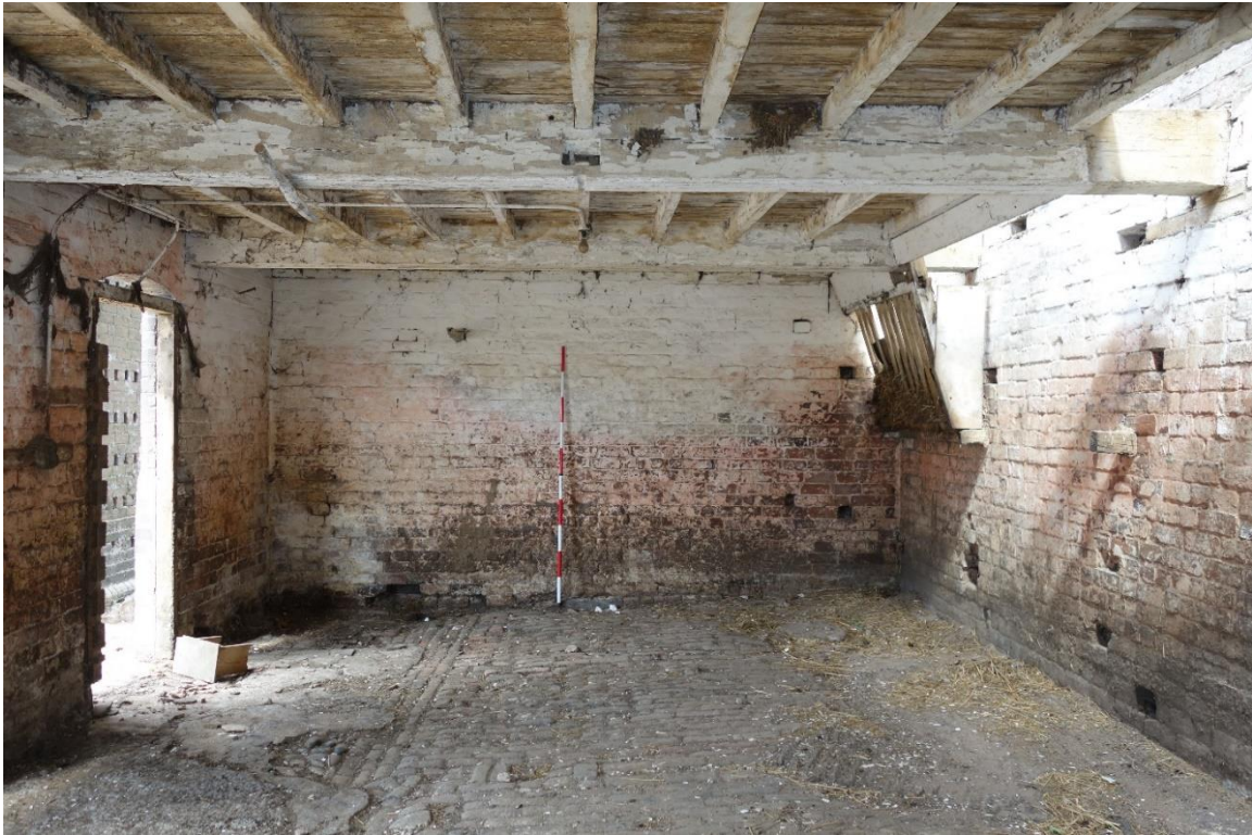
Plate 17: Internal view looking NW showing interior of four-bay stable block (Building B) with cobbled flooring and intact hayrack in NE corner
