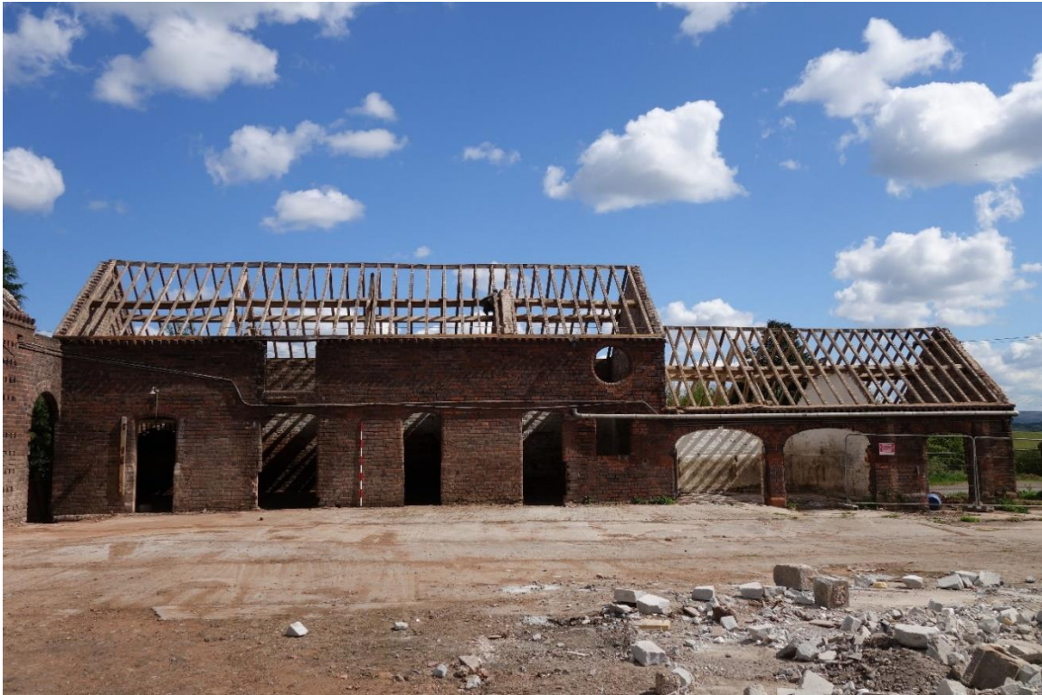
Plate 13: View looking NE showing the principal SW -facing elevation of Building B, showing the four-bay stable block with adjoining three-bay annexe, probably used as a cartshed
