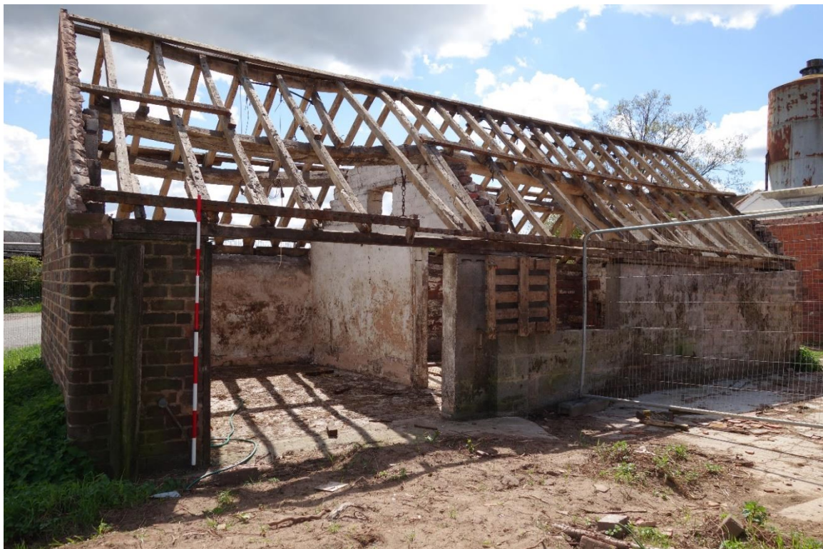
Plate 24: View looking S showing NW-facing elevation of Building C, heavily rebuilt with concrete breezeblocks, and the NE-facing elevation rebuilt in brick
