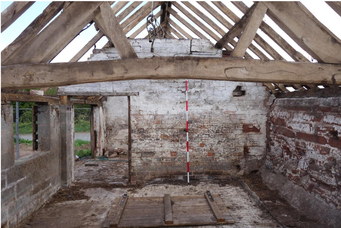
Plate 25: Internal view looking SE showing interior of compartment within Building C showing open-truss roof structure with angled struts connecting the tie-beam to the principal rafters
