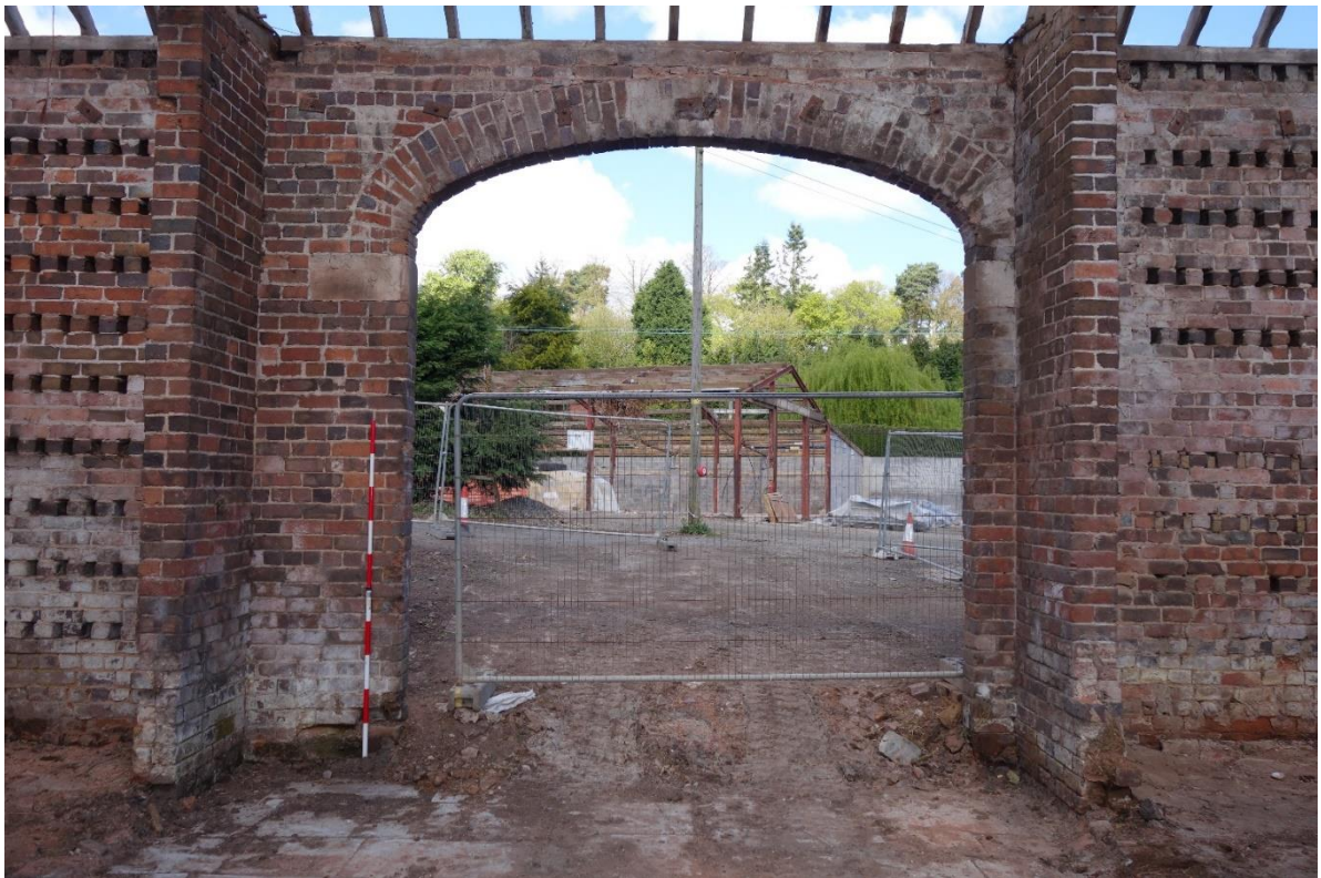
Plate 4: Internal view looking NW showing the wagon arch towards the NE end of Building A, with the threshing floor in background, partially truncated by a modern concrete ramp
