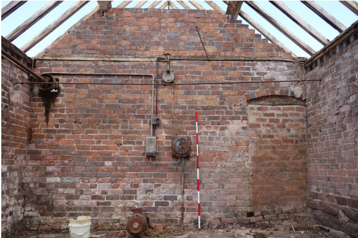
Plate 20: Internal view looking NW showing partition wall in smaller compartment at SE end of Building B, with blocked doorway to right of picture and generator in centre of picture
