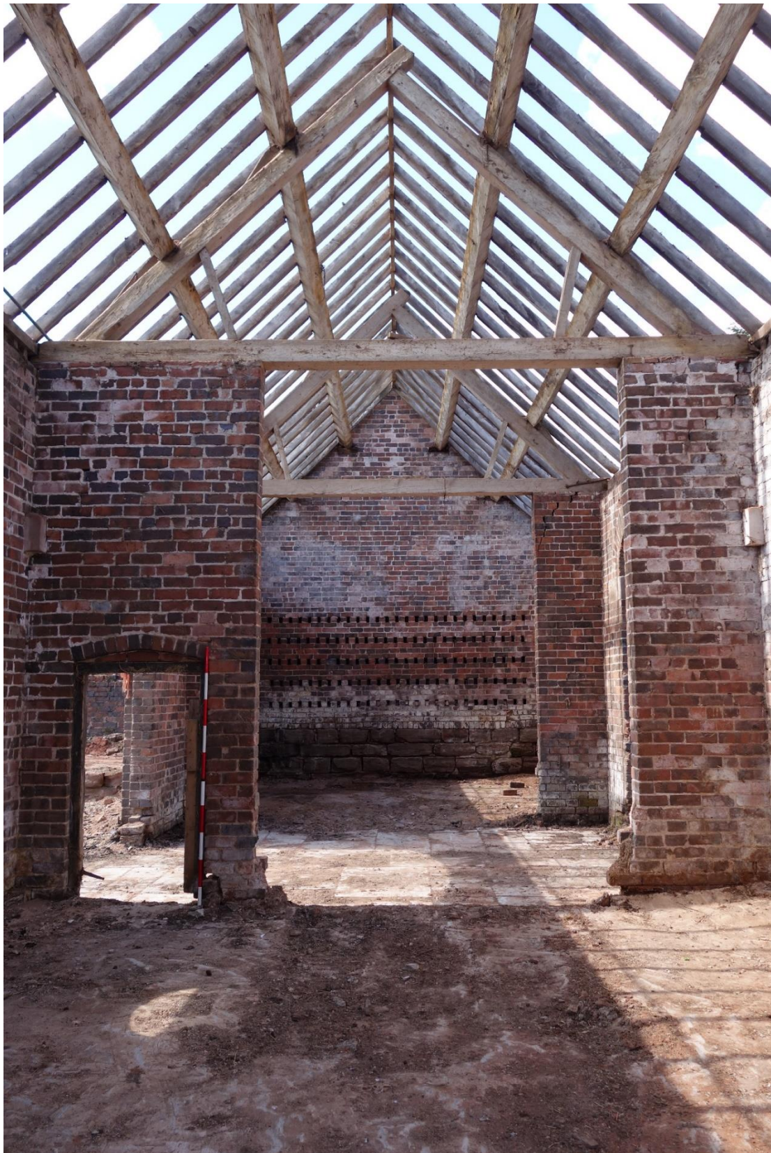
Plate 7: View looking SW showing SW end of threshing barn (Building A) with segmental-arched doorway inserted in buttress to left of picture, with evidence for a low brick partition wall indicated by heavily truncated wall stubs.
