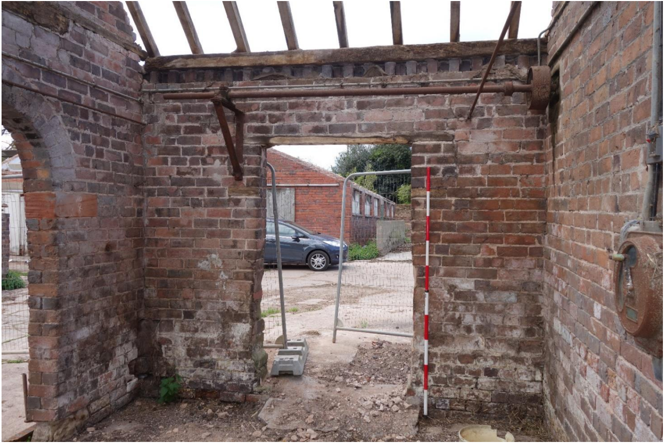
Plate 21: View looking SW showing cast iron overhead drive shaft and gear wheel above doorway in smaller compartment of Building B
