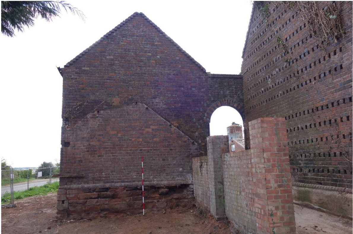
Plate 15: View looking SE showing NW gable end of stable block (Building B), with evidence of a gabled extension indicated by a pitched roofline and projecting brick wall stub
