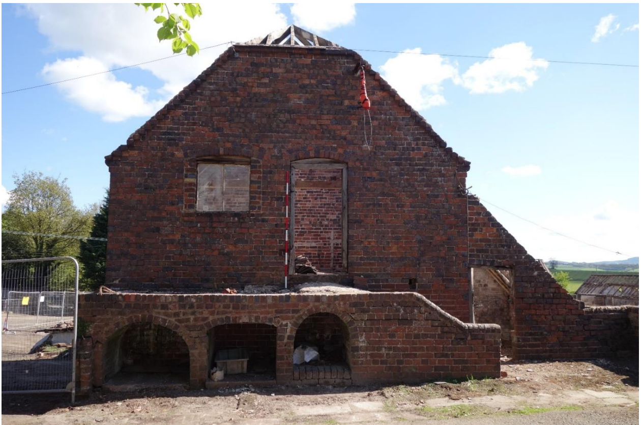
Plate 8: View looking NE showing SW-facing elevation of granary with arched recesses in stairs and lean-to piggery building to right of picture
