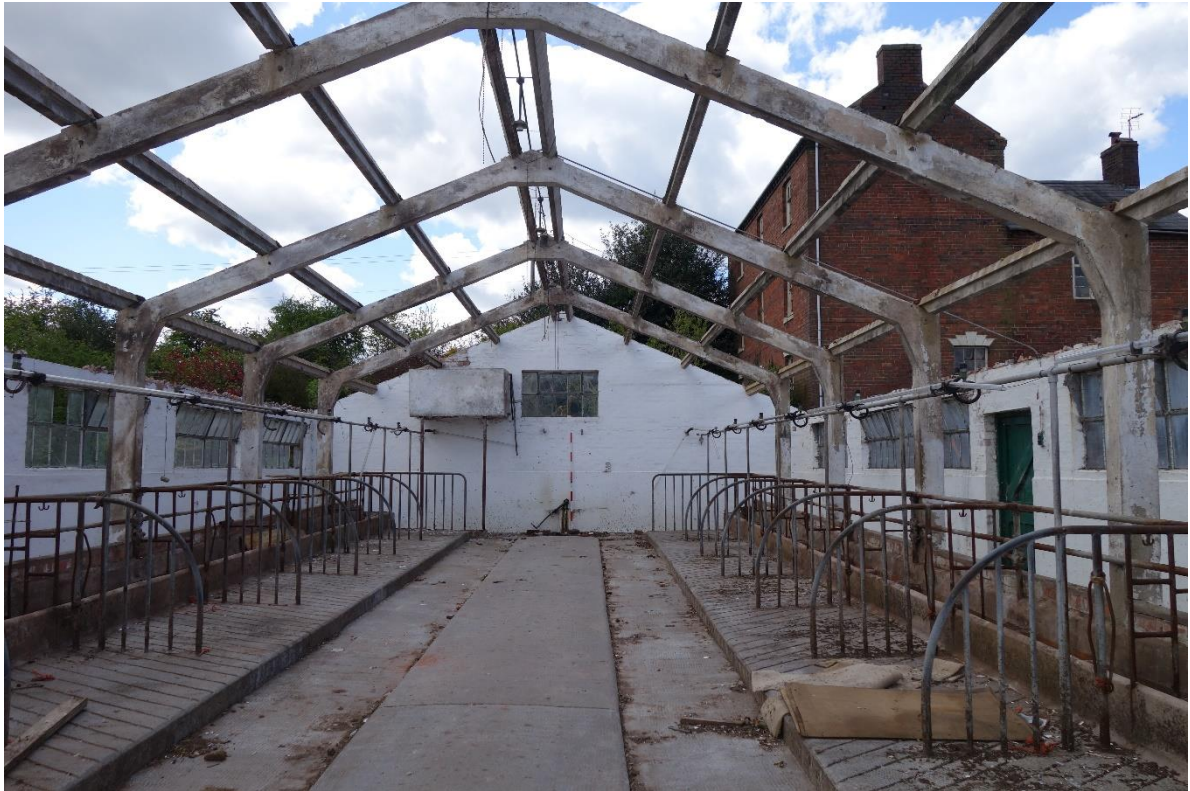
Plate 28: View looking SW showing interior of milking parlour (Building D) with steel roof trusses
