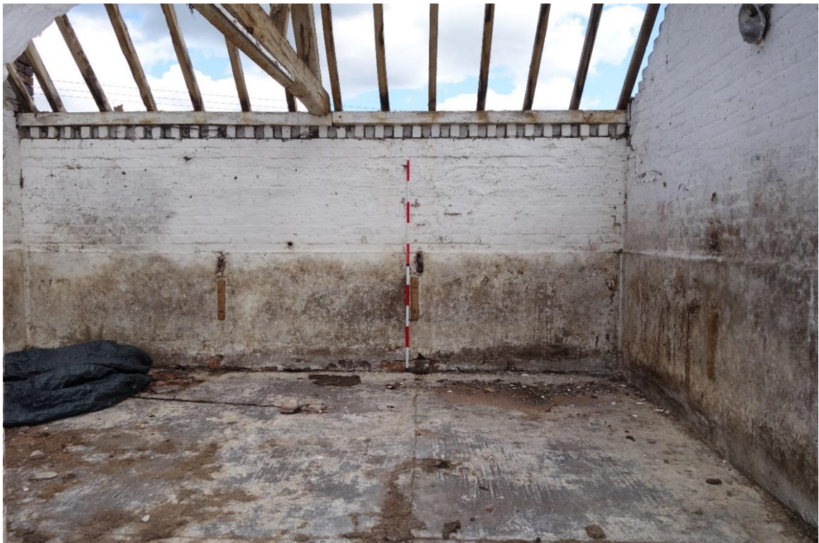
Plate 19: Internal view looking NE showing interior of two-bay compartment (Building B) with later concrete flooring
