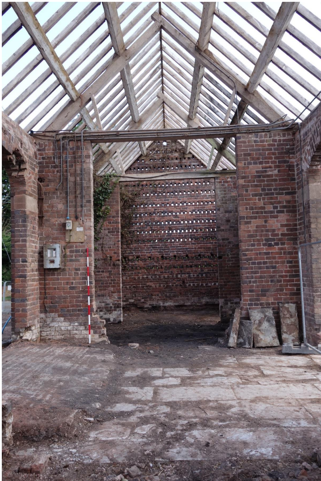
Plate 6: Internal view looking NE showing NE part of Building A with open-truss roof structure, the stone-flagged threshing floor in the foreground and beam slots for loft in NE gable wall
