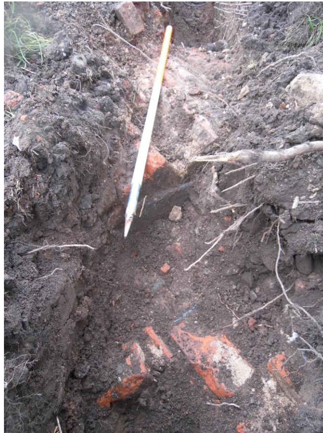
Plate 3: View N of culvert (513) showing stone slab blocking close to scale and loose bricks in foreground
