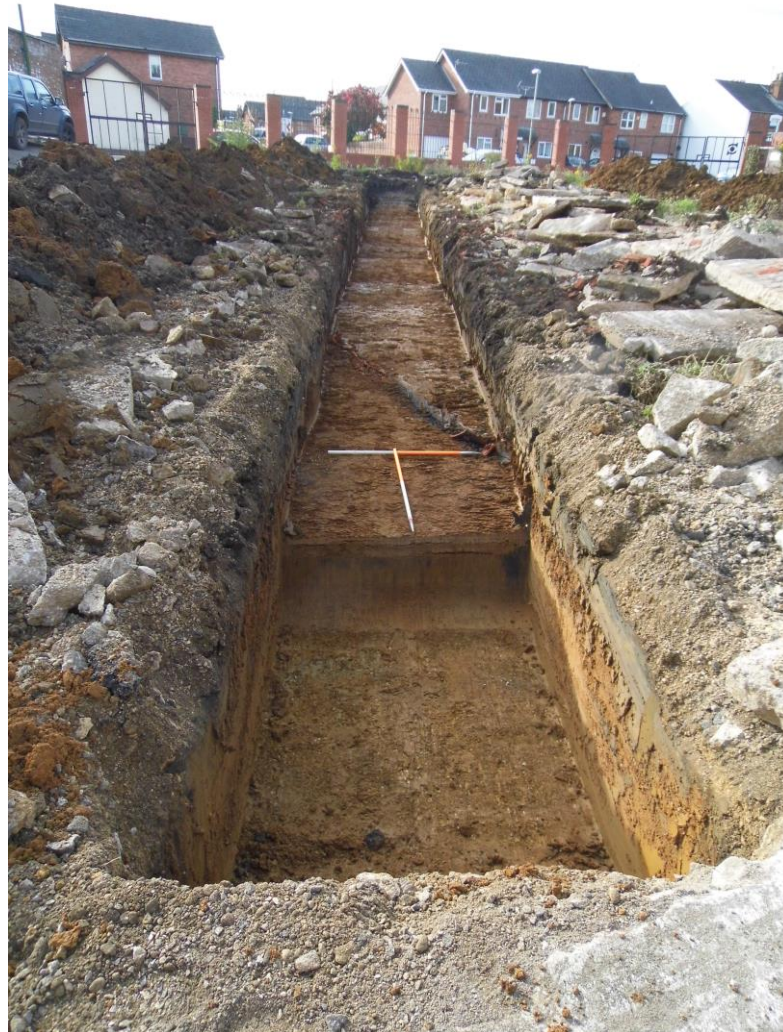
Plate 2: View SW of Trench 2 showing modern storm drain and sondage into natural clay
