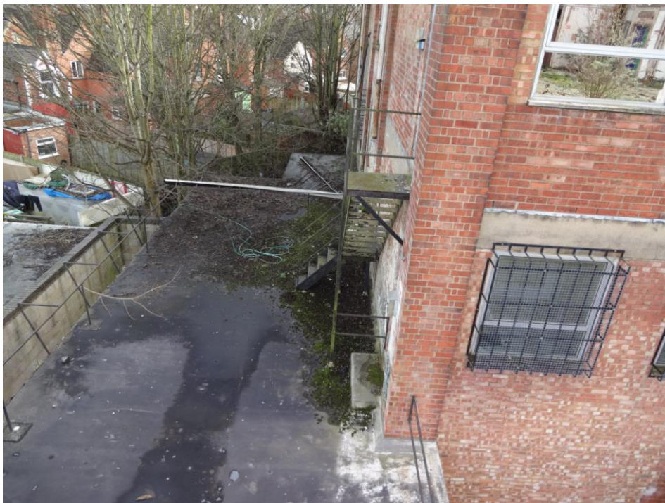
Plate 13: View SE of NE elevation Building 1 showing metal fire escape descending onto flat roof of annex
