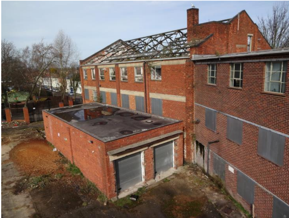
Plate 14: View N of SE elevation of Building 1 abutted and largely obscured by Building 2. Building 1a is situated to left
