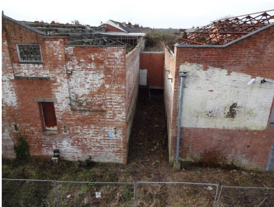
Plate 46: View W showing E elevations of Buildings 6 (right) and 7 (left) with connecting link block (centre). Note evidence of lean-to structure formerly attached to Building 6 and traces of whitewash adhering to the Building 7 elevation
