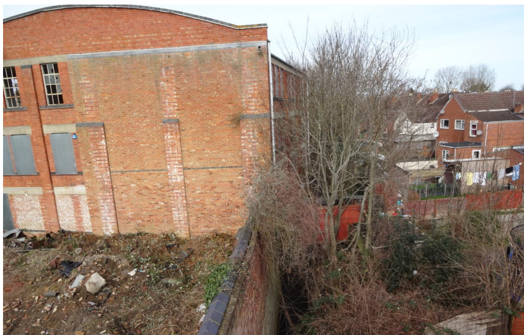
Plate 22: View NW showing S elevation of Building 3 and culverted watercourse (Sud Brook), with NE-facing elevation just visible adjacent to the watercourse and rear gardens of neighbouring properties. The photograph shows a thickening of the brickwork marking the point at which a former ironmonger's store built in 1909 abutted the elevation.
