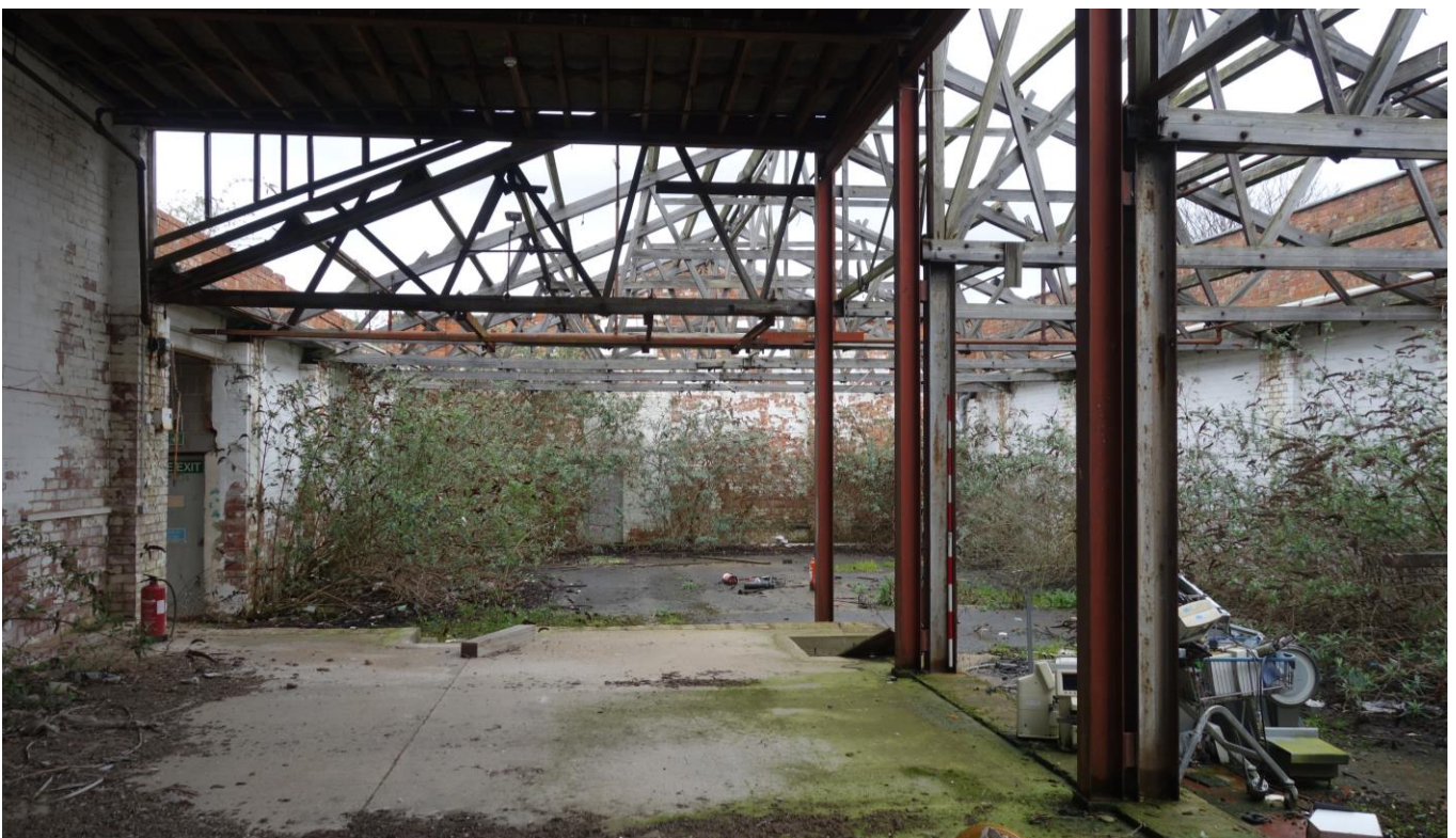
Plate 49: Interior of Building 7. View E from modern loading bay with original roof trusses to right and rear.
