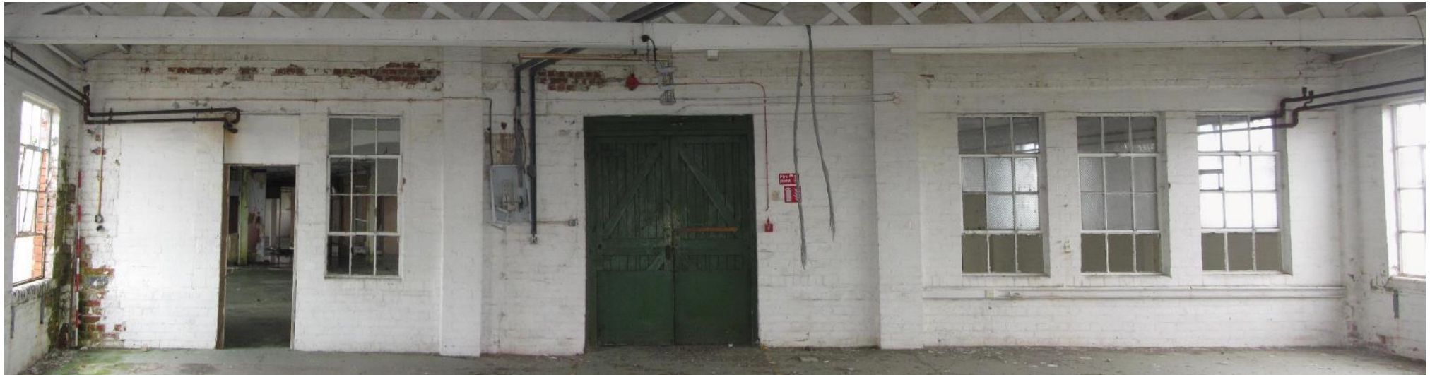
Plate 30: View of internal end wall elevation at upper storey level looking N through into Building 2
