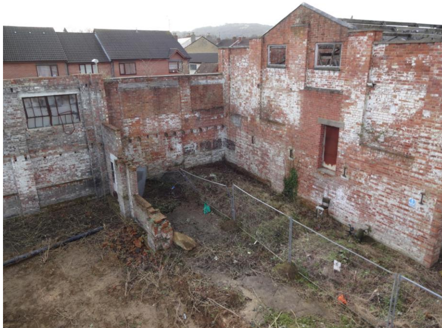
Plate 1: View SW showing Building 7 and other structural remains at the southern extent of site, with fire-damaged building to left
