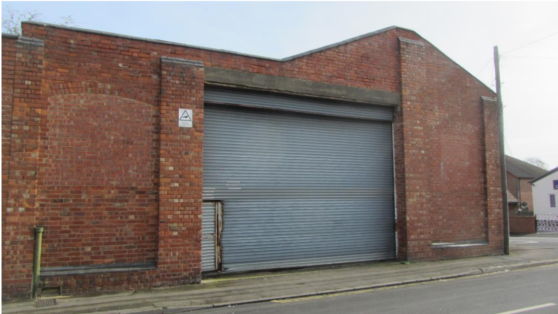
Plate 50: View ESE from Tarrington Road towards Hatherley Road showing existing west elevation of Buildings 6 & 7 with earlier openings to the left and right infilled with later brickwork.
