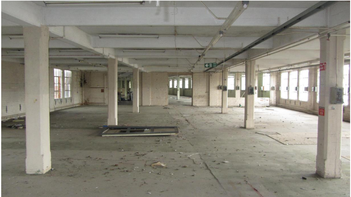
Plate 26: View NW of first floor Building 3 looking through into Building 2 and showing moulded pillars and reinforced concrete beams
