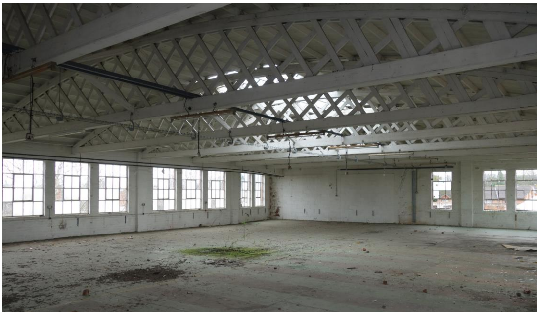
Plate 27: Internal view SE of upper storey of Building 3 showing lattice trusses supporting roof structure. Note: Open plan with no moulded beams.
