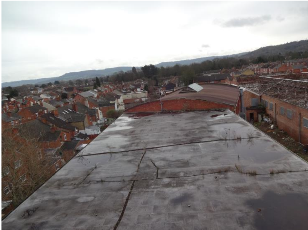
Plate 34: Detail of external roof structure showing flat roof of Building 2 (foreground) and curved profile of Building 3
