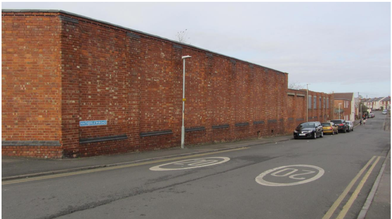
Plate 51: View along Hatherley Road showing present condition of S elevation of Building 7. Note blocked window openings
