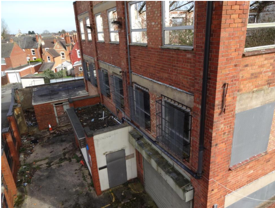
Plate 12: Building 1 view NNE of NW elevation showing modern annex at ground floor level
