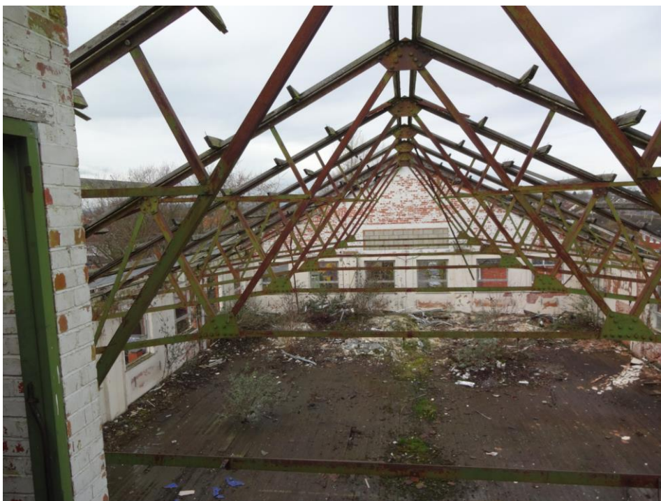
Plate 15: View NW of upper storey Building 1 showing double fink roof truss construction
