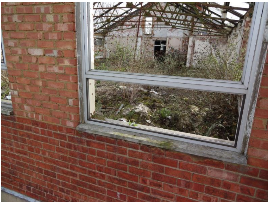
Plate 9: View through upper storey window of Building 1 showing internal floor space and gable end with access through to Building 2 with stairwell and elevator shaft to rear right. Note door threshold positioned at ceiling height.
