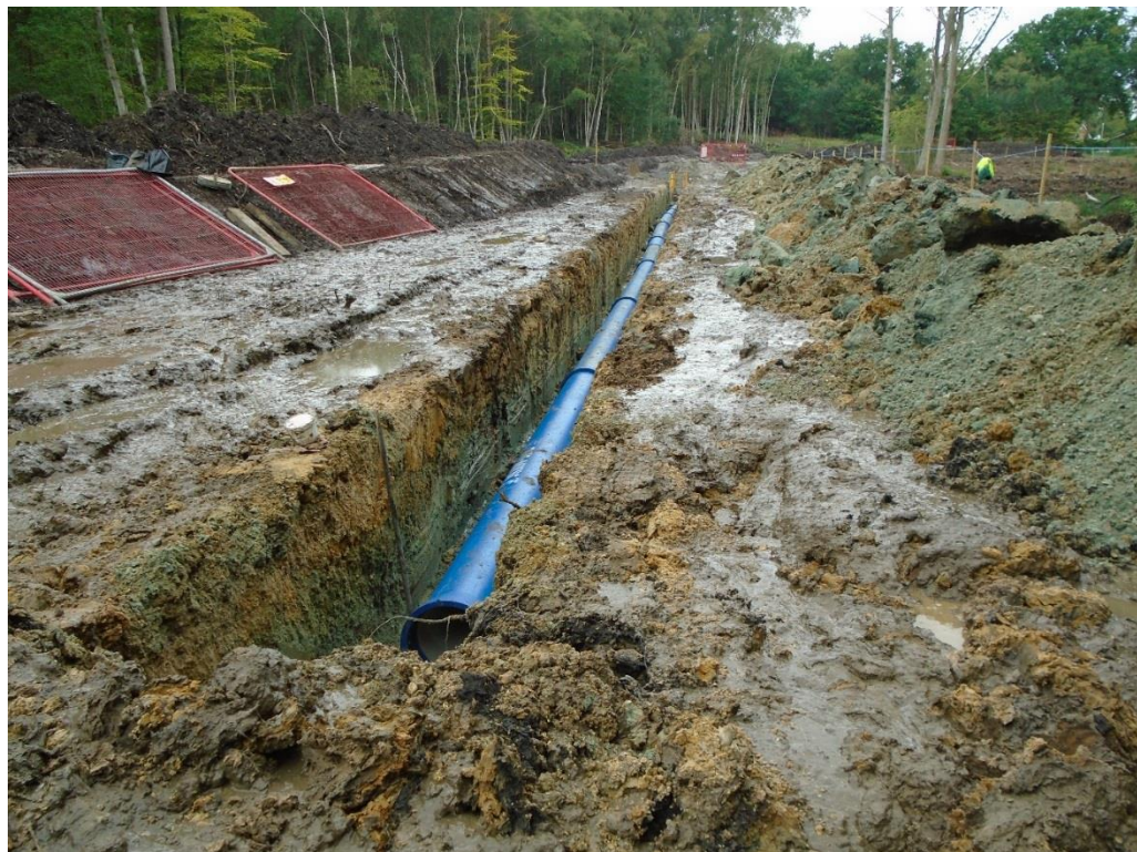
Plate 19: General view NW along pipe trench, looking towards the third bend of Section 3 of Route 3
