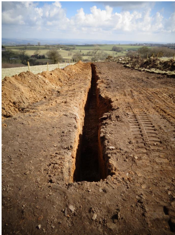
Plate 1: View NE (downslope) of trench and easement extending across pasture field adjacent to Mast Reservoir
