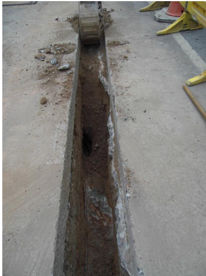
Plate 3: Concrete beneath existing road surface and bedrock in base of trench on Rainbow Hill; view SW
