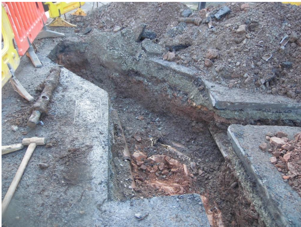
Plate 1: View NE at the junction of Lansdowne Crescent Lane and Lansdowne Walk showing existing ducts and natural bedrock
