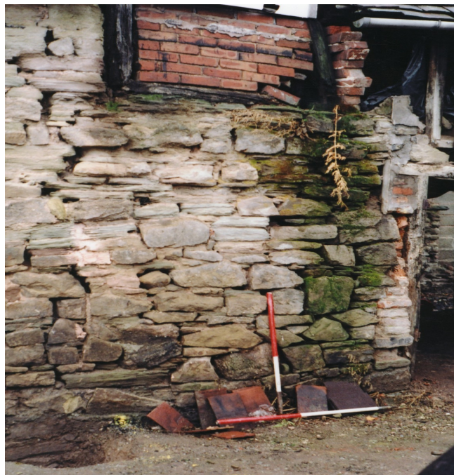
Fig. 4: W elevation showing collapse of dormer window
