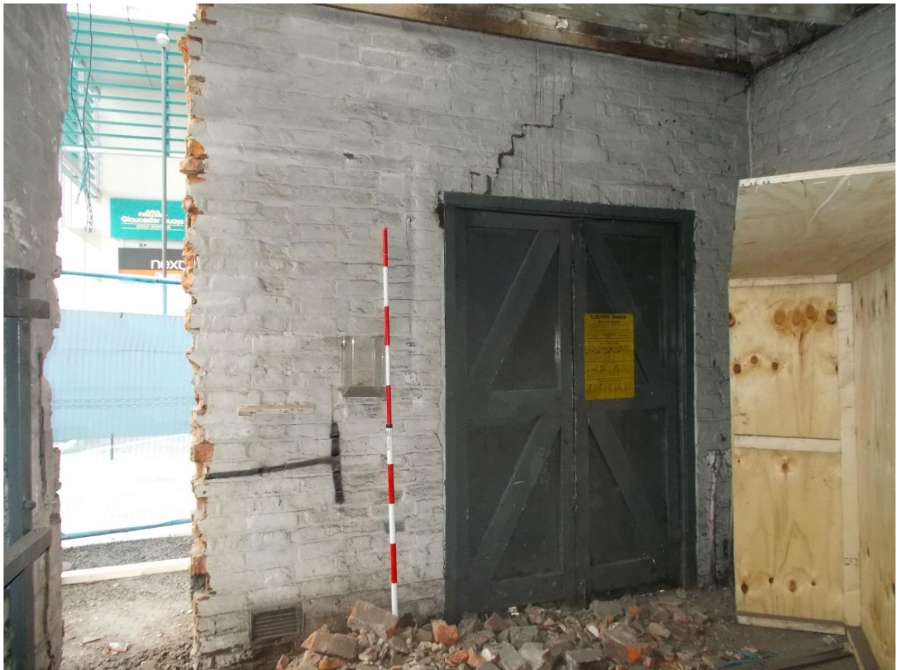
Plate 8: Internal view looking W showing flat headed doorway with pair of wooden double doors in W gable wall
