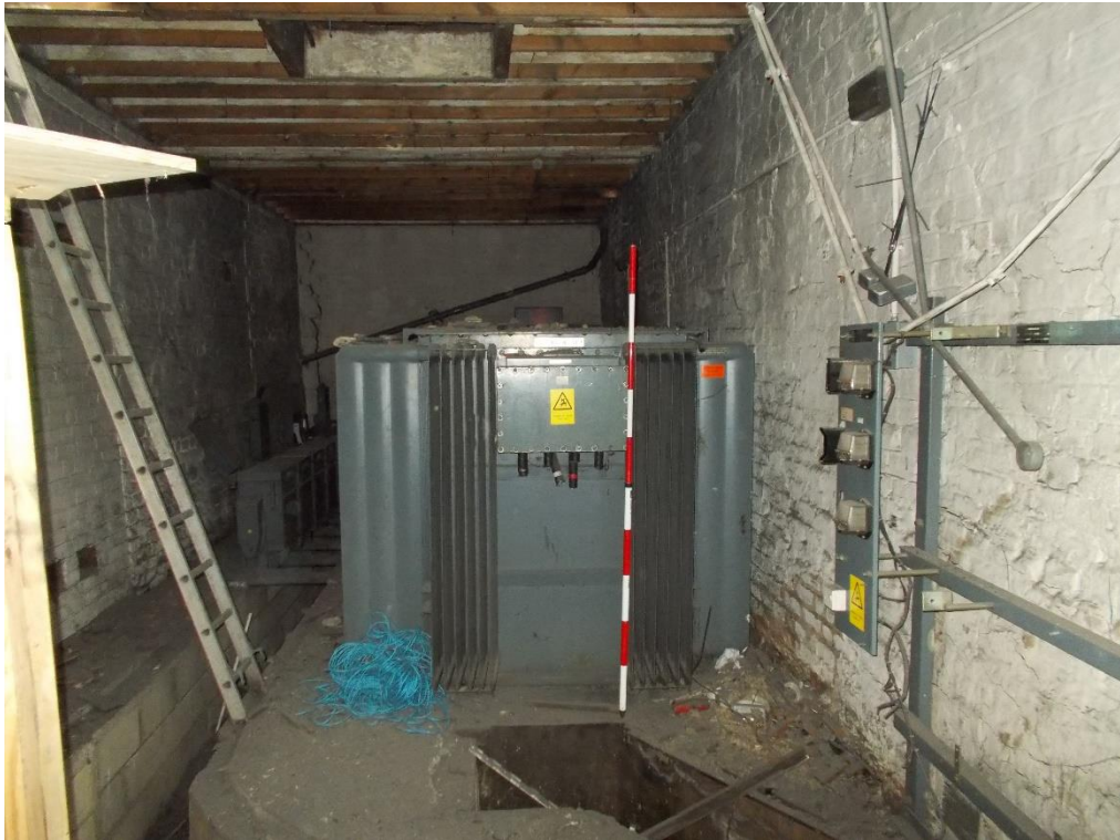
Plate 9: View looking E showing interior of Building A with raised concrete flooring with cable trenches leading to transformer. A hatch is visible in the ceiling just above the transformer
