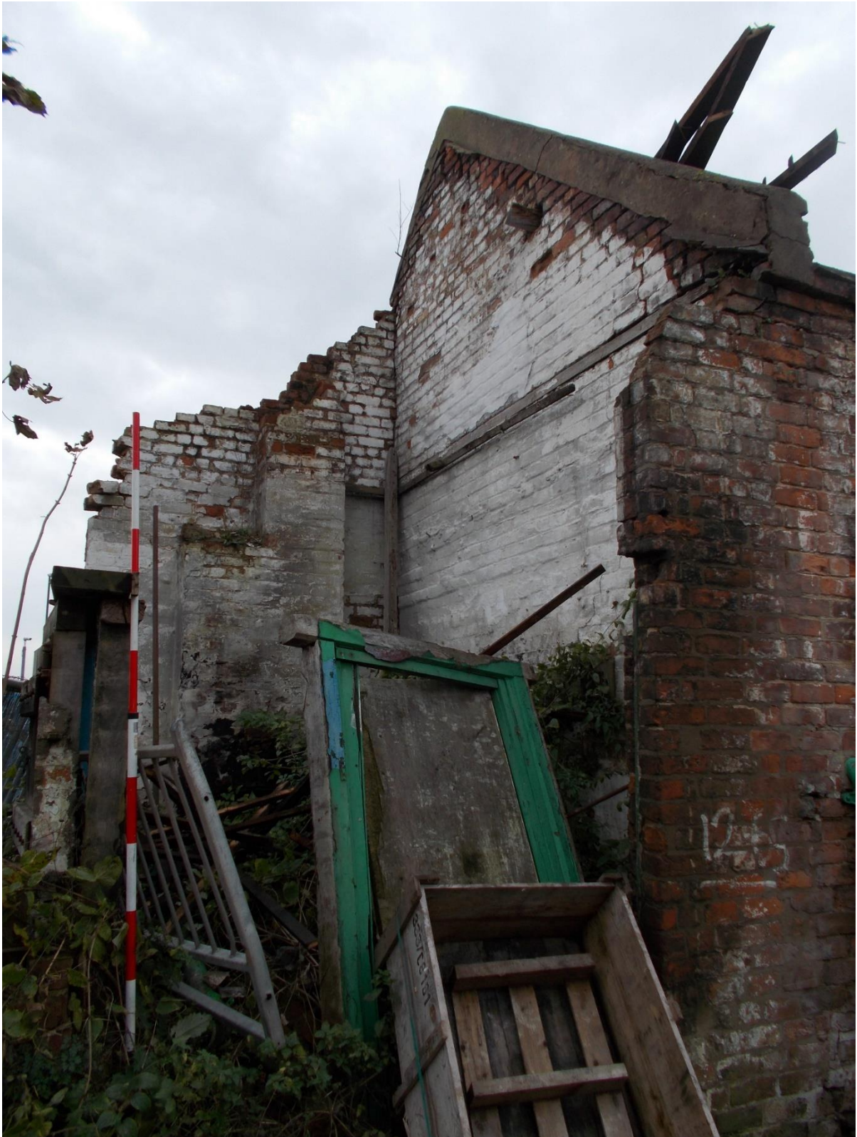
Plate 6: View looking SW showing detail of door jamb and door frame in N-elevation of Building B and stepped chimney flue in thickness of S-wall
