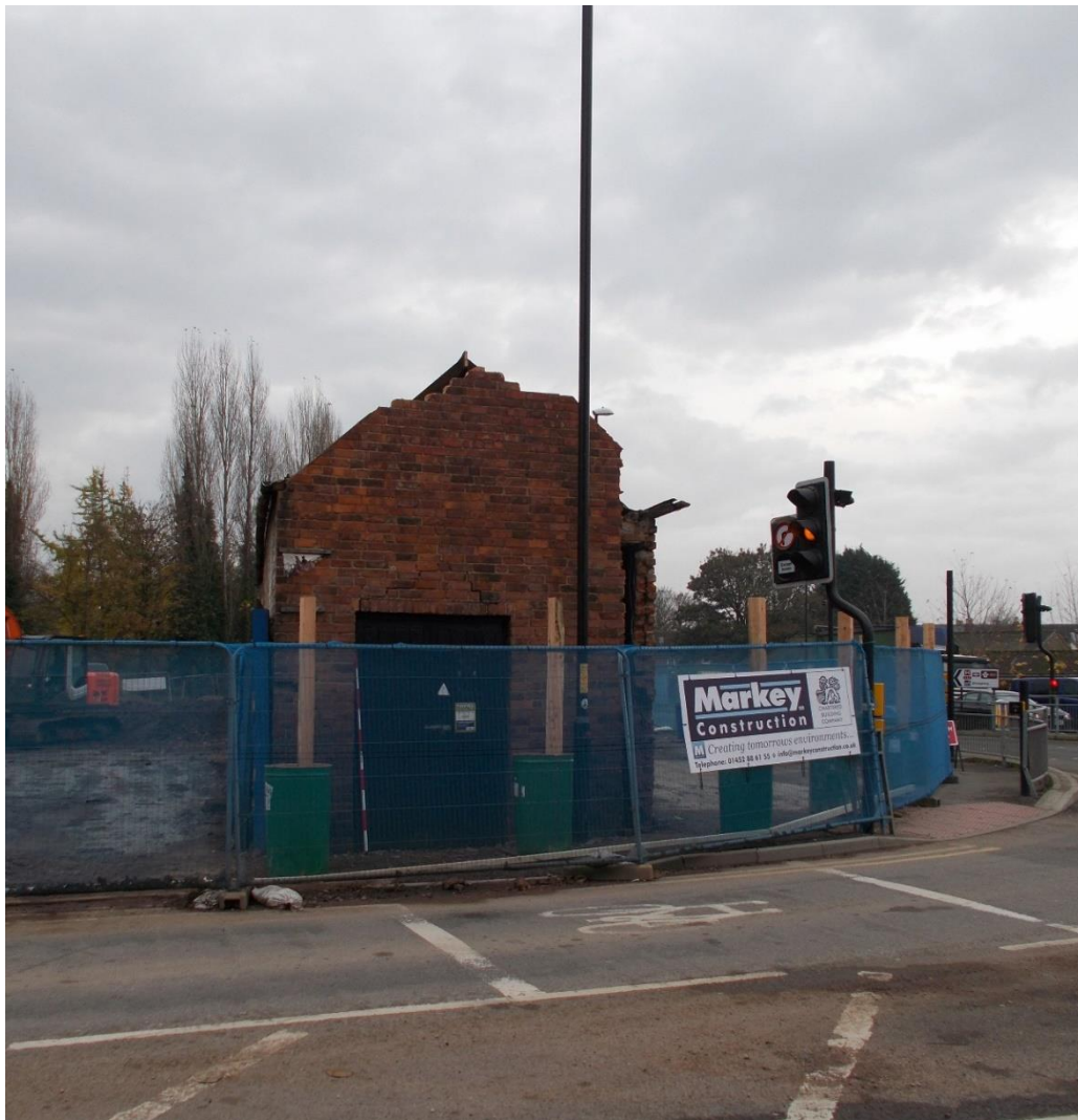
Plate 1: View looking E showing W-facing gable end of former sub-station fronting onto Southgate Street at junction with Trier Way
