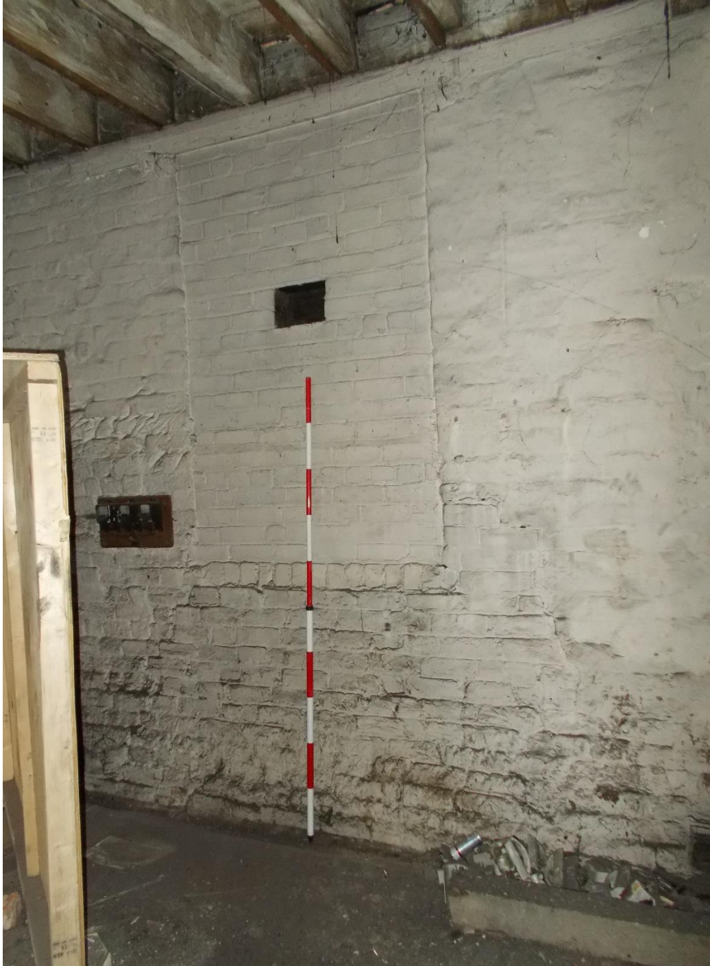
Plate 11: Internal view looking NW showing blocked up window with modern ventilation grille at W end of N wall, with indentation for possible partition wall visible to right of window
