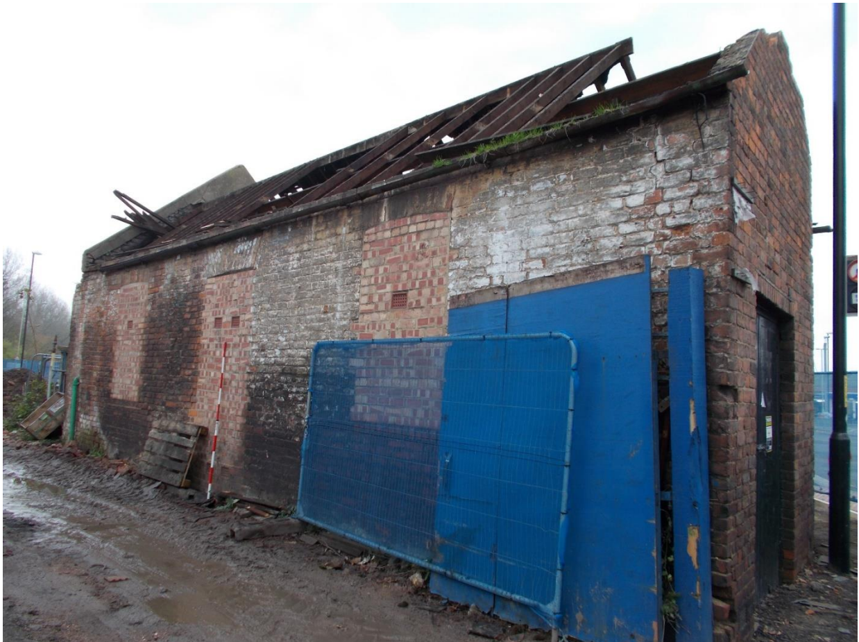
Plate 2: View looking SE showing N and W facing elevations of the former electricity sub-station (Building A) and the more steeply pitched roofline of the range attached to the E end (Building B)
