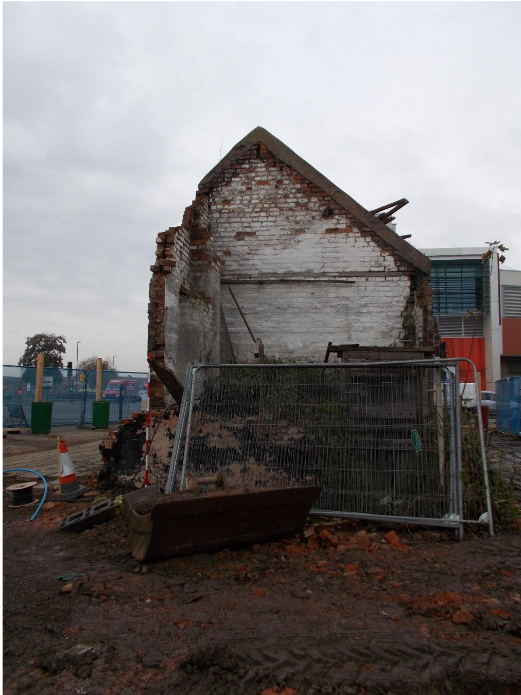
Plate 7: View looking W showing interior of Building B at E end of former sub-station with remains of chimney flue in thickness of S-wall
