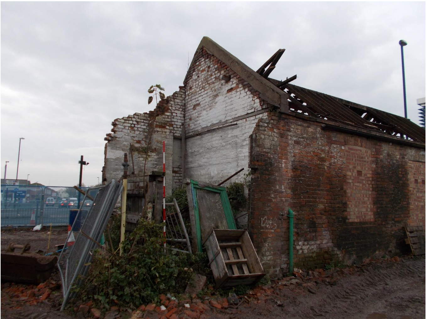
Plate 5: View looking SW showing largely demolished remains of gabled range (Building B) at E end of former sub-station building
