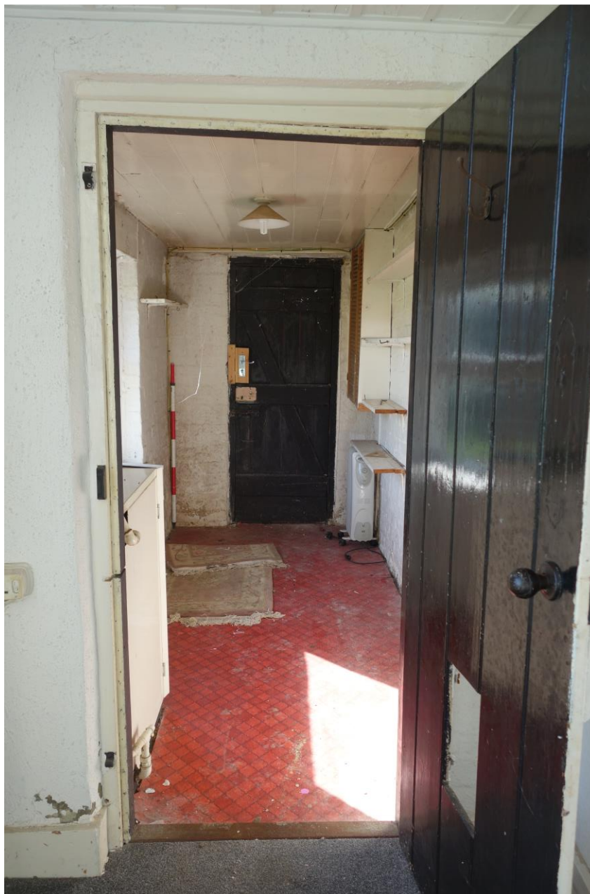
Plate 15: Boiler Room with plank ledged and braced doors viewed from Rear Hall showing bead-and-butt panelled ceiling aligned N/S.
