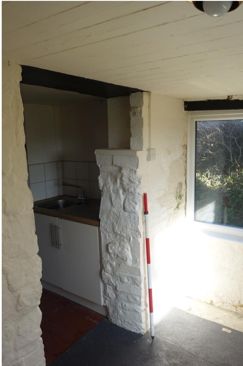
Plate 10: View from Pantry through into Kitchen showing 400mm thick stone wall built up with brick, with planked ceiling above.
