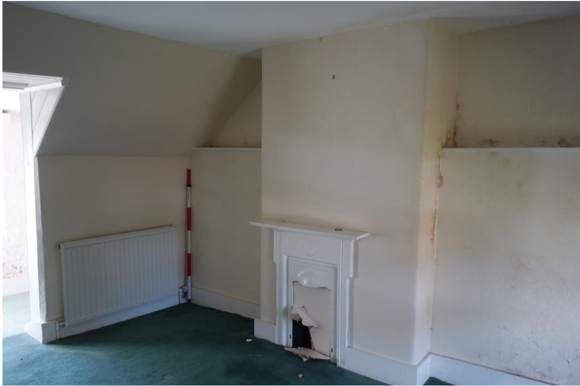
Plate 20: Bedroom 3 showing in-situ blocked sculpted cast-iron fireplace and timber-lined dormer-style opening through to adjacent room and Rear Hall (Upper).
