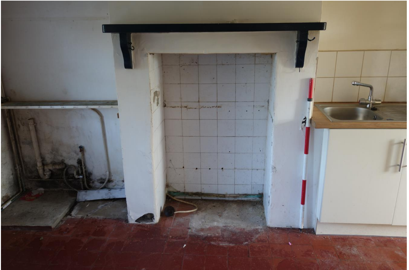
Plate 8: N wall of Kitchen showing fireplace probably intended to accommodate a cast-iron range.
