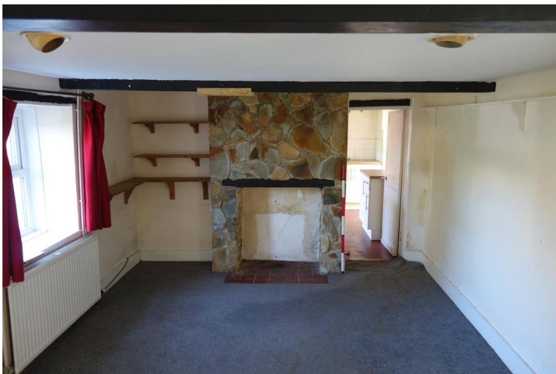
Plate 11: N wall of Living Room with view through to Kitchen showing modern decorative chimney breast and exposed E/W ceiling beams. UPVC window to left of picture in principal (W) elevation.
