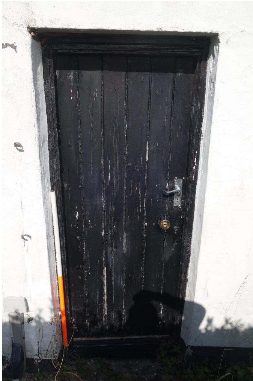
Plate 6: External plank and batten door in front (W) elevation opening into Kitchen.
