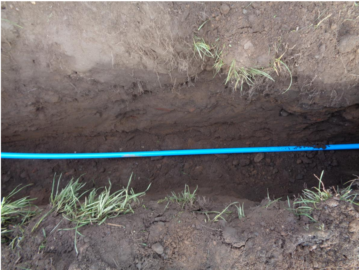
Plate 1: NE-facing section of Trench 1 showing modern ground disturbance containing brick, metal and plastic.
