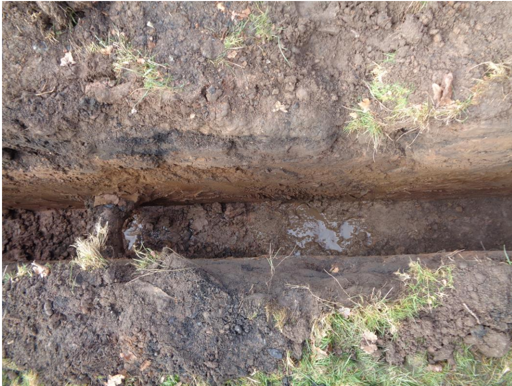
Plate 6: View of Trench 3 showing disused waterpipe.
