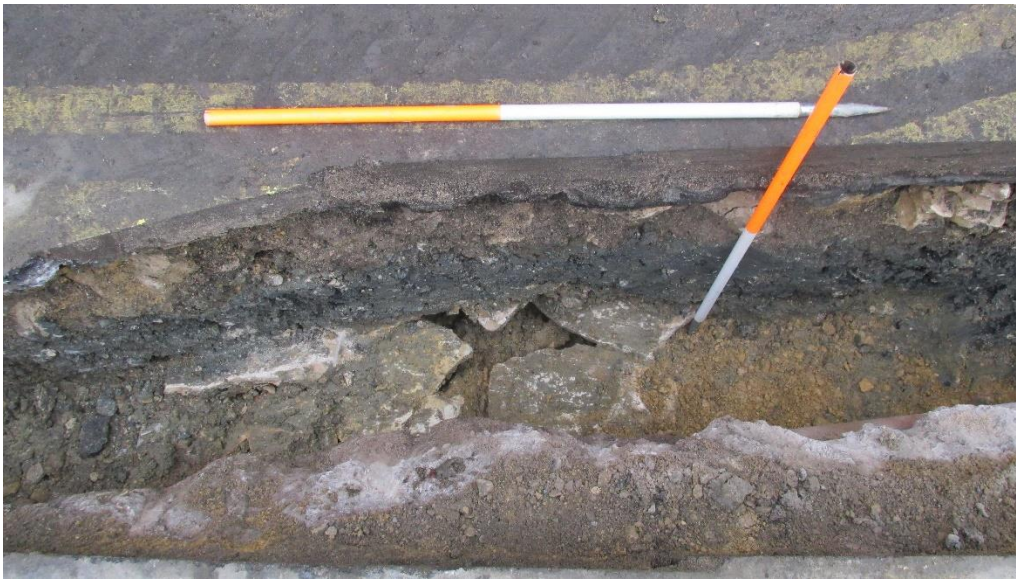
Plate 7: Back Lane: capping stones of 18 th / 19 th century masonry culvert (1008) and sealing deposit (1007). NW-facing section.
