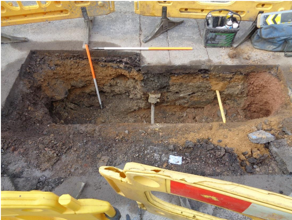
Plate 4: North Street: Extent of modern services [1003] running parallel and perpendicular to trench and pits. NE-facing section.
