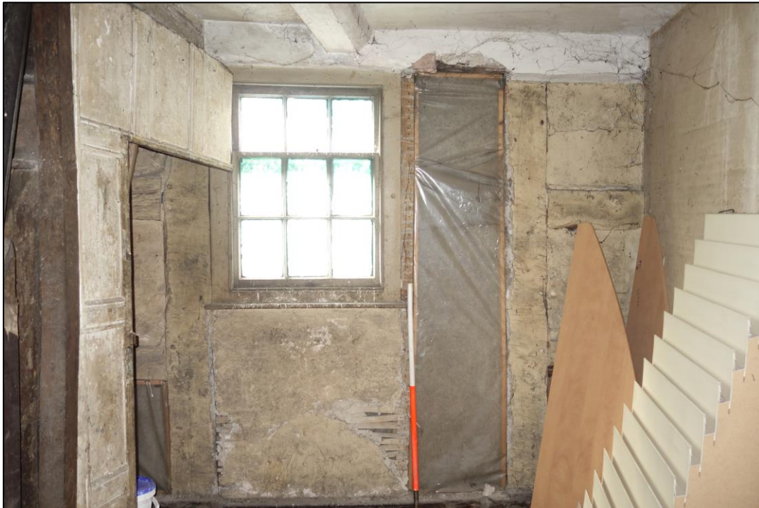
Plate 13: Internal view looking S showing SE compartment at first floor within No. 45, lit by sash window with section of oak panelling to left of picture
