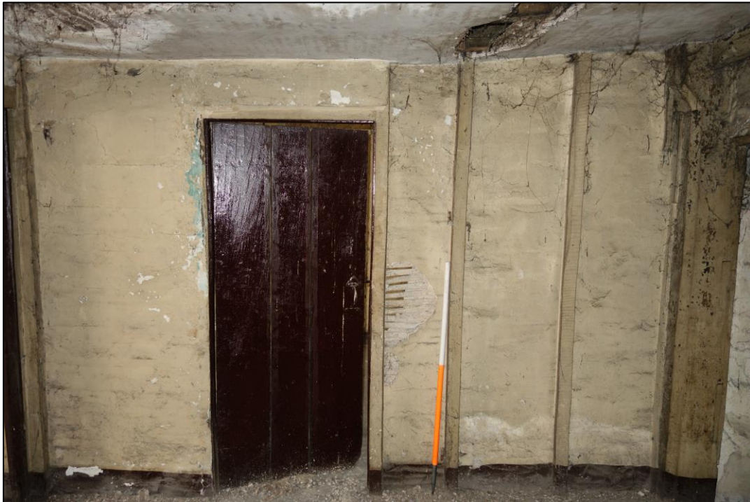
Plate 25: View looking N showing detail of N wall in SE room at second floor level (No. 45), with plank and batten doorway and close studding with lath-and-plaster infill, with jowelled vertical post at far right of picture
