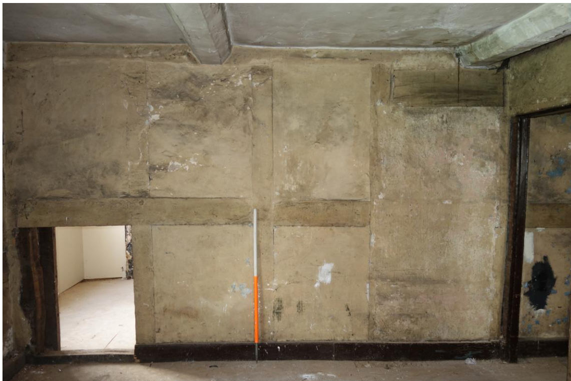
Plate 22: Internal view looking N within SW room at first floor level (No. 45) showing N wall with thick-scantled, square framed panels with lath-and-plaster infill clearly marking the division between No. 45 and No. 43 (to the N)
