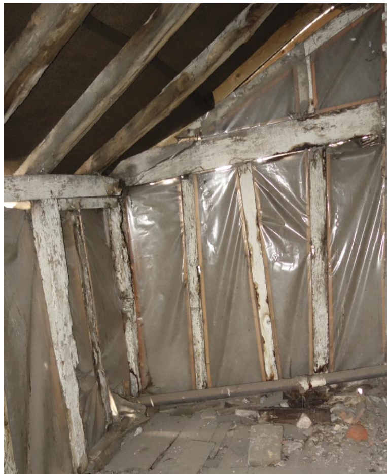
Plate 27: Internal view looking S showing detail of room in eastern extension at second floor level (No. 45) with thin-scantled timber-framing
