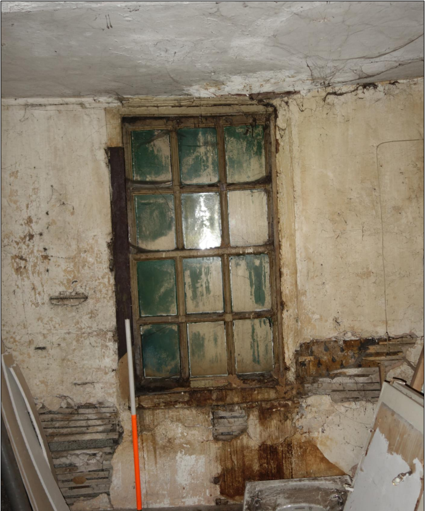
Plate 18: Internal view looking E showing 6/6 sash window in NE room on first floor (No. 45) with evidence of earlier painted wall decoration visible to right of window frame, concealed by later lath-and-plaster work
