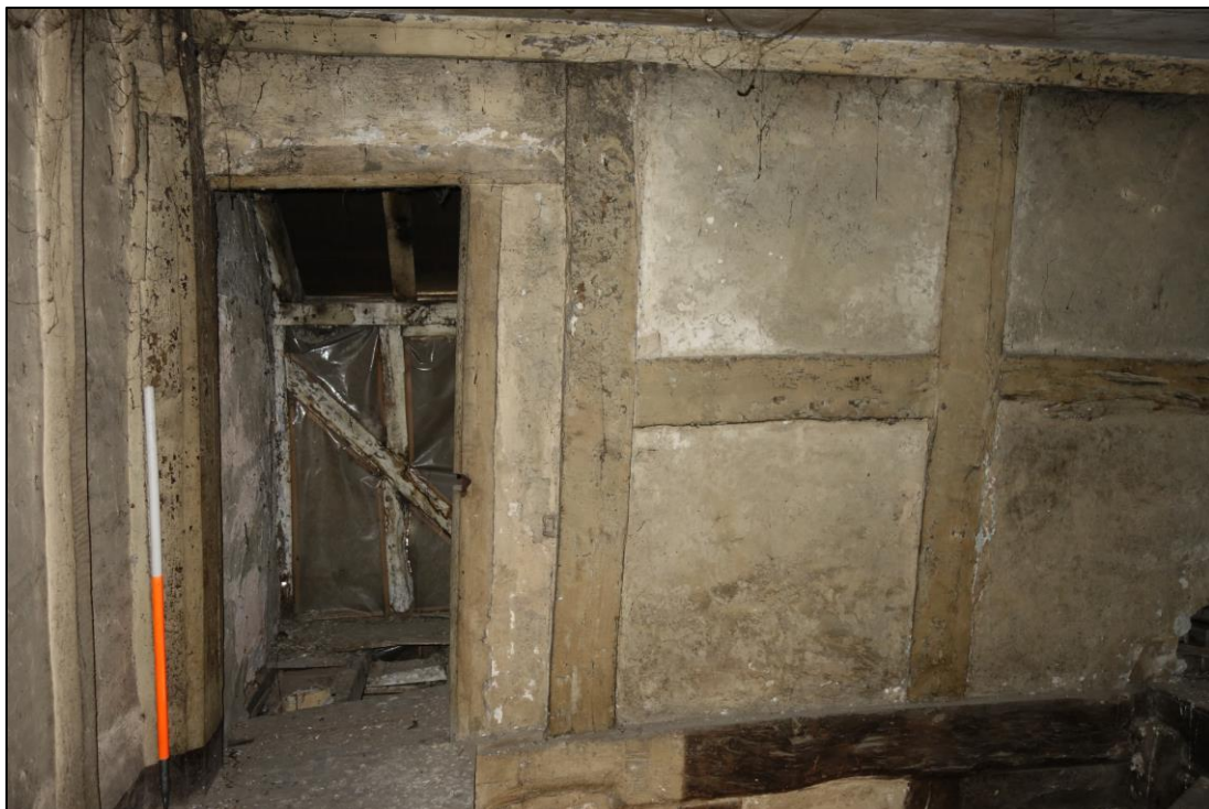
Plate 26: Internal view looking E showing detail of E wall of SE room at second floor level (No. 45), with later flat headed doorway leading to E extension, inserted within a section of thick-scantled square framed panels with jowelled chamfered post with infilled slots for horizontal rails to left of doorway
