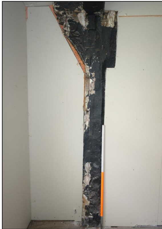
Plate 40: View looking N showing vertical jowelled post in westernmost bay of first floor room (No. 43) with enriched scrolled bracket and slots for horizontal rails, formerly denoting the W end of the house
