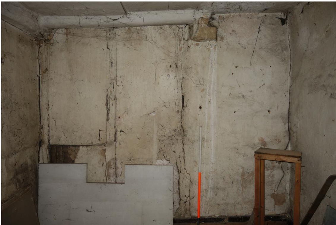
Plate 19: Internal view looking W in NE room on first floor (No. 45) showing close studded partition wall at W end of room and possible location of former fireplace in NW corner
