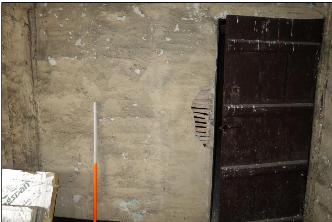
Plate 30: Internal view looking S showing S wall of NE room at second floor level (No.45) with plank and batten door and exposed lath-and-plaster work to left of picture
