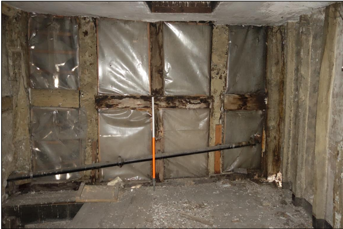
Plate 23: Internal view looking S showing SE room at second floor level (No. 45) with exposed square-framed, thick-scantled panels in the S wall and a hatchway in the ceiling leading to the roofspace
