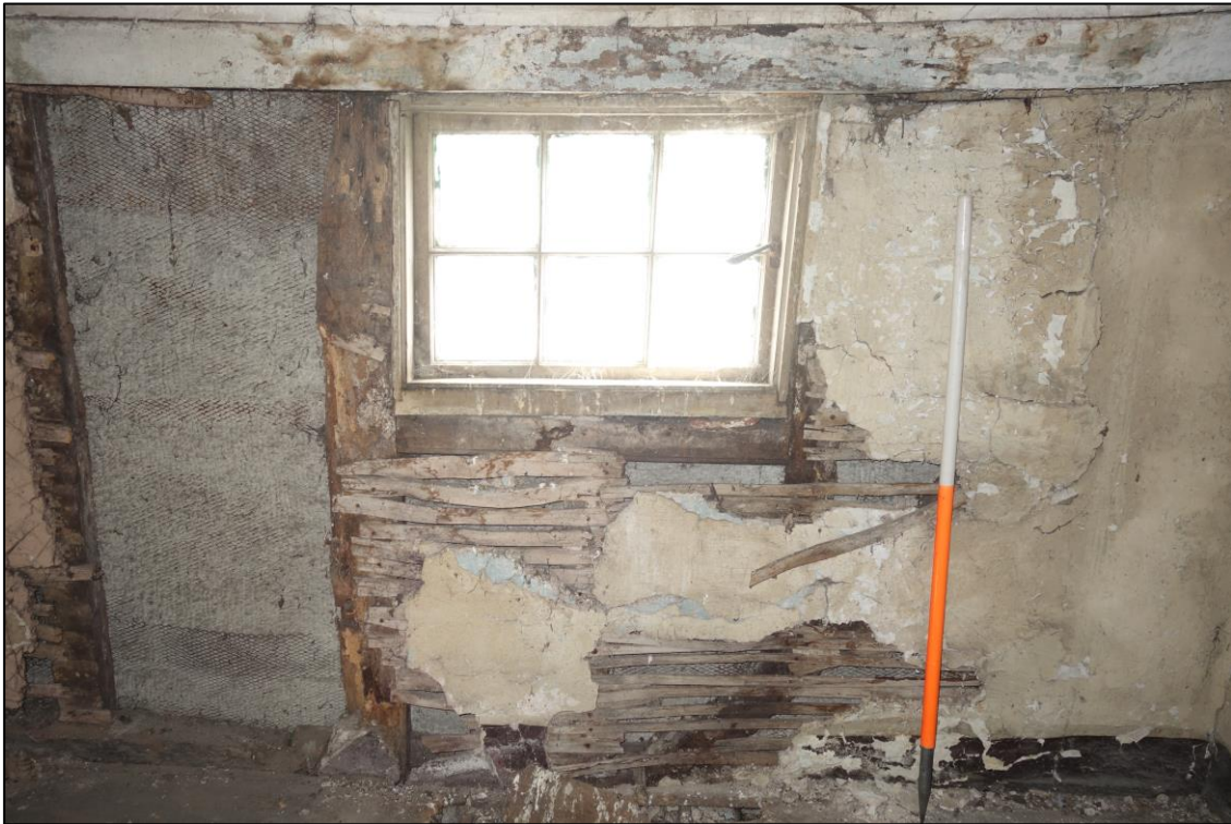
Plate 29: Internal view looking E showing 6-pane casement window in E wall of NE room at second floor level (No. 45) with exposed studding and lath-and-plaster work below
