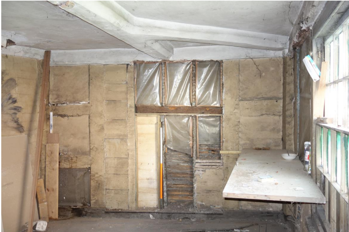
Plate 21: Internal view looking S within SW room on first floor (No. 45) showing exposed lath-and-plaster work in S wall and diagonal dragon beam in ceiling
