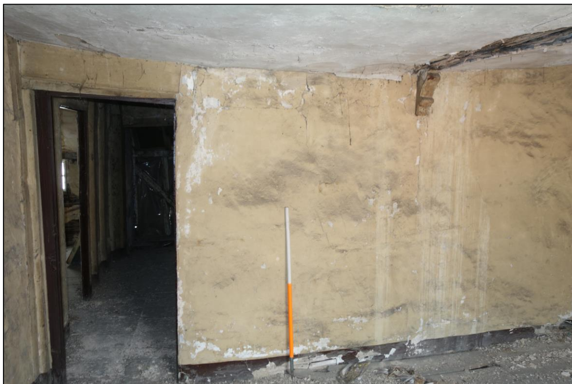
Plate 34: Internal view E showing flat headed doorway in NE corner of E wall of SW room at second floor level (No. 45) with carved wall bracket to right of picture
