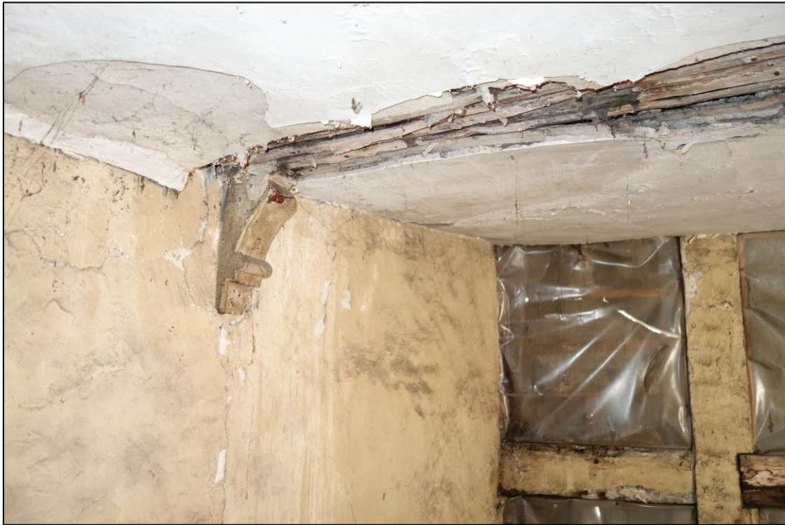
Plate 38: Internal view looking SE showing double ogee moulded bracket with traces of painted decoration on E partition wall of SW room at second floor level (No. 45)
