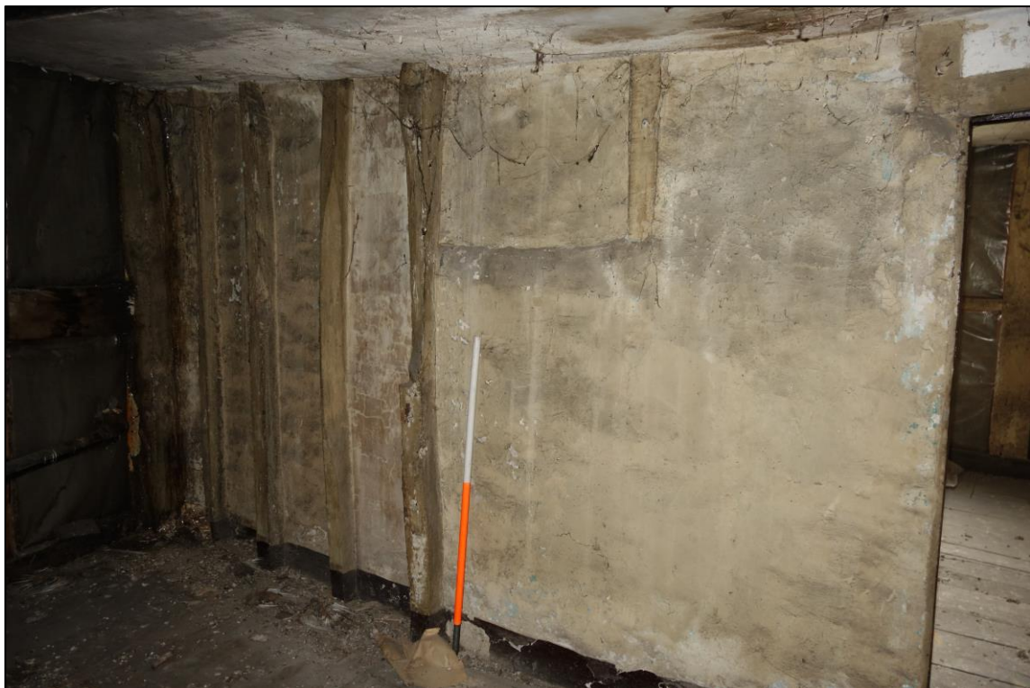
Plate 24: Internal view looking SW showing detail of close-studded wall with lath-and-plaster infill marking the division between the SE and SW rooms at second floor level (No. 45)
