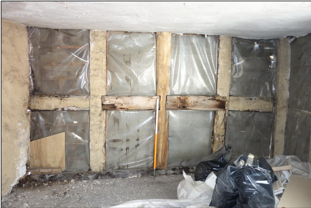
Plate 36: Internal view looking S showing square-panelled timber framing with thick scantling in S wall of SW room at second floor level (No. 45)
