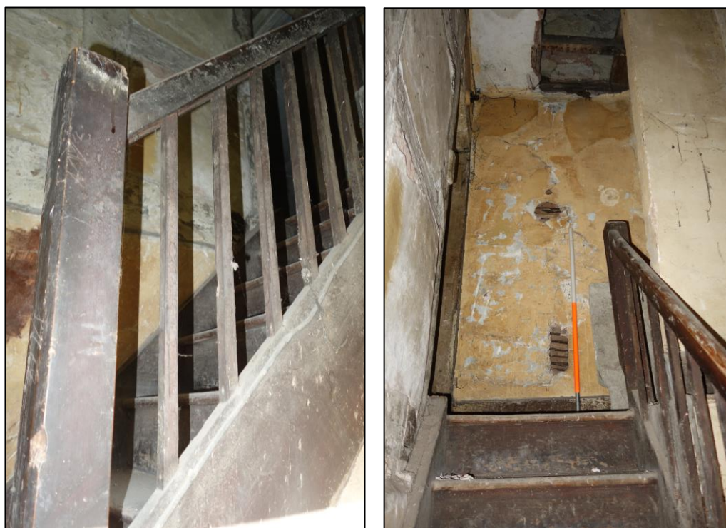
Plate 7: Internal view looking NW showing detail of ground floor staircase with newel post and stick balusters with evidence of square framed panels with thick scantling in background Plate 8: Internal view looking N showing upper part of staircase leading to first floor landing
