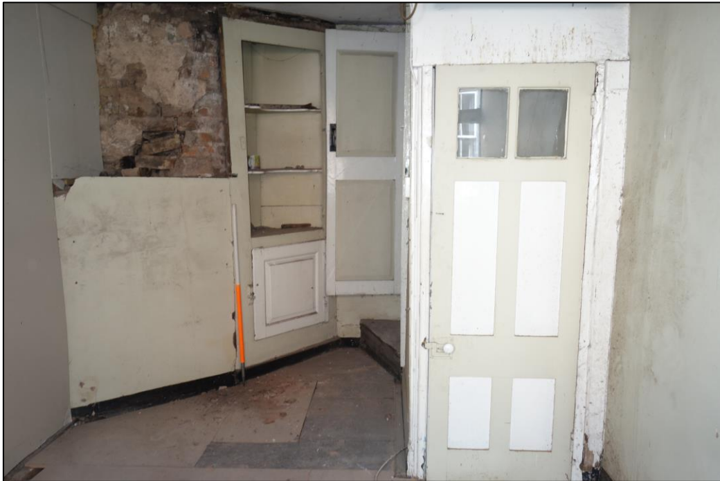
Plate 42: Internal view looking E showing E end of first floor room (No. 43) with brick chimneybreast and cupboard to left of picture and doorway formerly leading to a stairway to ground floor level (now blocked up)
