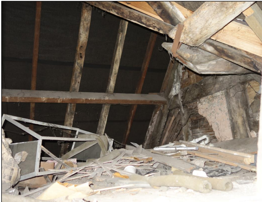
Plate 50: Internal view looking NE from hatchway showing detail of roof trusses within roofspace of No. 43
