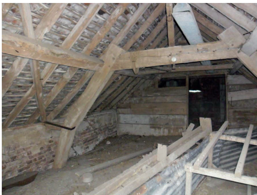
Plate 8: Internal view of upper storey of Barn A looking SW showing composite roof construction
