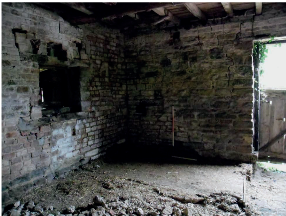
Plate 6: Internal view looking NE showing the makeshift timber lintel and slots inserted in the window of the NW elevation of Barn A
