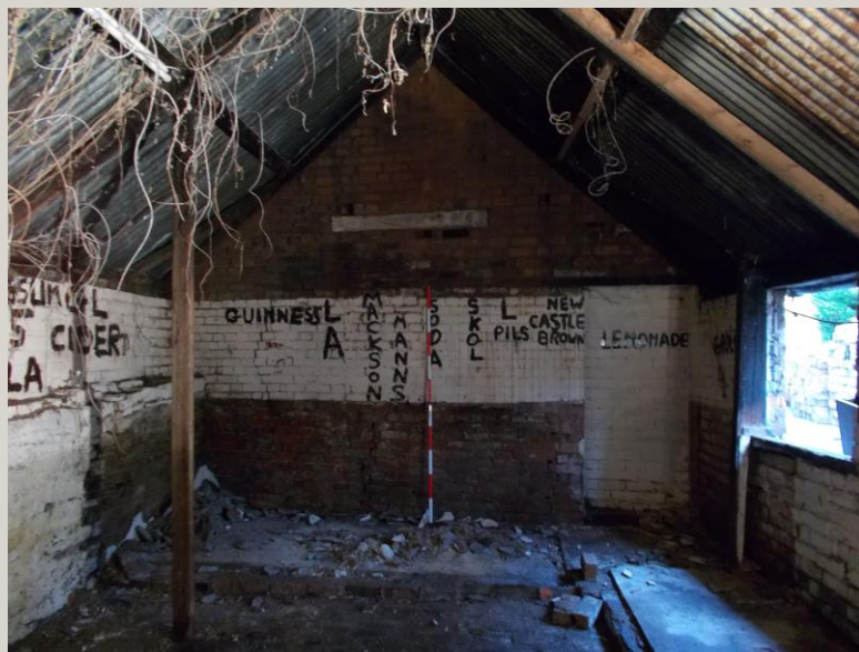
Plate 5: Internal view looking N of S elevation of Area 2, showing bricked-up doorway and corridor extending along the E side of the Area 1 building; the wooden sill for a possible pitching door is also visible in this picture
