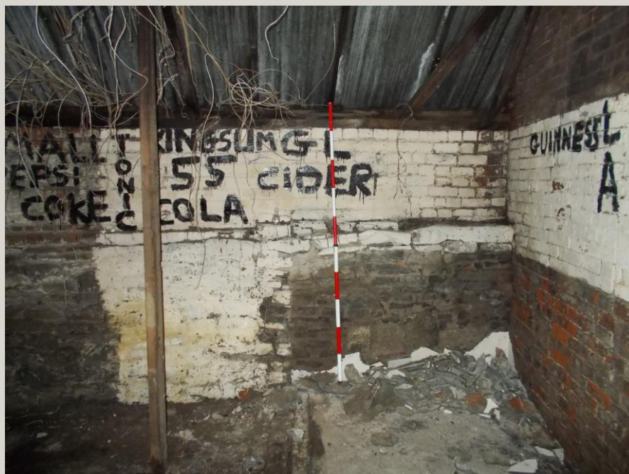
Plate 1: View W of extant boundary wall forming lower structure of western elevation of outbuilding (Area 1)
