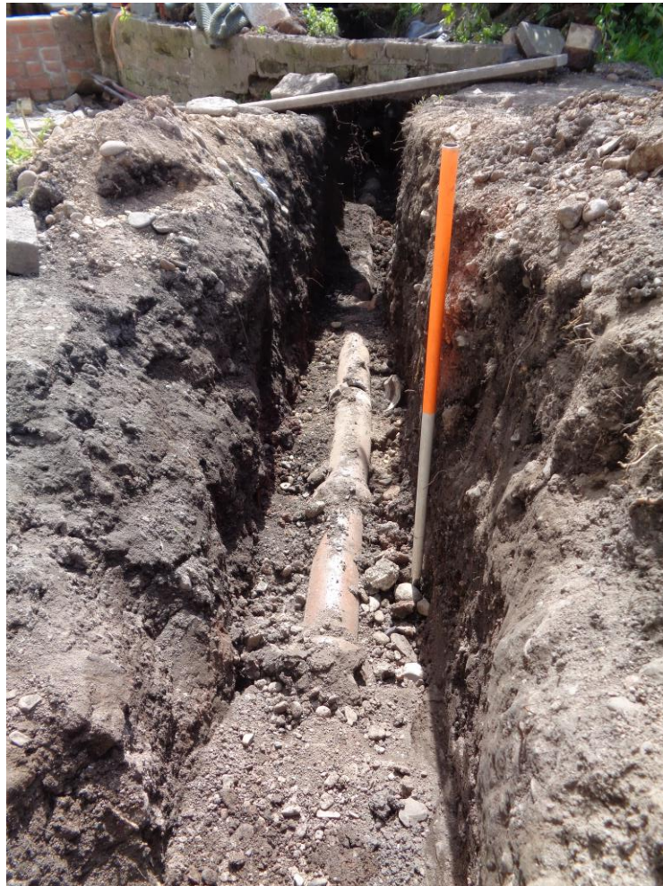
Plate 6: View SW of Drainage Trench 003, showing garden wall (005005) and drain pipe in [005003]
