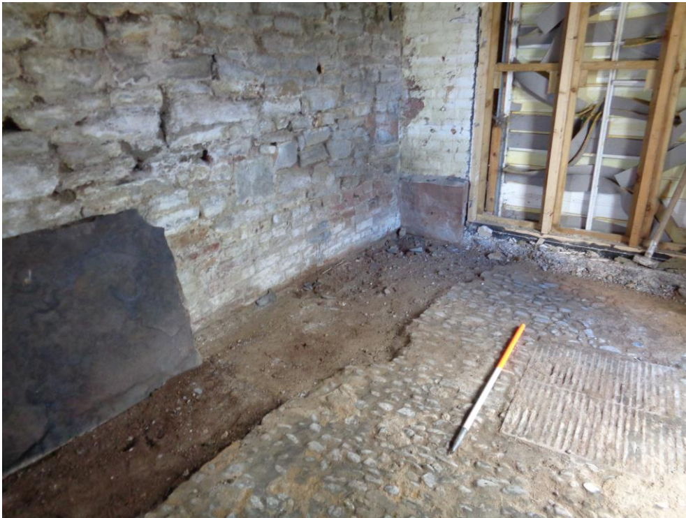
Plate 2: View S of Room 001 showing cobble surface (001002) with a central drainage grate
