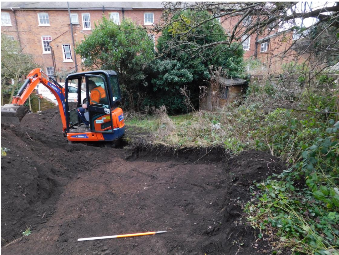
Plate 1: View S of work completed on W side of site, showing contexts (1001) and (1002).
