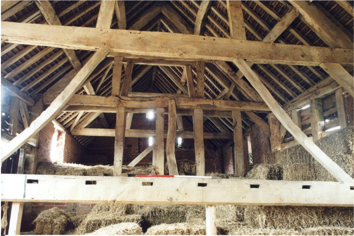
PLATE 3 BARN I SHOWING OAK TIMBER A-FRAME CONSTRUCTION WITHIN THE ROOF SPACE OF PHASE 1
