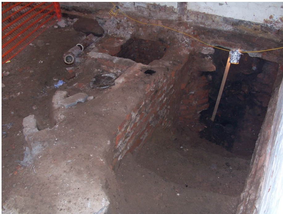
Plate 7: Internal view looking N showing area of stepped excavation in NE corner of room revealing evidence of brick walling (207) and segmental archway (220) leading to cellarage
