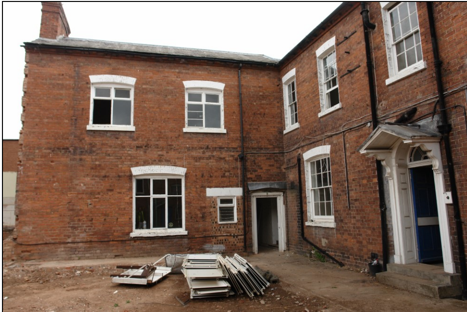
Plate 10: View N showing two-storey gabled extension to W of the main house built c.1875
