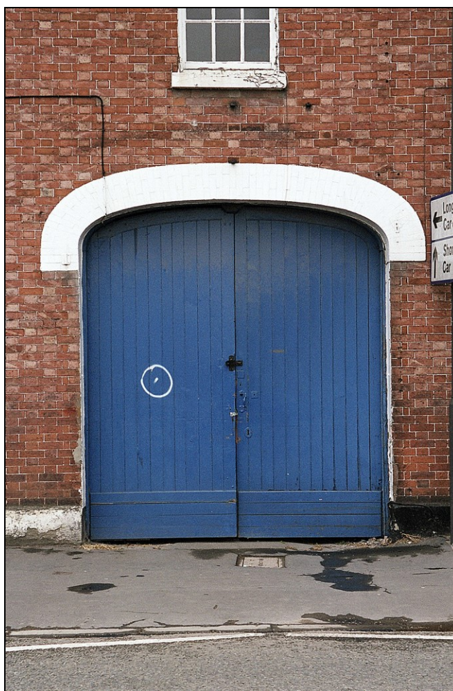
Plate 5: View W showing elliptical gauged brick carriageway arch to the left of the house, with 12-paned sash window above
