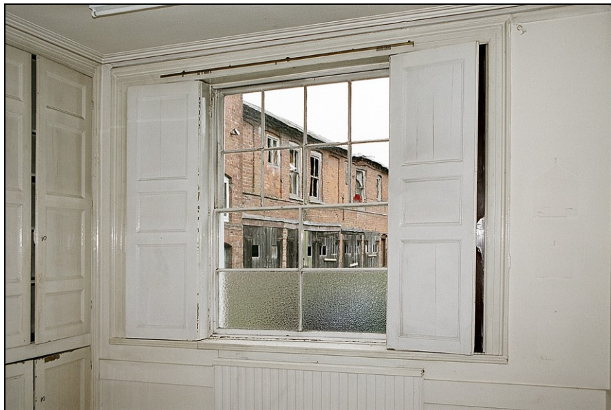
Plate 33: View W showing altered 12-pane sash window within a fluted architrave with panelled cupboard to the left
