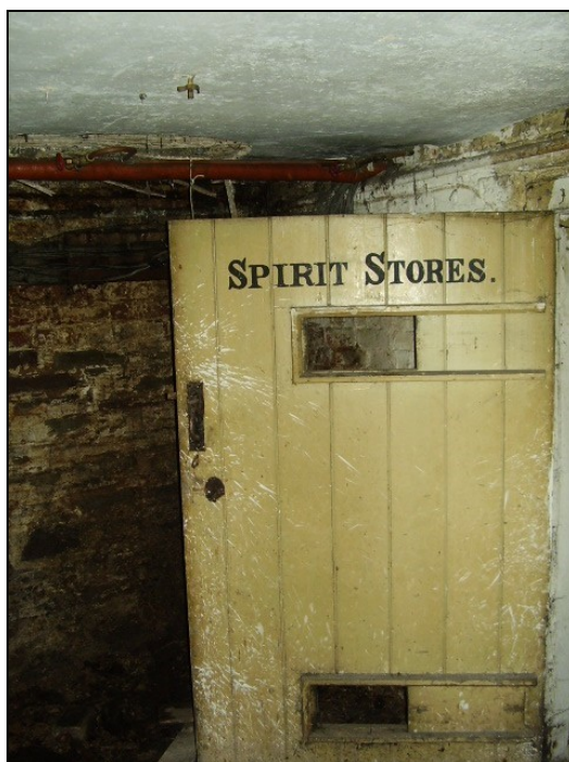
Plate 20: View showing late 19 th century plank-and-batten door marked 'Spirit Stores'
