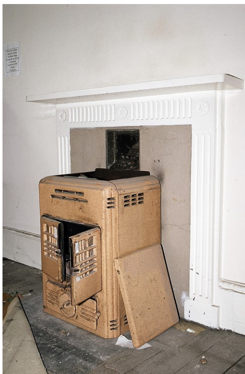
Plate 66: View SW showing 1950s stove hob set into late 19 th century fluted wooden surround and mantel
