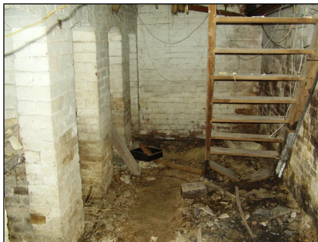
Plate 23: View N showing wooden stairway to ground floor on right, opposite which is a series of recesses under narrow segmental-headed arches
