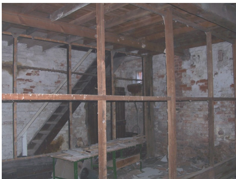
Plate 67: View SE showing stairway to first floor at E end of outbuilding range and cross-framed partitions for stalls
