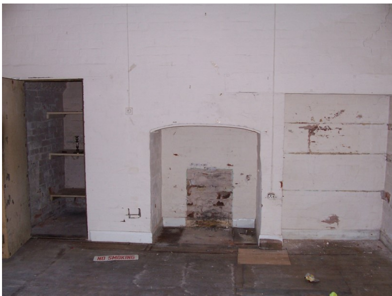
Plate 42: View showing interior of ground-floor room within later extension of c.1875 with central fireplace flanked by the strongroom (left) and deep recess in wall (to right)
