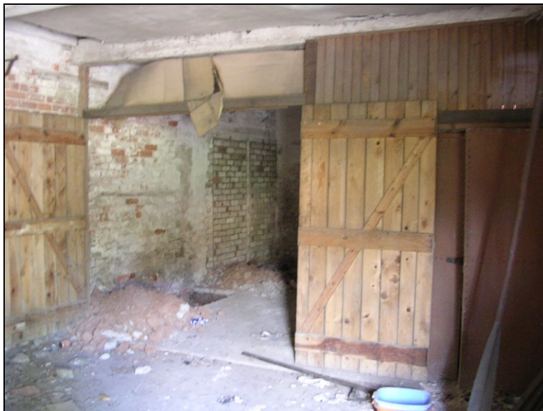
Plate 71: View W showing large single-celled compartment at W end of outbuilding range with a set of bricked-up double doors in the SW corner
