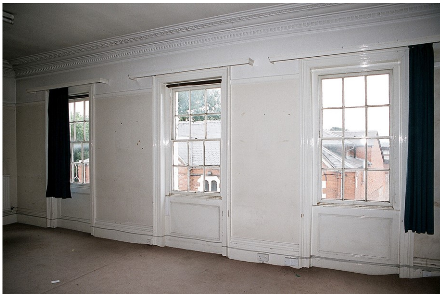
Plate 54: View NE showing 'drawing room' lit by three double- hung sash windows within fluted architraves, with elaborate moulded cornice above
