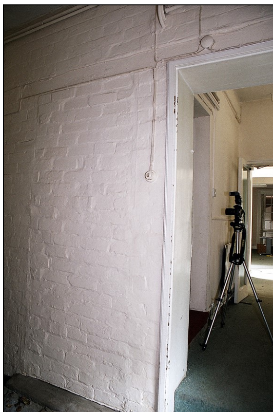
Plate 41: View E showing blocked doorway and stone threshold in ground-floor hallway within late 19 th century W extension to main house
