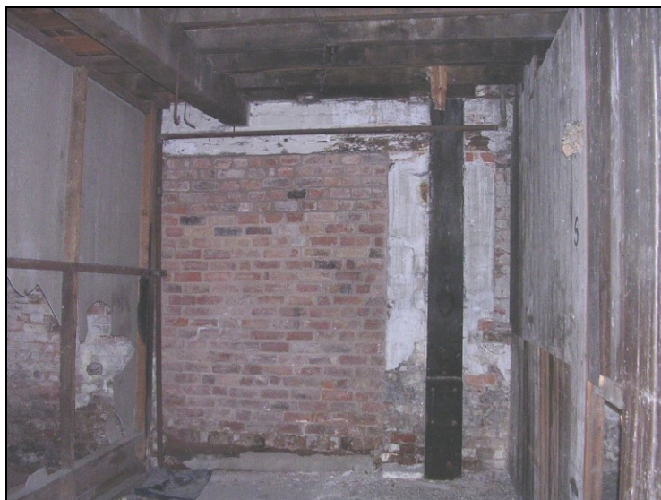
Plate 68: View S showing bricked-up rectangular door opening in S wall of outbuilding range
