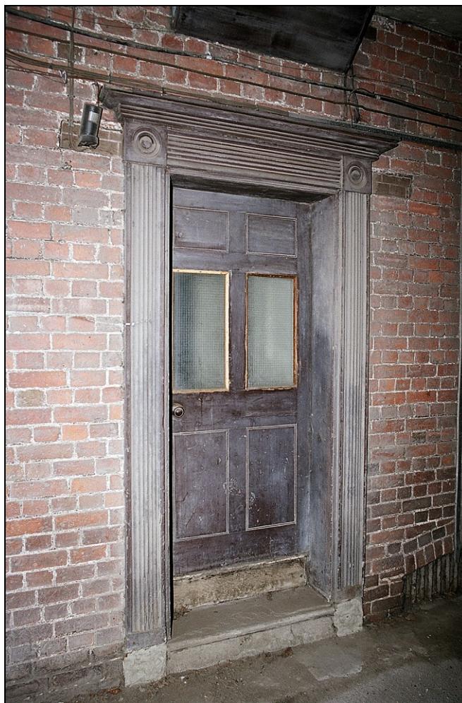
Plate 6: View looking NE showing doorway with reeded architrave and paterae in the N wall of the carriageway passage
