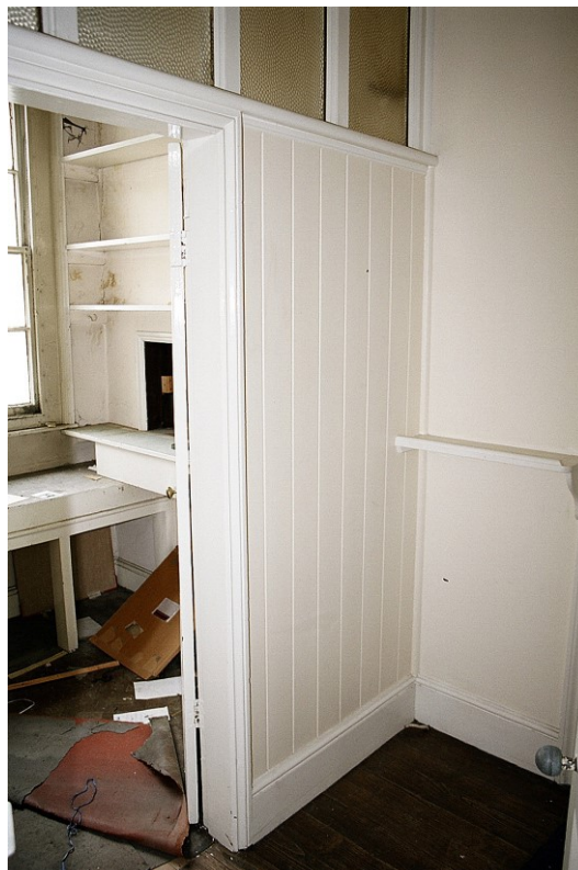
Plate 64: View NE showing modern panelled partition with four-light window above, with doorway to left leading to pantry
