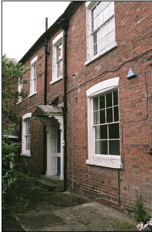
Plate 7: View looking N showing the rear (W-facing) elevation at No. 38 South Street
