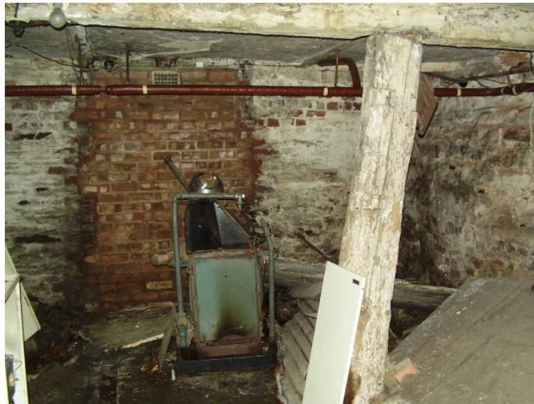
Plate 19: View S showing reused timber upright supporting beam across the ceiling, with drainage channel visible to left of picture
