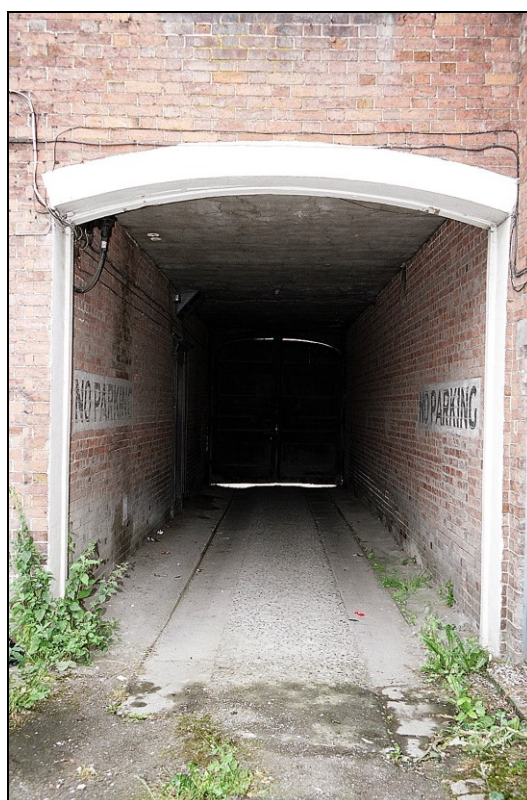
Plate 9: View E showing rear carriageway arch with metal tracks set into the carriageway surface to carry brewers' drays and carriages
