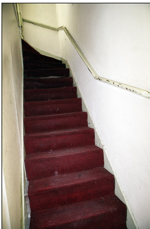
Plate 40: View looking N showing dogleg stairwell to first floor of late 19 th century W extension
