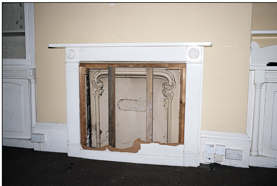
Plate 29: View S showing fireplace with late 19 th century ornated iron surround within earlier wooden surround with 'bullseye' paterae of Regency date (c.1830-40)
