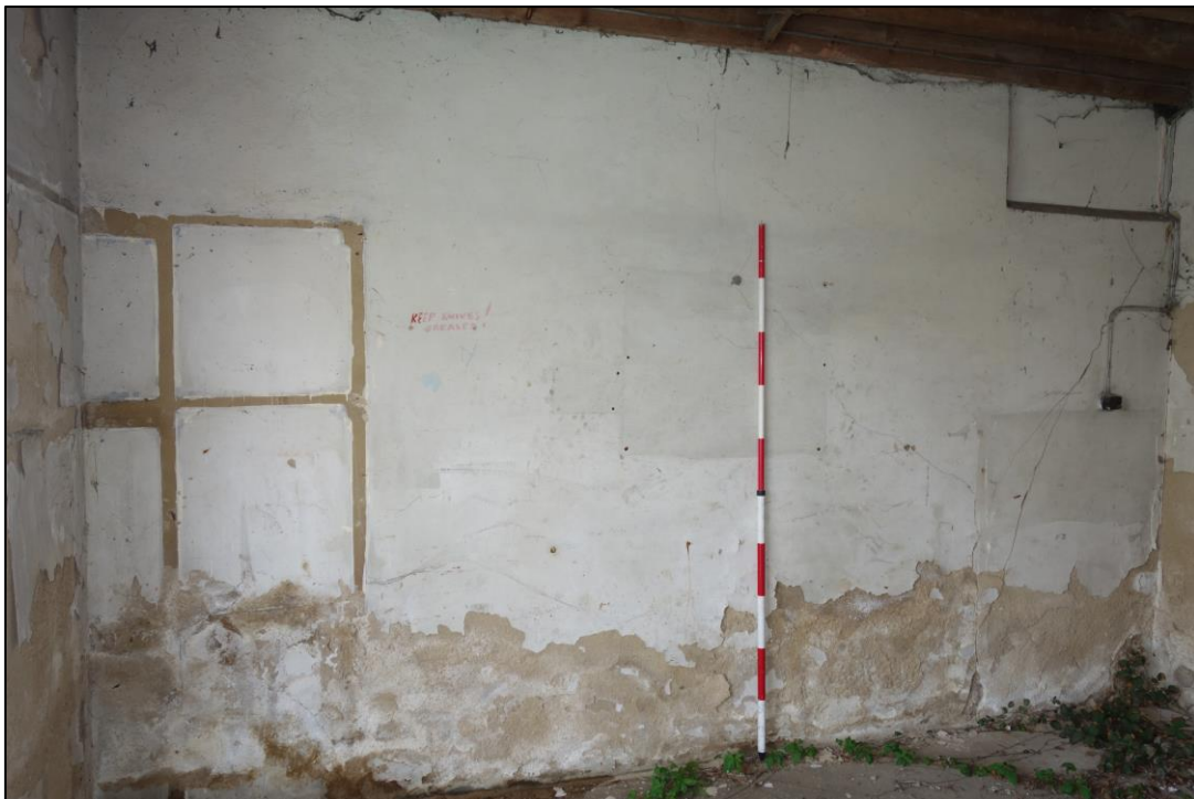
Plate 18: Internal view looking N showing N wall of southernmost compartment on ground floor showing lower part of blocked doorway to top right of picture
