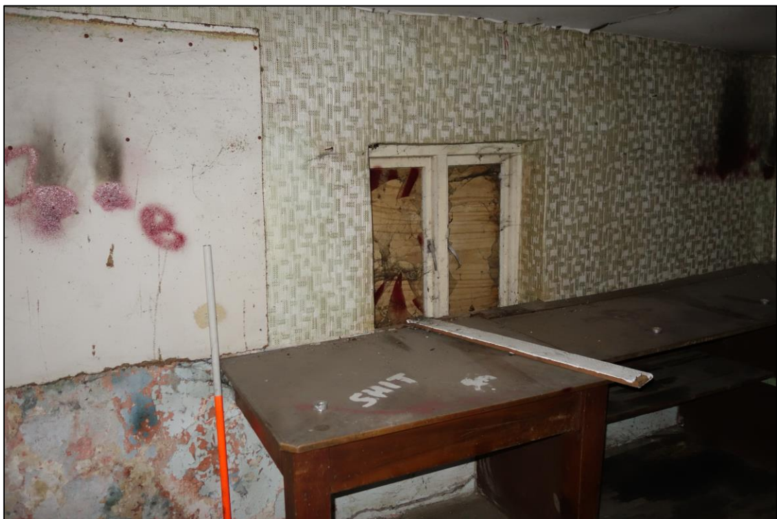
Plate 26: Internal view looking SE showing casement window in E wall of compartment to E of first floor landing
