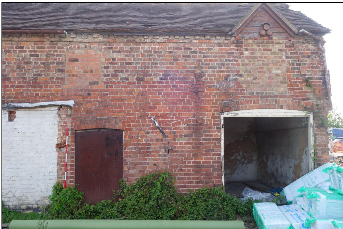
Plate 4: External view looking E showing detail of central and southern bays of principal W-facing elevation
