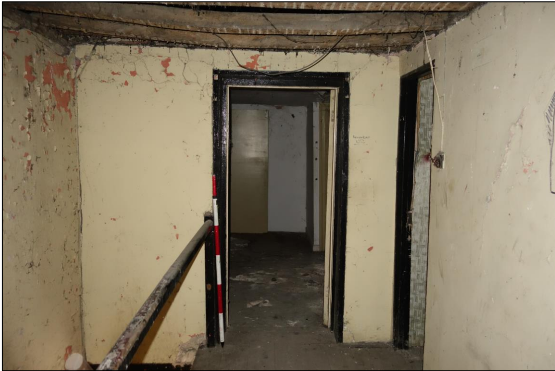
Plate 21: Internal view looking N showing rooms to N and E of first floor landing
