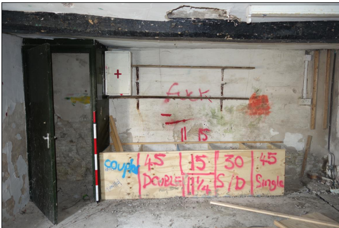
Plate 11: Internal view looking N showing northern compartment at ground floor level with chamfered ceiling beam
