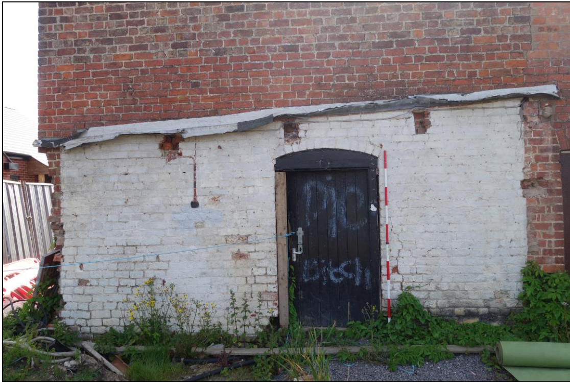
Plate 3: External view looking E showing detail of northernmost bay of W-facing elevation with segmental-arched doorway and roofline of demolished single-storey modern extension
