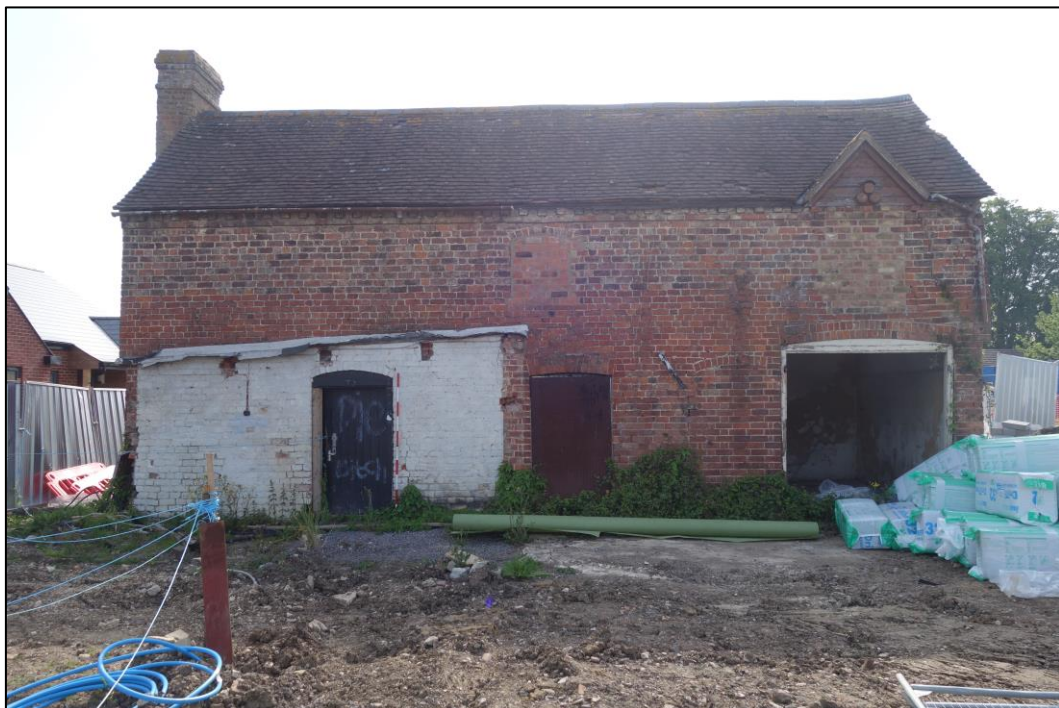
Plate 2: External view looking E showing principal W-facing elevation of the 'Old Coach House'
