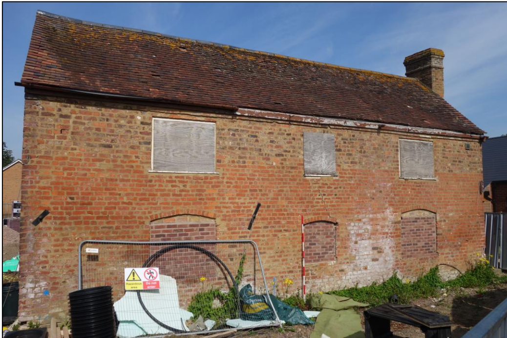
Plate 7: External view looking WNW showing rear (E-facing) elevation of 'Old Coach House'
