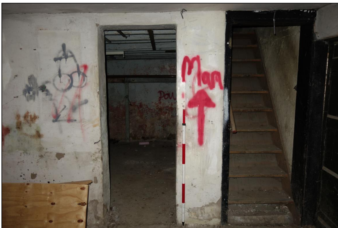
Plate 12: Internal view looking S showing doorway leading to central compartment at ground floor, to the right of which is a stairway leading to the first floor
