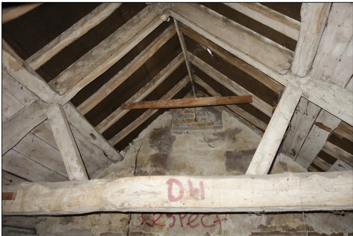
Plate 28: Internal view looking S showing exposed tie beam roof truss in loft compartment with blocked opening in apex of S wall
