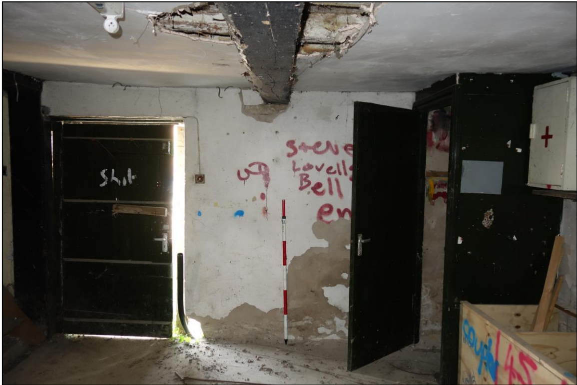
Plate 9: Internal view looking W showing doorway and modern cabinets in W wall of northern compartment at ground level
