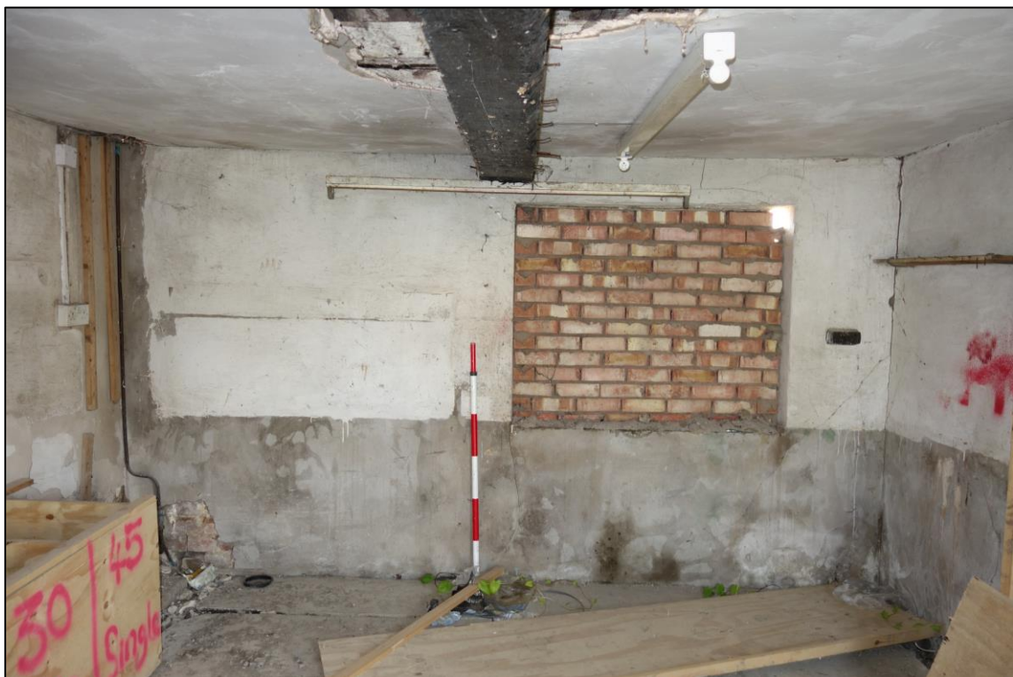
Plate 10: Internal view looking E showing blocked window in E wall of northern compartment at ground level
