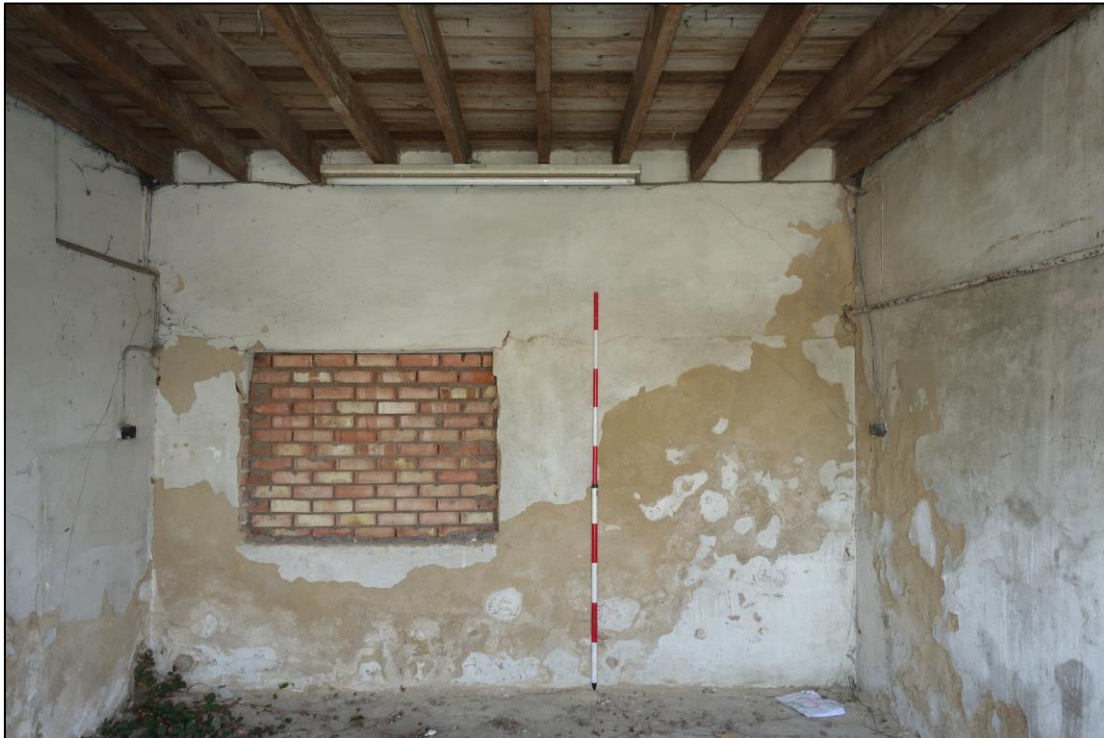
Plate 17: Interior view of southernmost compartment ('Coach House') at ground floor level, with blocked window in E wall and heightened ceiling
