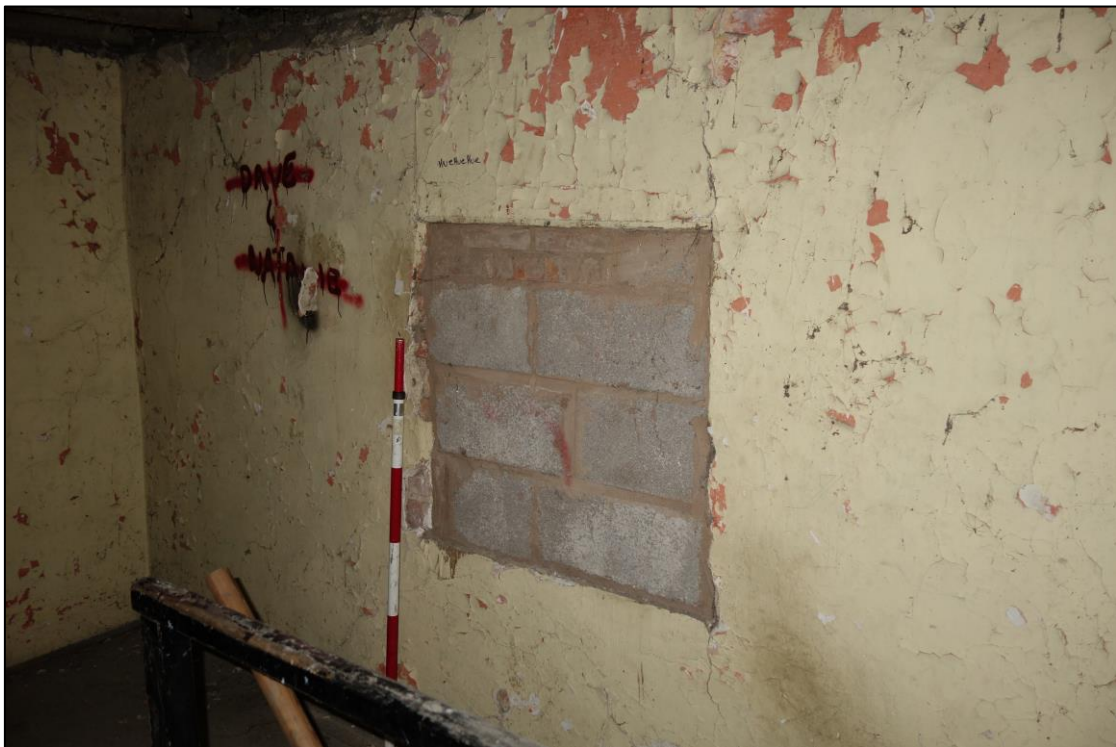
Plate 22: Internal view looking SSW showing blocked window in W wall of first floor landing
