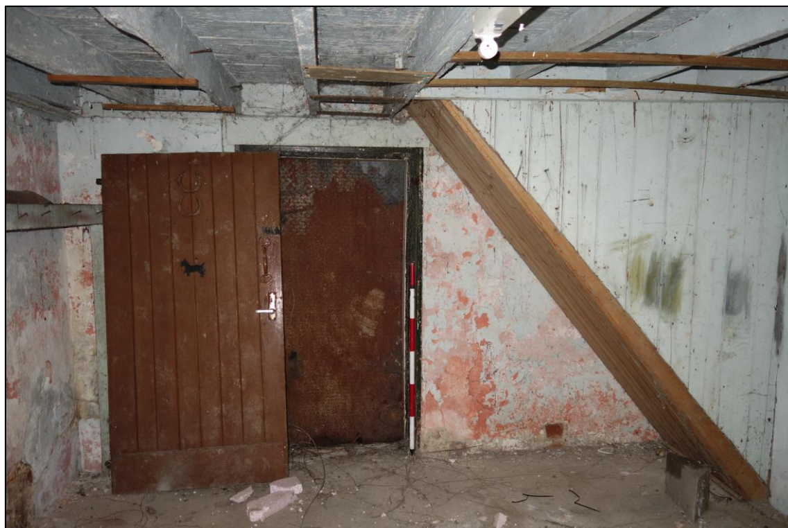
Plate 14: Internal view looking W showing doorway in S wall of central compartment on ground floor, adjacent to which is an earlier plank and batten door with horseshoes attached
