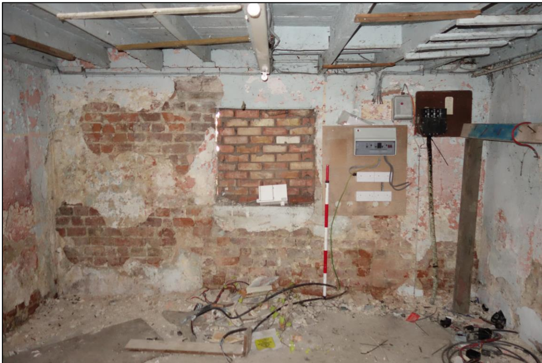
Plate 15: Internal view looking E showing blocked window in E wall of central compartment at ground floor level with exposed, whitewashed ceiling beams and joists
