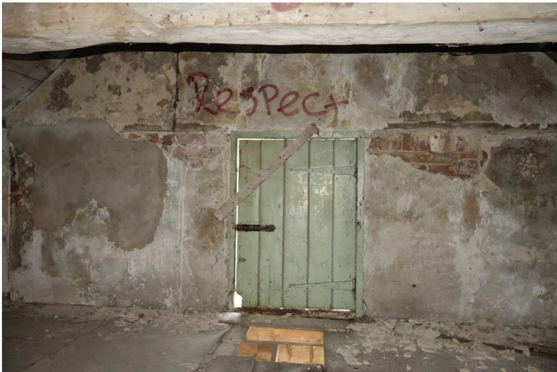
Plate 29: Internal view looking S showing plank and batten door in S wall of loft compartment, formerly leading to stable
