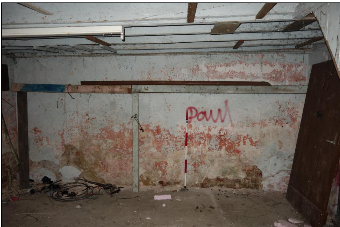
Plate 16: Internal view looking S showing S wall of central compartment on ground floor with wooden horizontal rails, possibly for hanging harnesses
