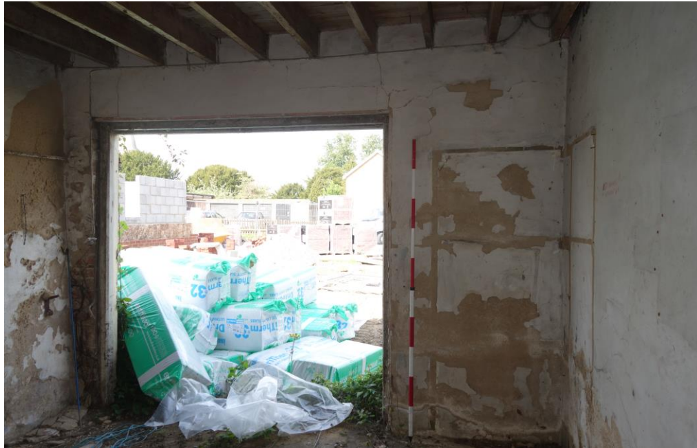
Plate 19: Internal view looking W showing W wall of southernmost compartment on ground floor with indentations for cupboards to right of doorway
