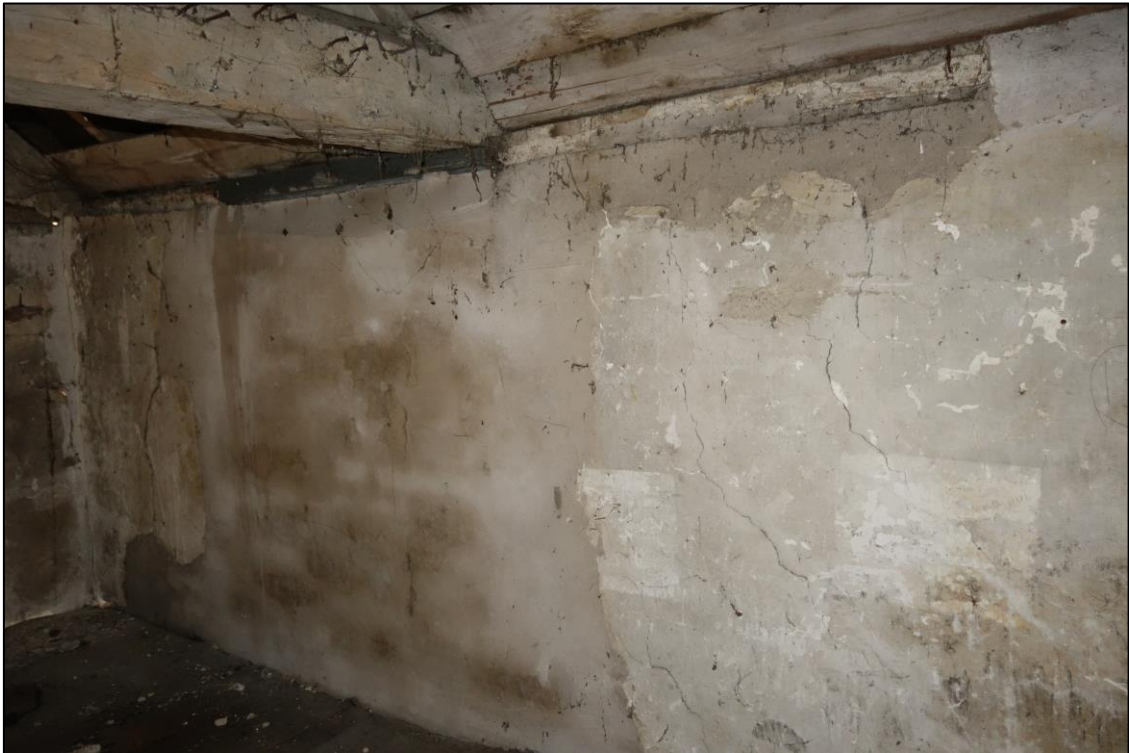
Plate 31: Internal view looking SW showing blocked window (with lintel) in W wall of loft compartment
