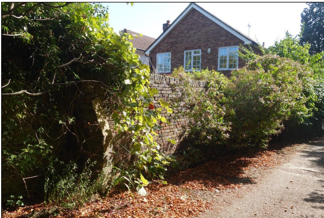
Plate 3: View looking ESE along driveway showing boundary wall partially concealed by foliage
