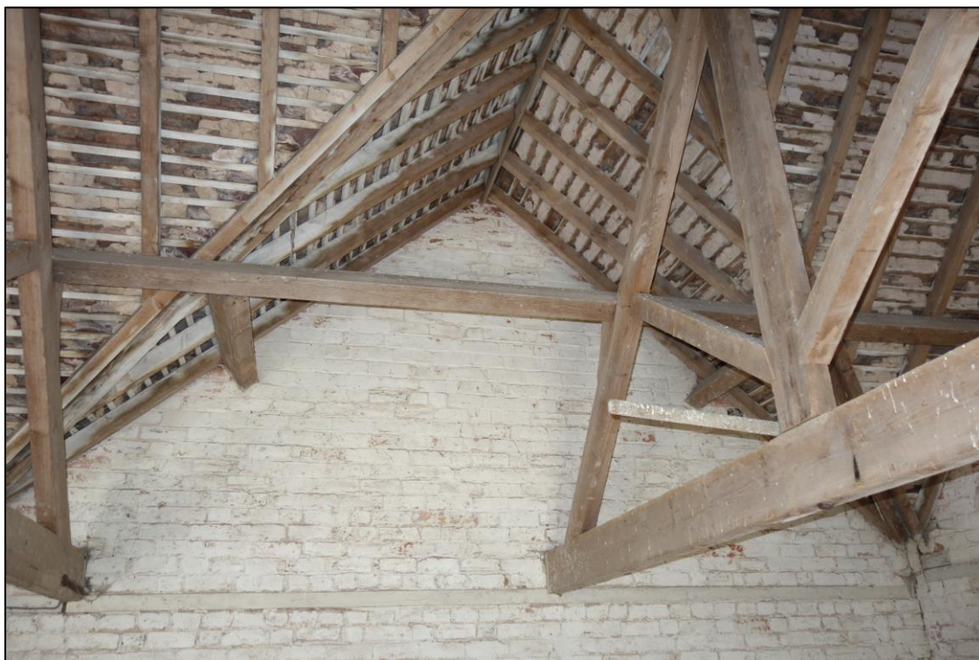
Plate 24: Internal view looking SE showing cross-gabled roof structure in SW bay of granary
