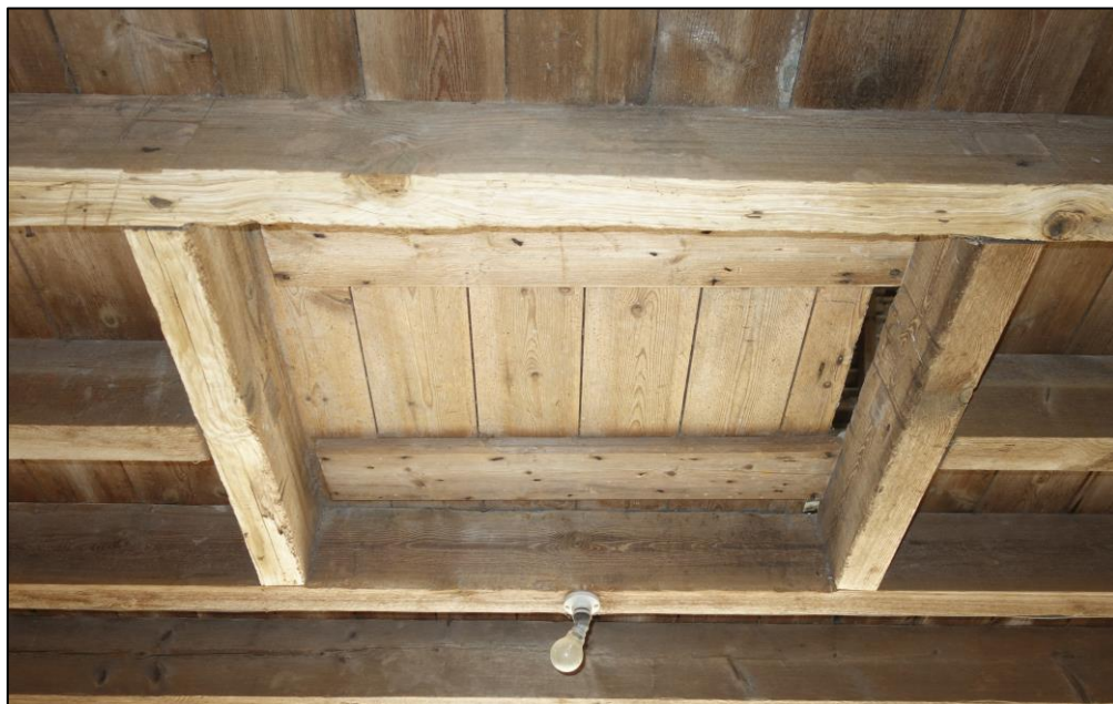
Plate 20: View looking SE showing detail of trap door in ceiling within southwesternmost bay of cartshed
