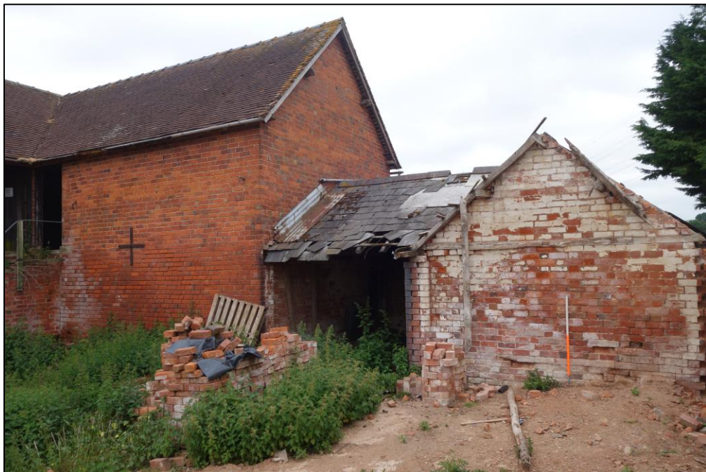
Plate 11: View looking NW showing gabled outbuilding with slate roof to NE of granary/cartshed
