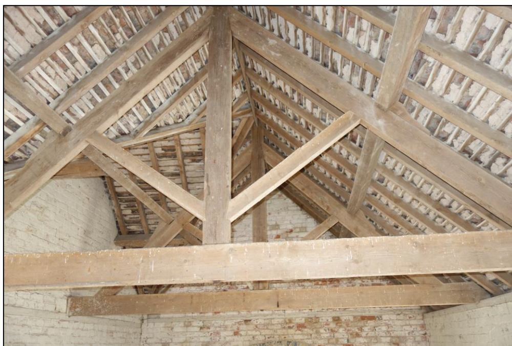
Plate 23: Internal view looking SW showing detail of kingpost roof trusses in granary with angled struts connecting the kingpost to the principal rafters, which are connected by a pair of trenched purlins
