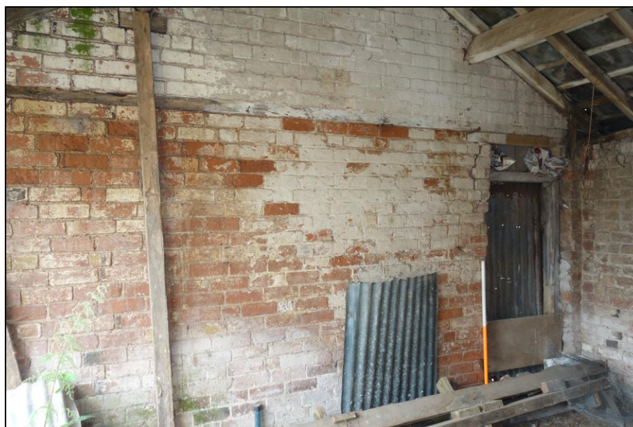
Plate 41: View looking W showing lower portion of NE wall of cartshed, partially whitewashed
