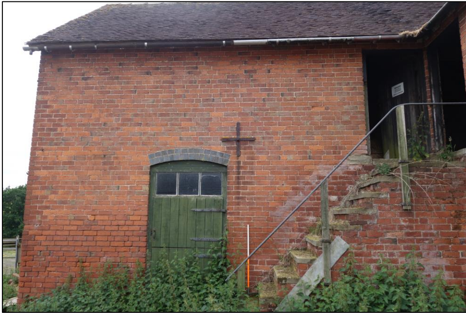
Plate 10: View looking SW showing detail of rear elevation of stable range with segmental-arched stable door
