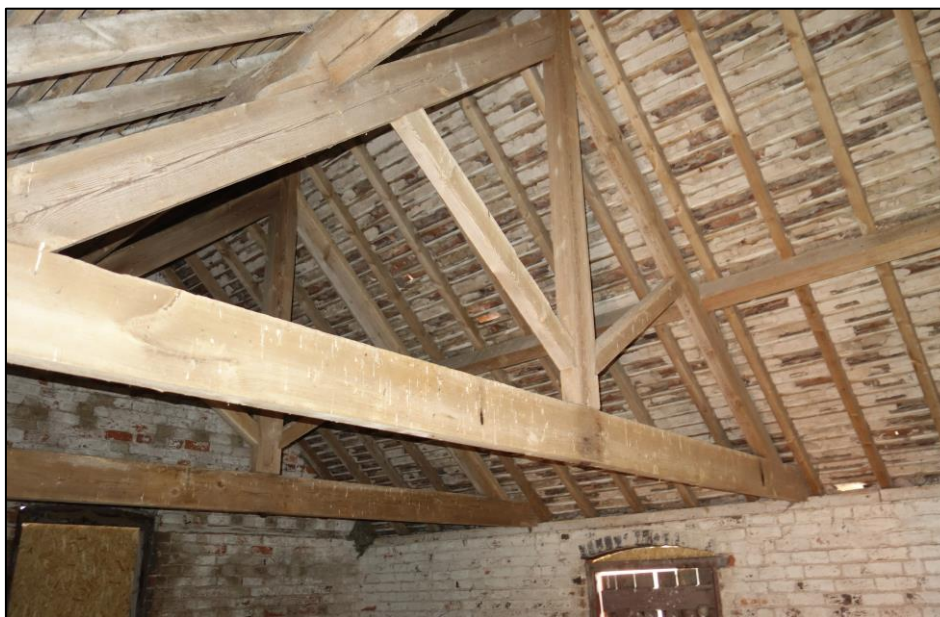
Plate 39: Internal view looking S showing detail of roof structure with central kingpost truss and angled struts in hayloft
