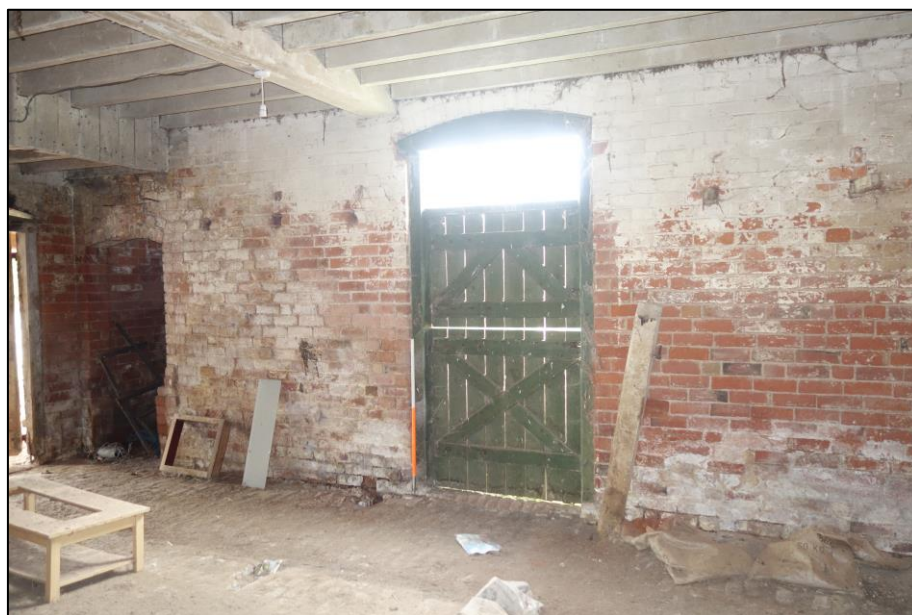
Plate 33: View looking N showing segmental-arched door with glazed overhead in NE wall of stable flanked by indentations for harness rails (with an intact harness rail to right of picture)
