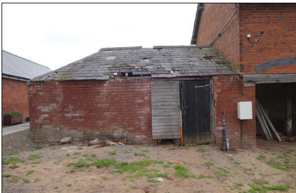
Plate 12: View looking SE showing front elevation of single-storey outbuilding with slate roof attached to NE end of granary/cartshed
