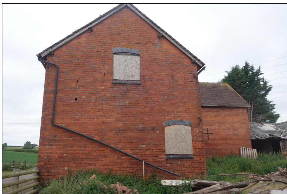
Plate 7: View looking NW showing SE-gable end of two storey stable range with bargeboarded gable
