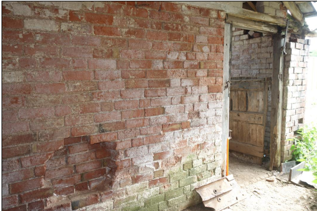
Plate 42: View looking E showing flat-arched door in SW-facing elevation of brick outbuilding to NE of cartshed
