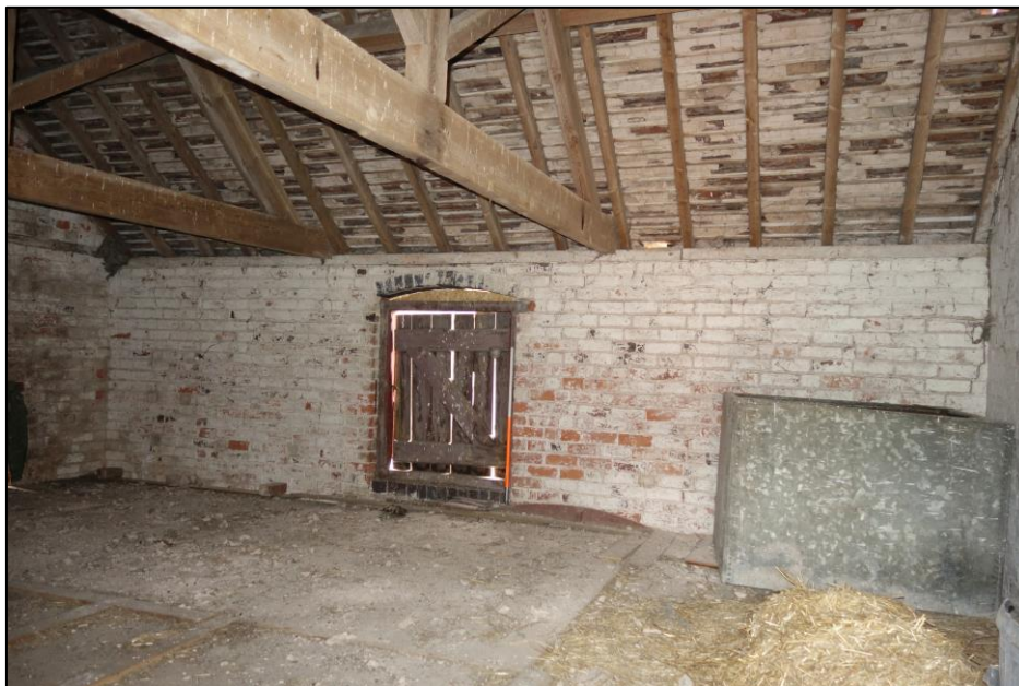
Plate 38: View looking SW showing interior of hayloft above stable with loading bay door in SW wall and metal tub (grain bin) to right of picture
