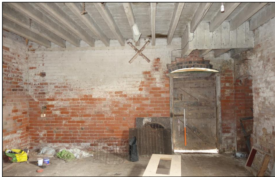
Plate 31: Internal view of stable range showing exposed ceiling joists and segmental-arched door in NW wall
