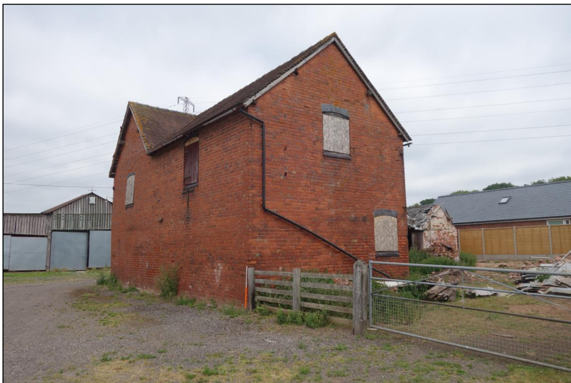
Plate 2: View looking NNW showing SE gable of two storey-stable range attached to rear of the granary/cartshed
