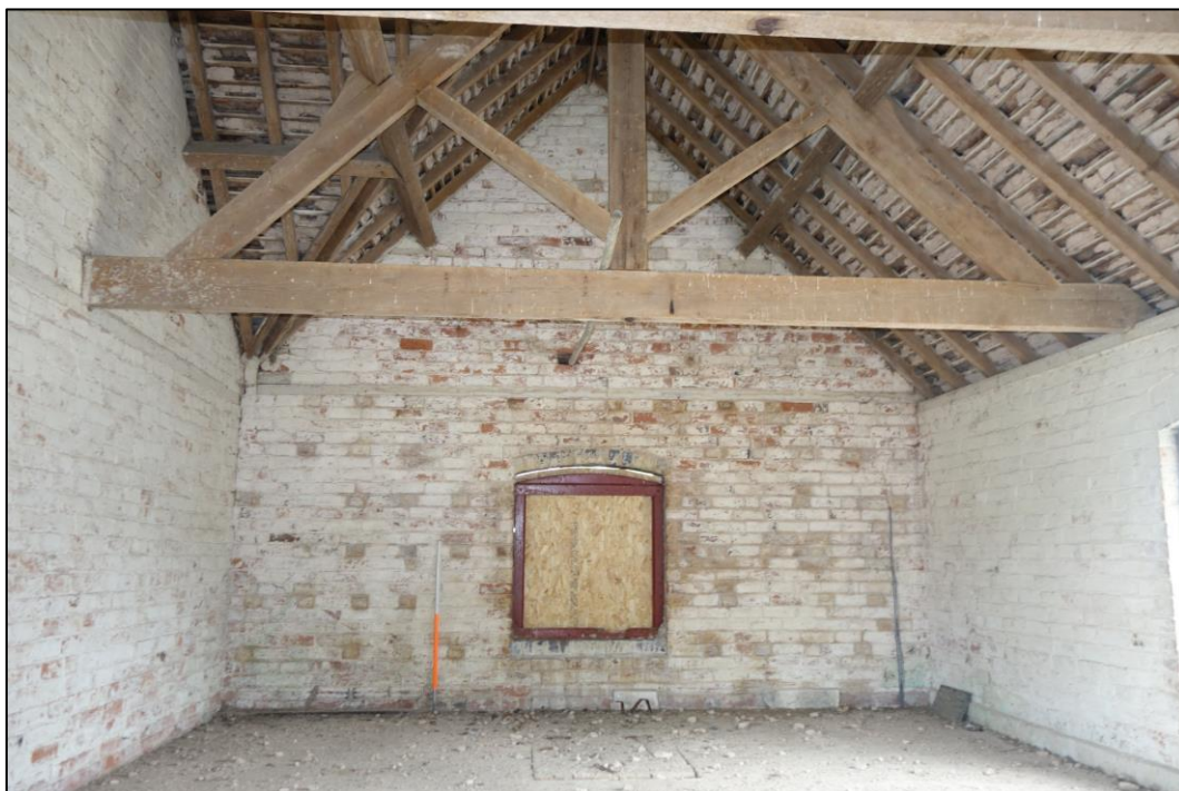
Plate 25: Internal view looking SW showing southwesternmost bay of granary with kingpost roof structure and segmental-arched window in SW wall
