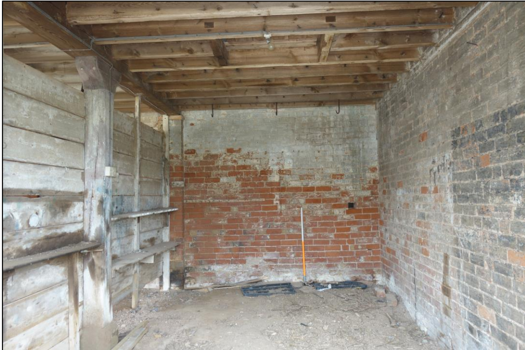
Plate 19: View looking SE showing interior of compartment within southwesternmost bay of cartshed, demarcated by horizontal wooden slats with shelving (to left of picture)
