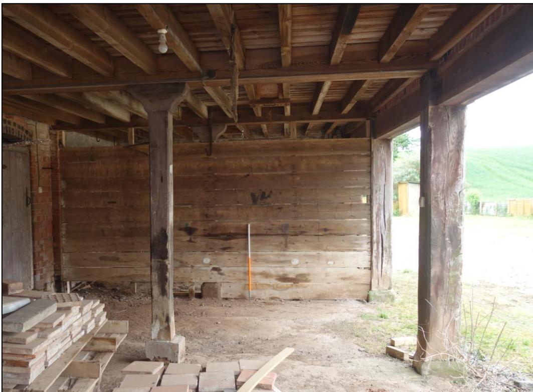
Plate 14: View looking SW showing interior of cartshed with arcade posts and a grain chute visible in the ceiling
