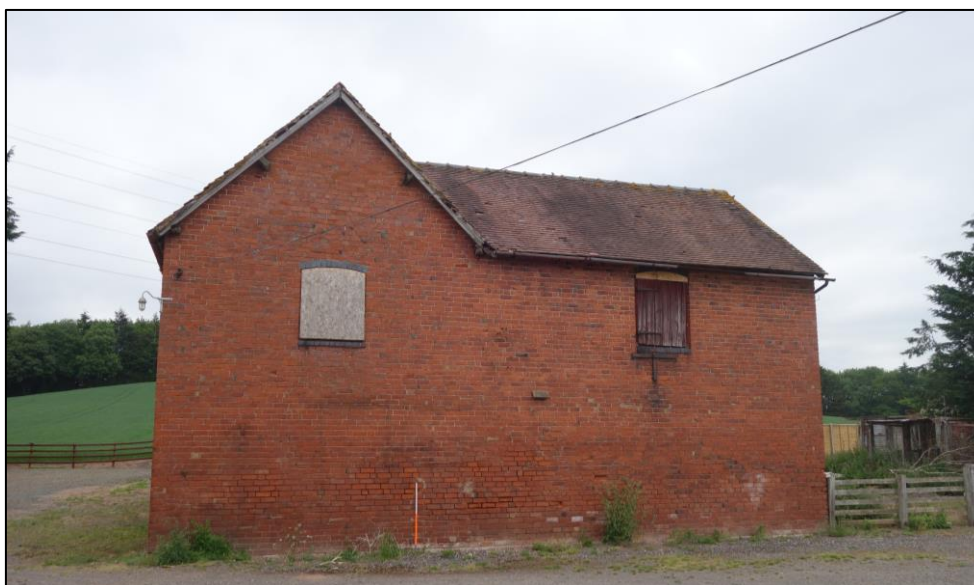
Plate 6: View looking NE showing SW-facing elevation of the granary/cartshed and attached two storey stable block
