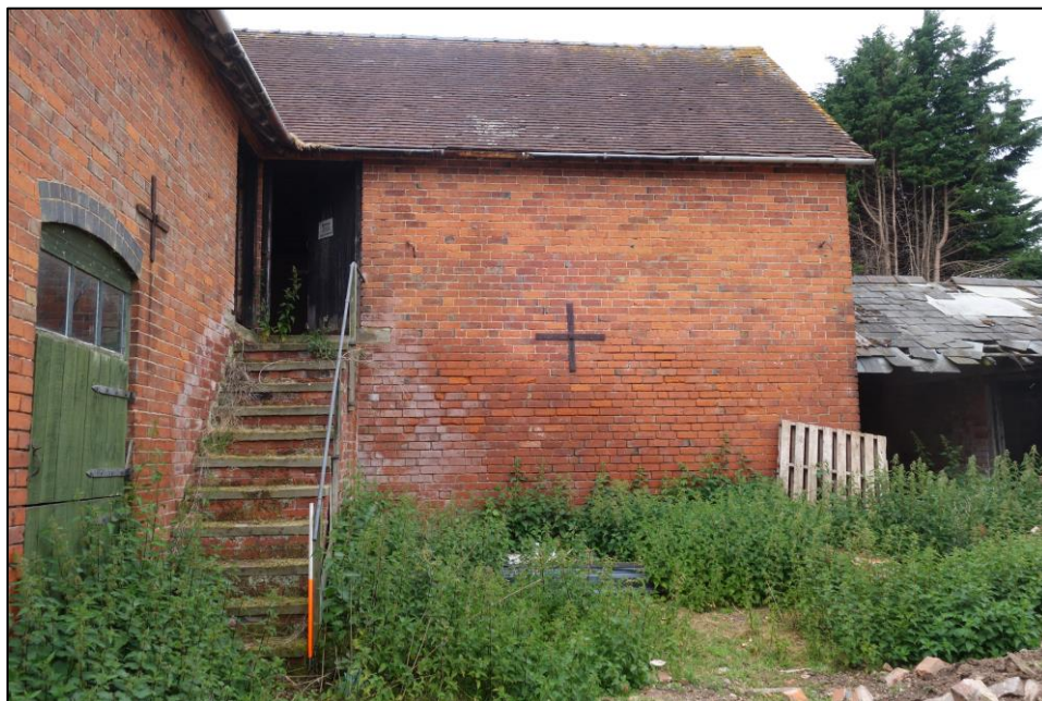
Plate 9: View looking NW showing rear elevation of granary/cartshed range and staircase leading up to granary and hayloft
