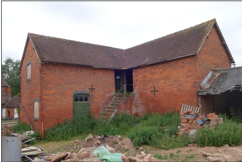
Plate 8: View looking W across former yard towards rear elevation of granary/cartshed and attached stable range with external staircase
