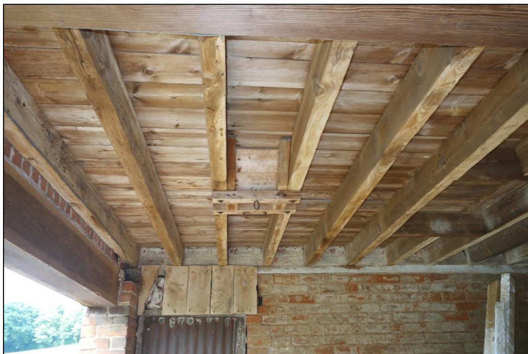
Plate 17: View looking NE showing detail of grain chute in ceiling of northeasternmost bay of cartshed with trap door visible to right of picture
