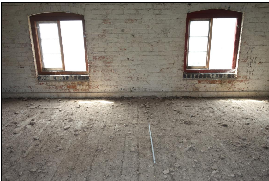
Plate 30: Internal view looking NW showing central two bays of granary lit by segmental-arched casement windows and rectangular grain chute in floor (in centre of picture)
