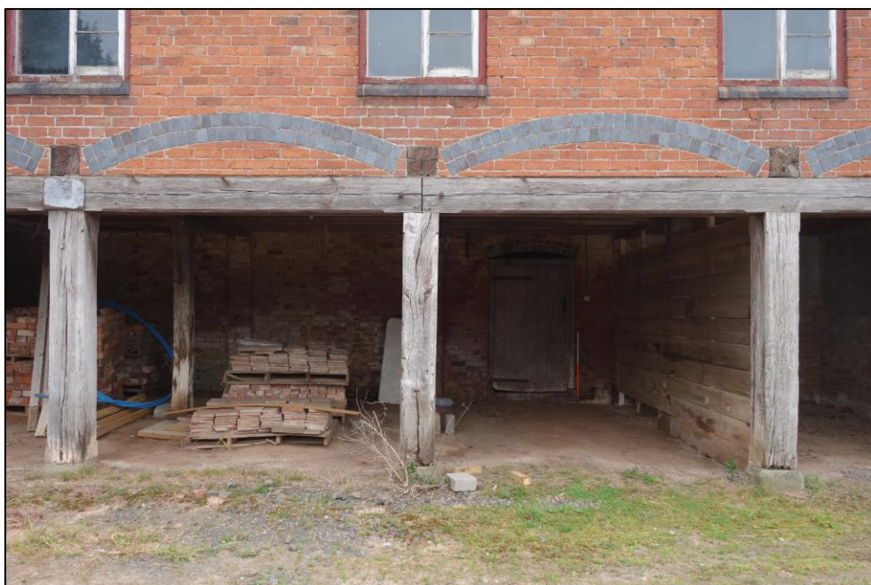
Plate 5: View looking SE showing detail of cartshed openings with stop-chamfered posts and lintel with segmental Staffordshire blue-brick arches above
