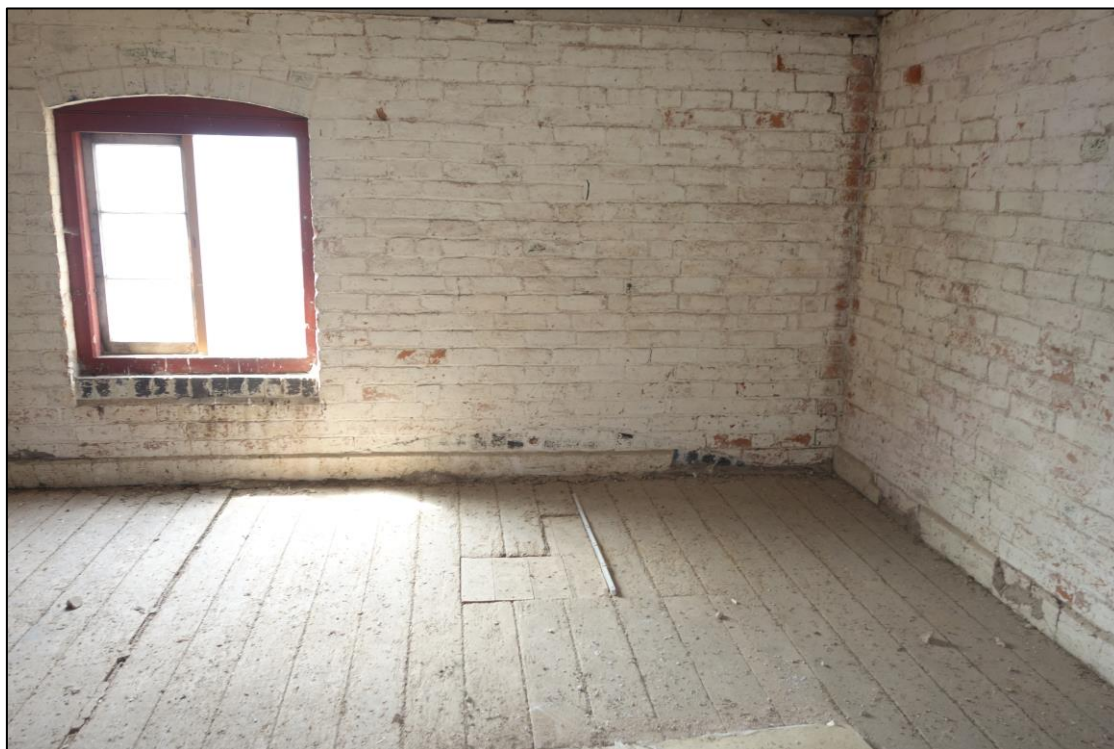
Plate 29: Internal view looking NW showing segmental-arched window and grain chute in northeasternmost bay of granary
