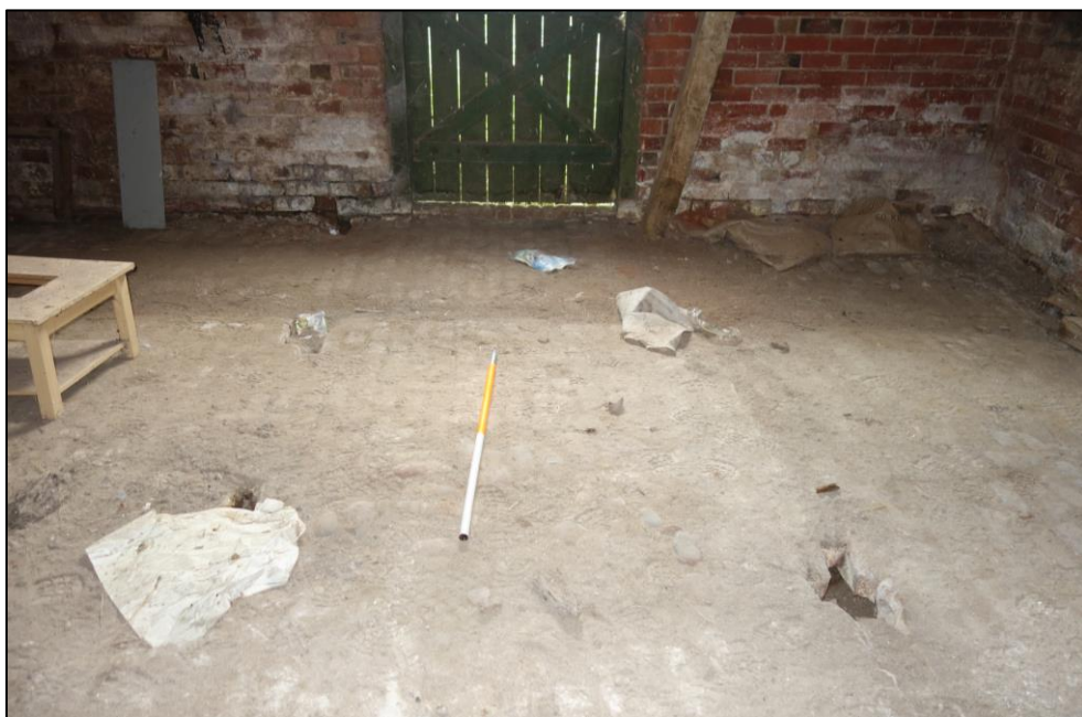
Plate 36: View looking NE showing detail of cobbled floor and drainage channel within stable range
