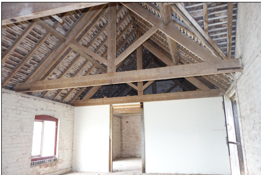
Plate 22: Internal view looking NE showing interior of granary with kingpost roof trusses and modern partition wall demarcating the NE compartment
