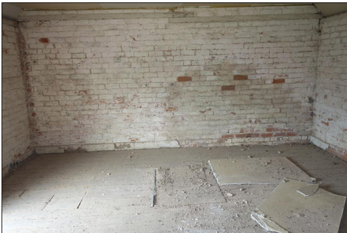
Plate 27: Internal view looking NE showing northeasternmost bay of granary with trap door and grain chute to left of picture
