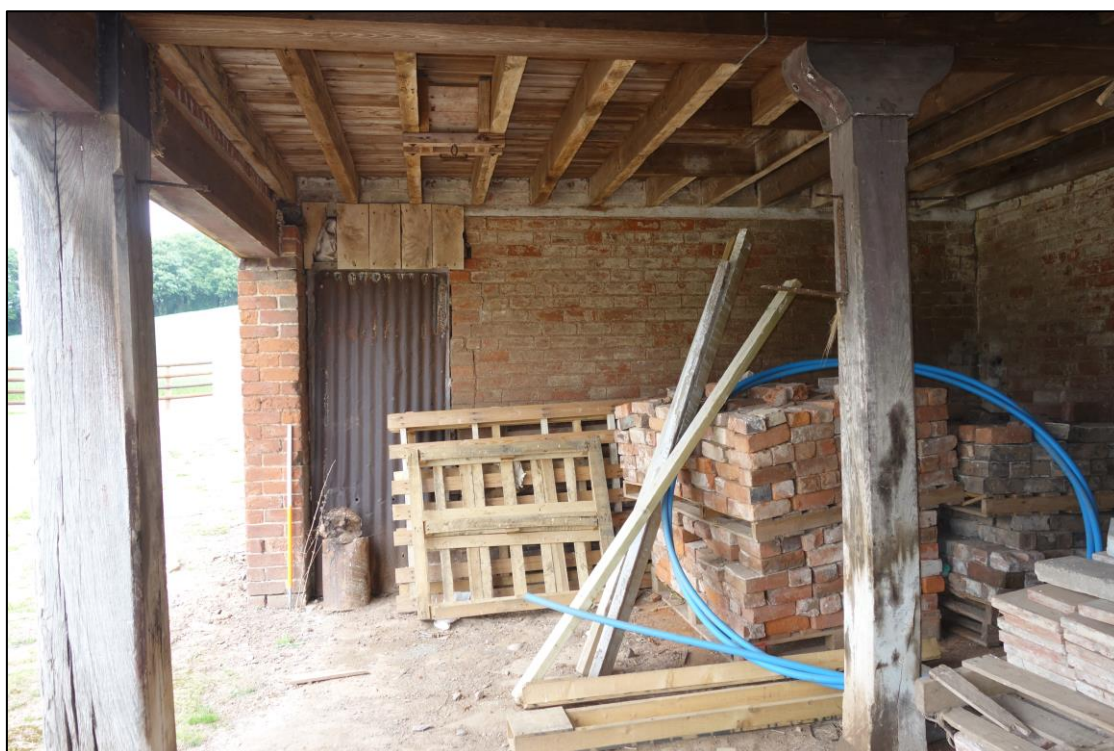
Plate 16: View looking NE showing northeasternmost bay of cartshed with grain chute and trapdoor in ceiling
