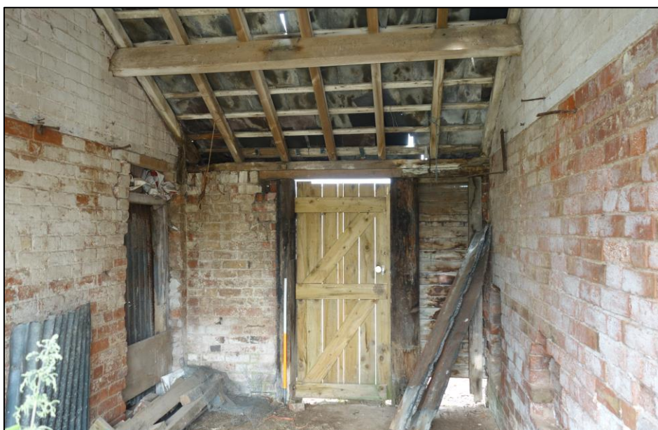
Plate 40: View looking NW showing interior of open-fronted shed/vestibule between cartshed and outbuilding
