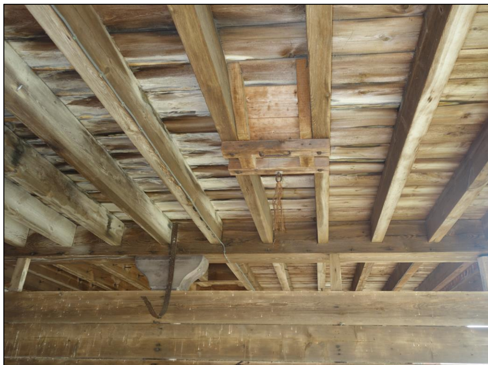
Plate 18: View looking SW showing detail of grain chute in cartshed bay opposite entrance to stable block
