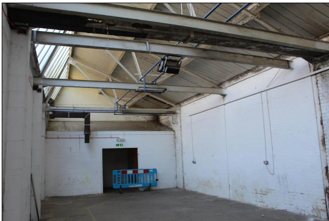
Plate 4: View N showing interior of central portion of former works building with steel transverse roof trusses
