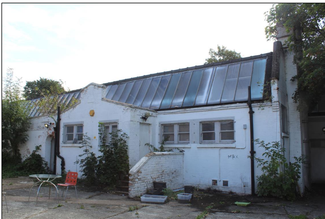
Plate 3: View NE showing W-facing elevation of former light industrial works building with central porch
