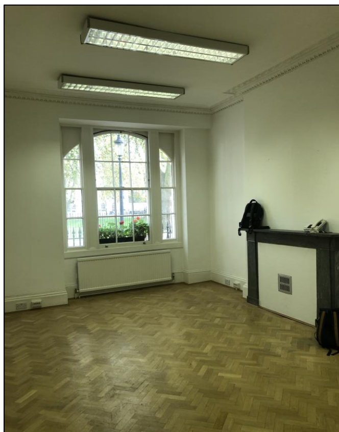
Plate 6: General view looking E showing front room on ground floor with fireplace visible to right of picture
