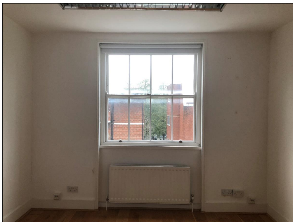
Plate 44: View looking W showing sash window in back room on third floor
