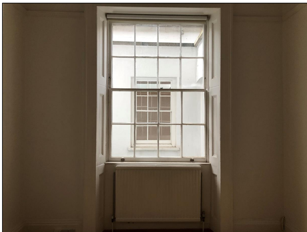
Plate 10: View looking W showing detail of sash window in ground floor back room
