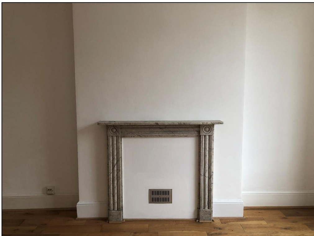
Plate 36: View looking S showing marble fireplace in S wall of back room on second floor
