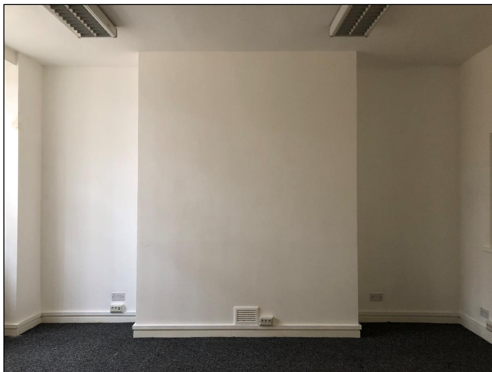
Plate 50: View looking S showing blocked chimneybreast in basement front room
