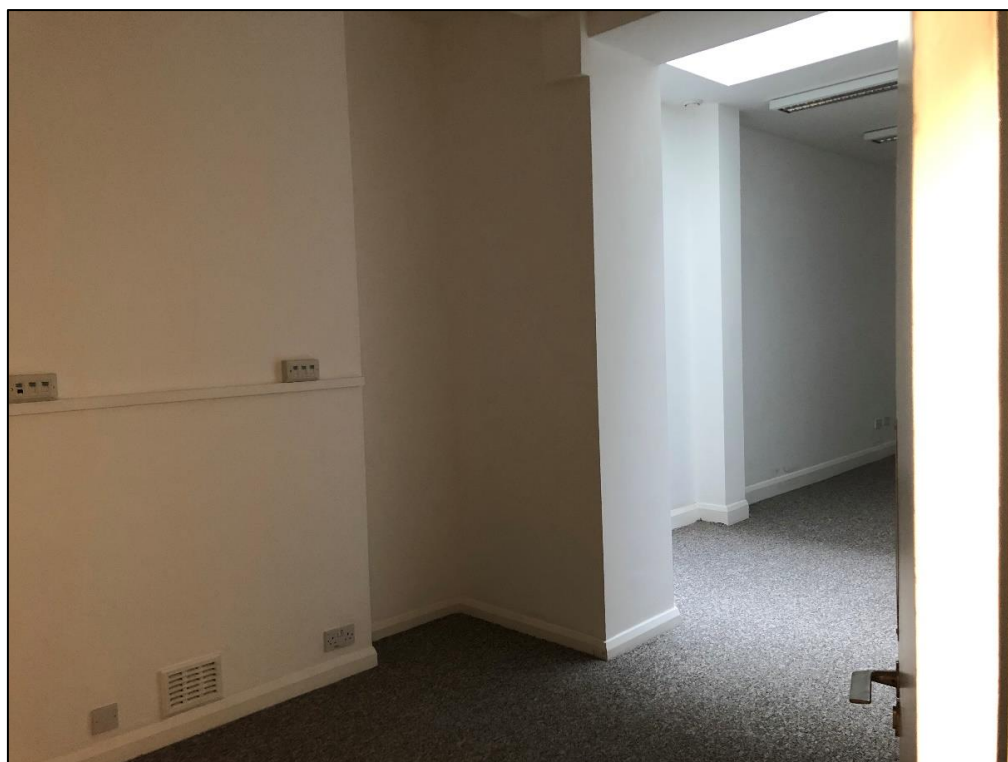
Plate 54: View looking SW showing blocked chimneybreast in S wall of basement room
