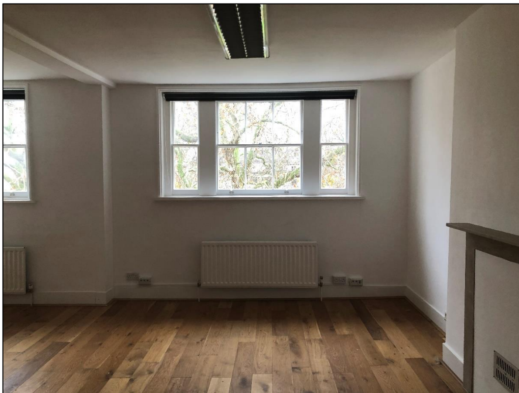
Plate 41: View looking E showing southern part of third floor front room, with wall stub visible to left of picture
