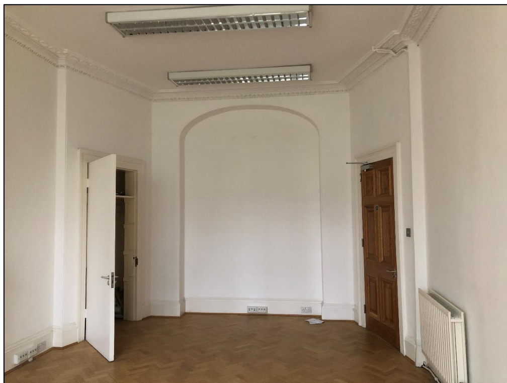
Plate 7: View looking W showing blocked archway in W wall of ground floor front room
