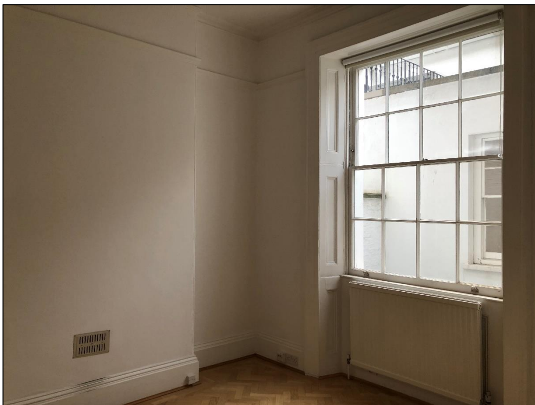
Plate 9: General view looking SW showing first floor back room with blocked fireplace and sash window
