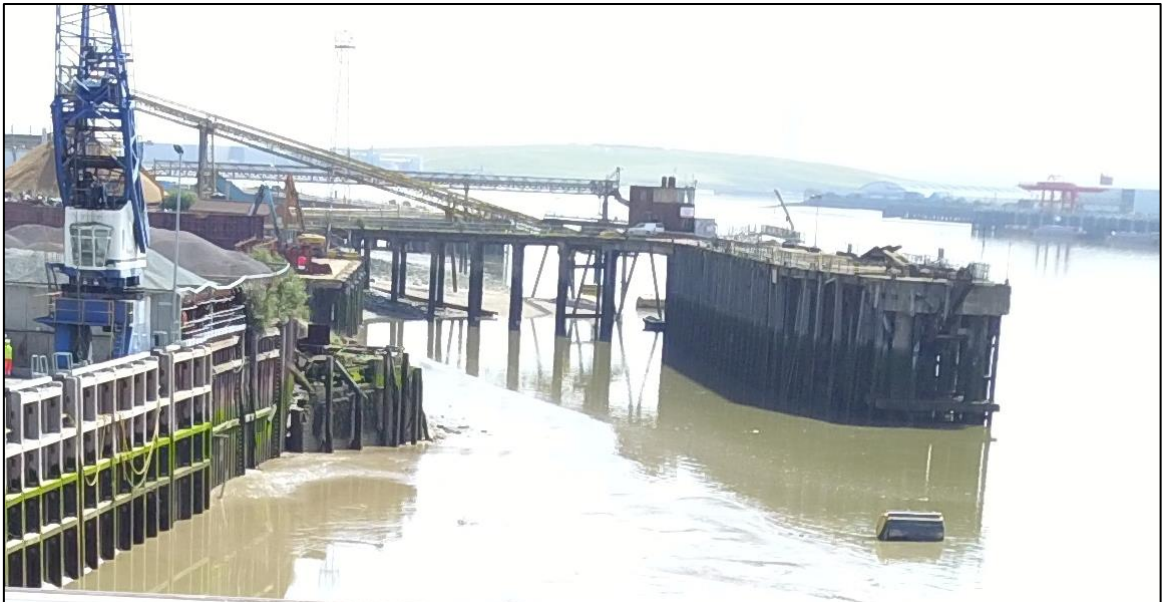
Plate 5: Close up view looking E showing Jetty No. 4 at Dagenham Dock and the approach structure
