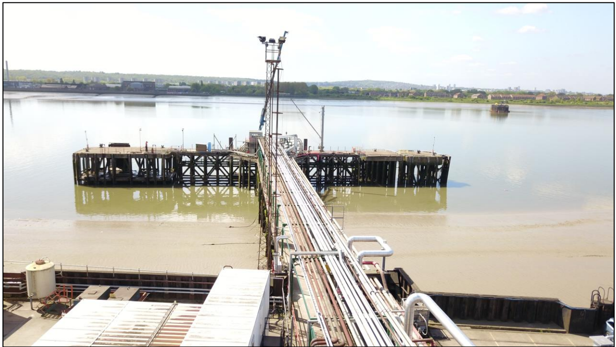
Plate 1: View looking S from landward side showing approach structure leading to Thunderer Jetty with the Crossness Pumping Station visible on the S side of the Thames
