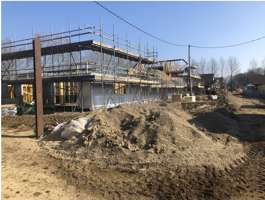
Plate 6: View looking NNE across development site showing vertical steel post (possible remnant of Building 2)
