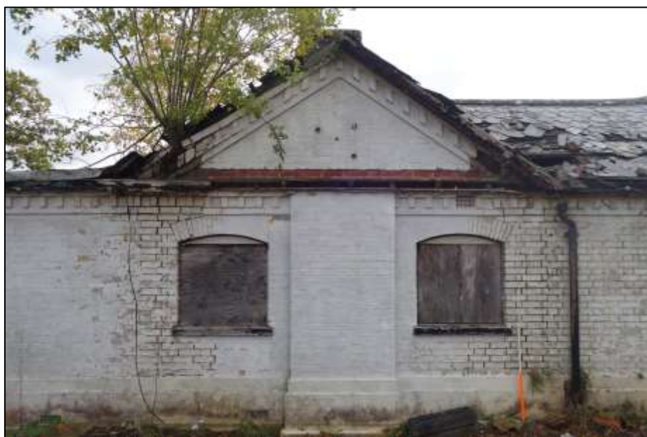
Plate 5: View looking SE showing detail of pedimented gable, chimneystack and windows in NW-facing elevation
