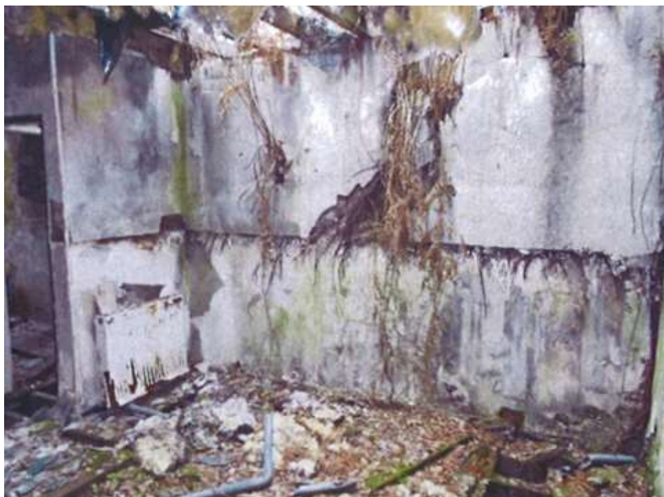
Plate 19: Internal view of NE room looking W showing interior partition wall and door leading to hallway (Reproduced by courtesy of the client)
