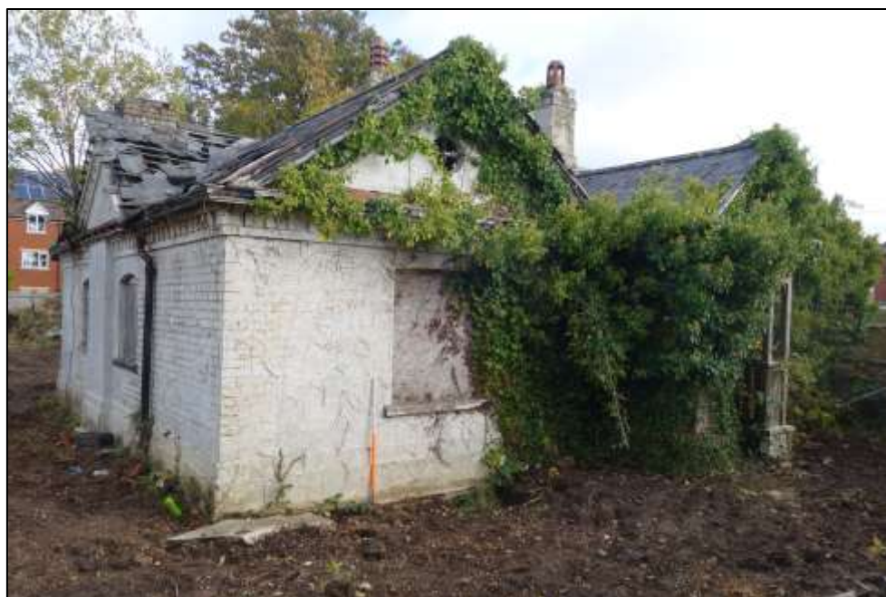
Plate 2: View looking SE showing principal SW facing elevation of The Lodge, heavily clad in ivy
