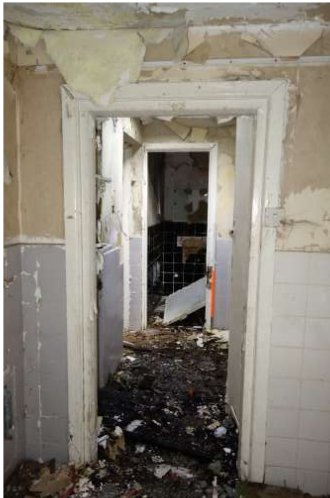
Plate 21: Interior view of modern annexe to rear of the Lodge looking NW, showing former bathroom
