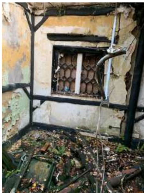
Plate 12: Internal view looking NW showing detail of latticed casement window in NW wall
