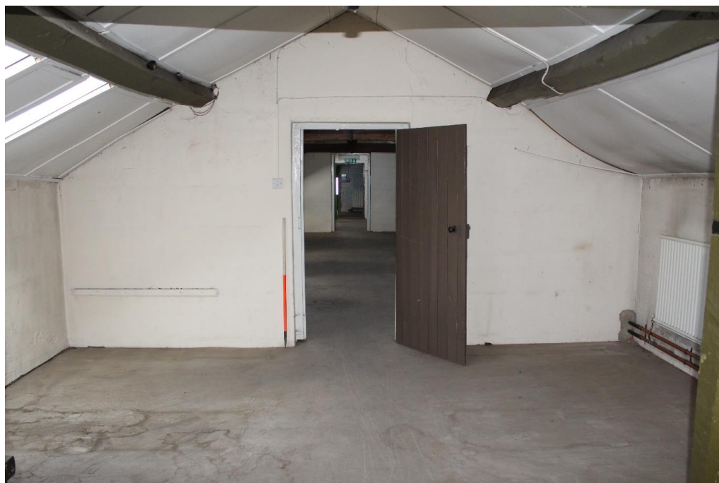
Plate 91: Internal view looking N along the attic compartments of the E wing
