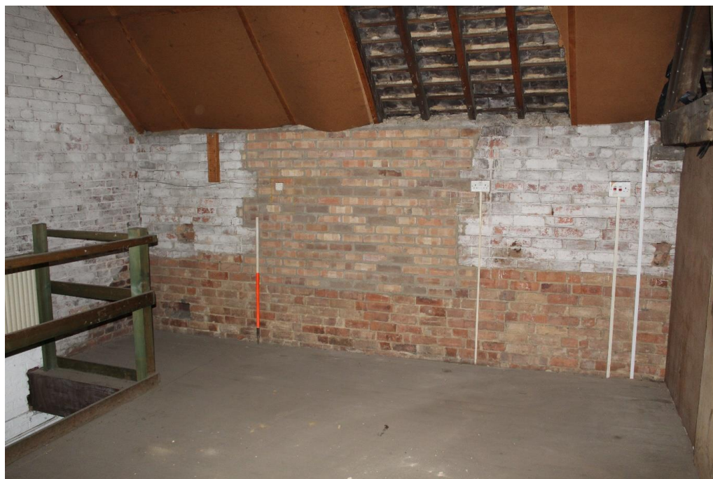
Plate 84: Internal view looking SSE within the central compartment of the first floor of the central range
