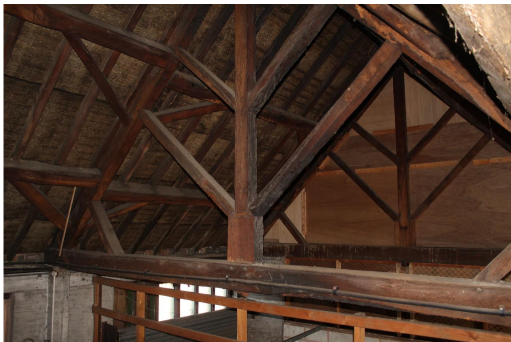
Plate 31: Internal view looking NW at the roof trusses within the W wing
