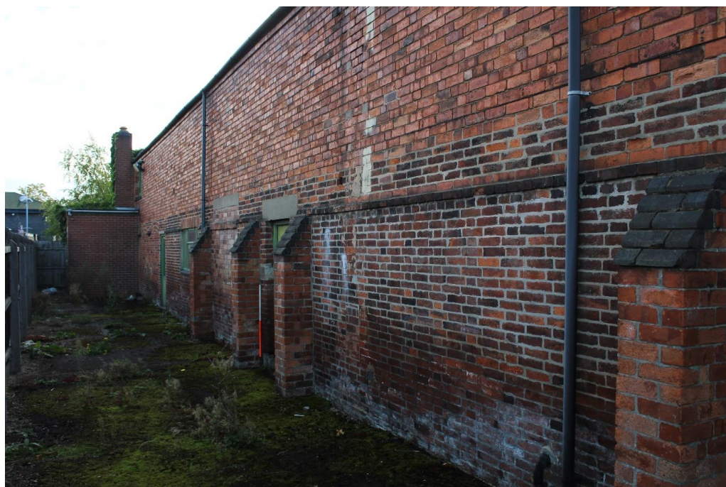
Pate 13: External view ESE of the north-facing elevation of the central range
