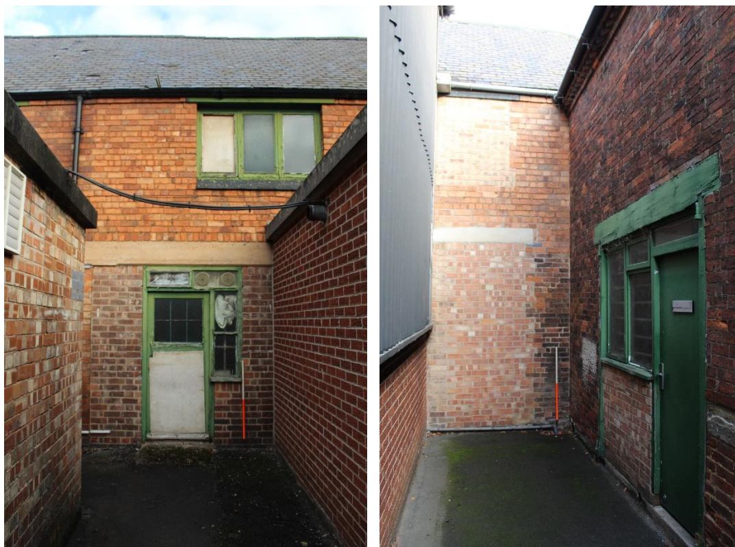
Plate 16 (left): External view looking N towards the south-facing elevation of the central range Plate 17 (right): External view looking N toward the south-facing elevation of the central range
