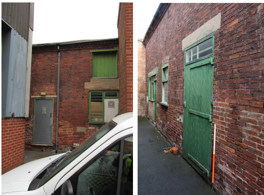
Plate 20 (left): External view looking E towards the west-facing elevation of the E wing Plate 21 (right): External view looking NNE towards the west-facing elevation of the E wing
