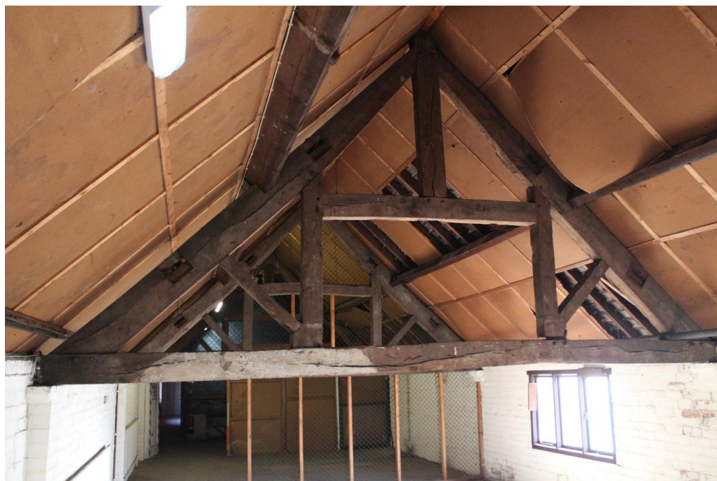
Plate 82: Internal view looking ESE within the central compartment of the first floor of the central range
