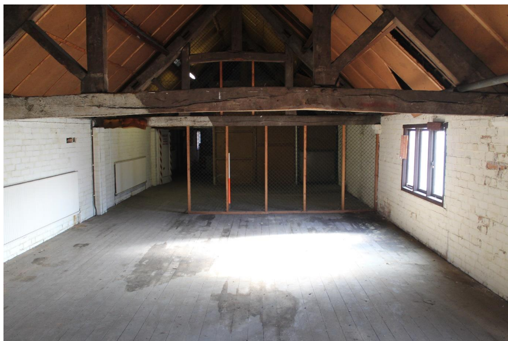
Plate 81: Internal view looking E within the central compartment of the first floor of the central range
