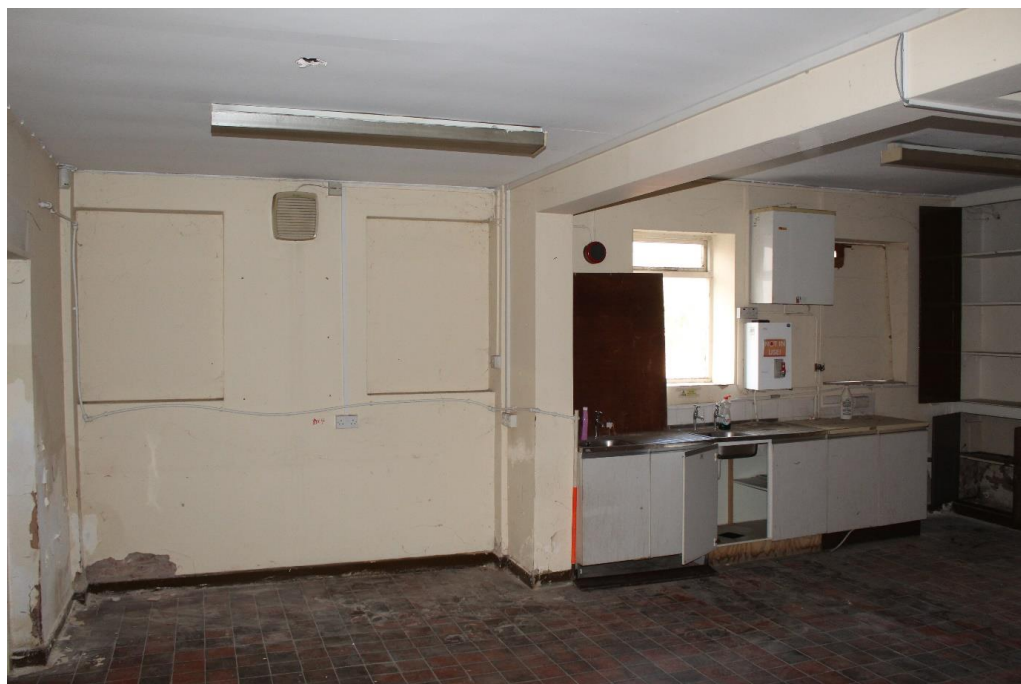
Plate 37: Internal view looking WNW within the fourth compartment of the W wing
