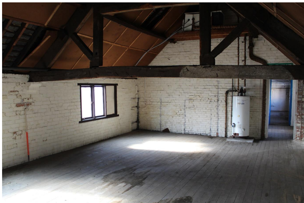
Plate 80: Internal view looking WSW within the central compartment of the first floor of the central range
