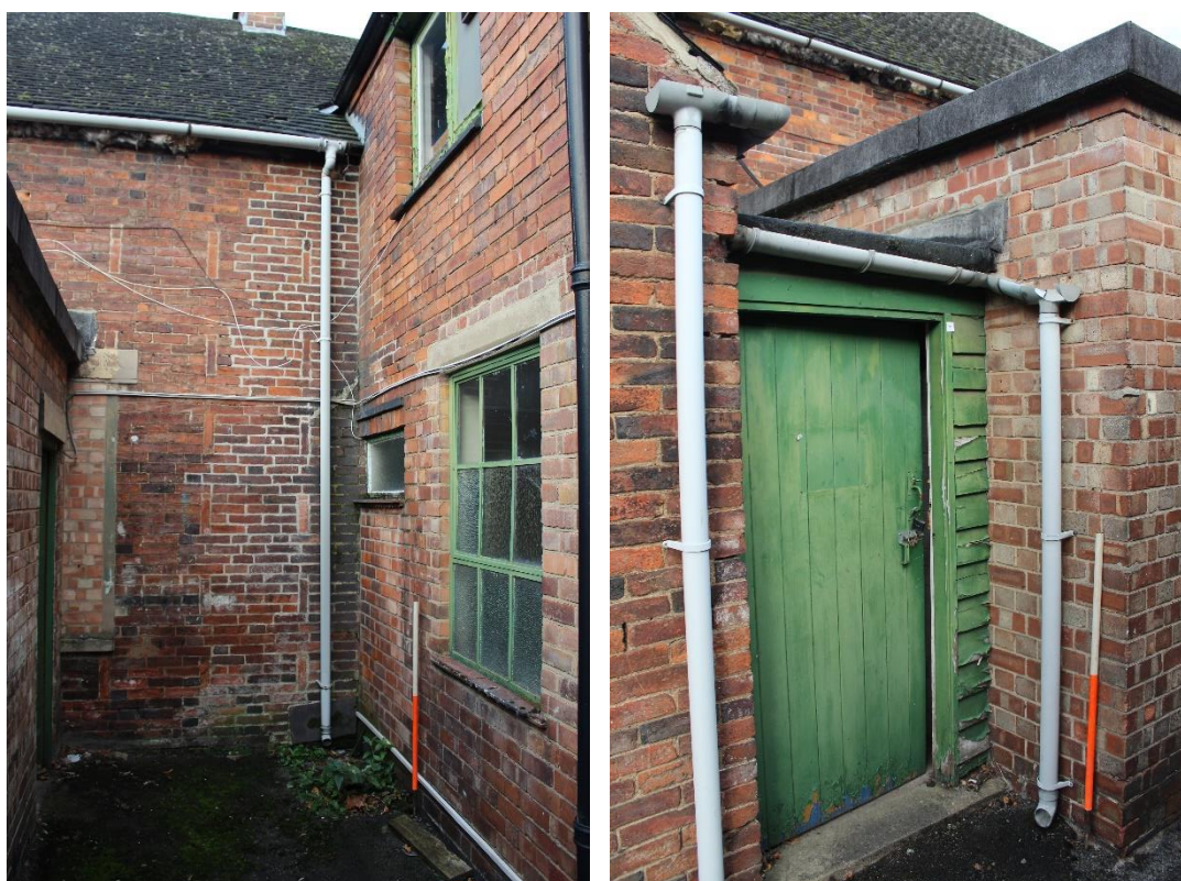
Plate 8 (left): External view looking WSW showing the east-facing elevation of the W wing Plate 9 (right): External view looking NW showing the east-facing elevation of the W wing
