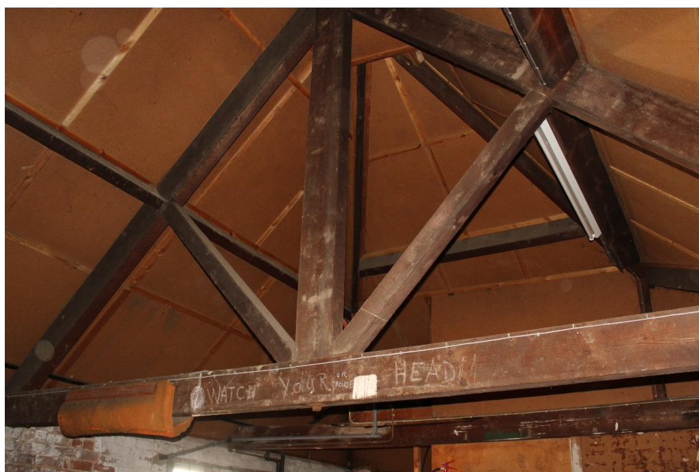
Plate 77: Internal view looking NE within the E compartment of the first floor of the central range
