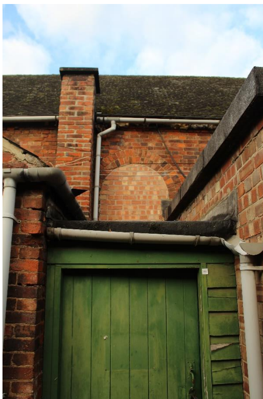
Plate 10: External view looking W showing a blocked window within the east-facing elevation of the W wing
