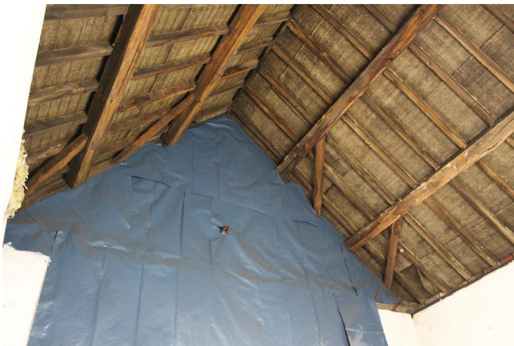
Plate 33: Internal view looking SSE at the roof structure within the third compartment of the W wing
