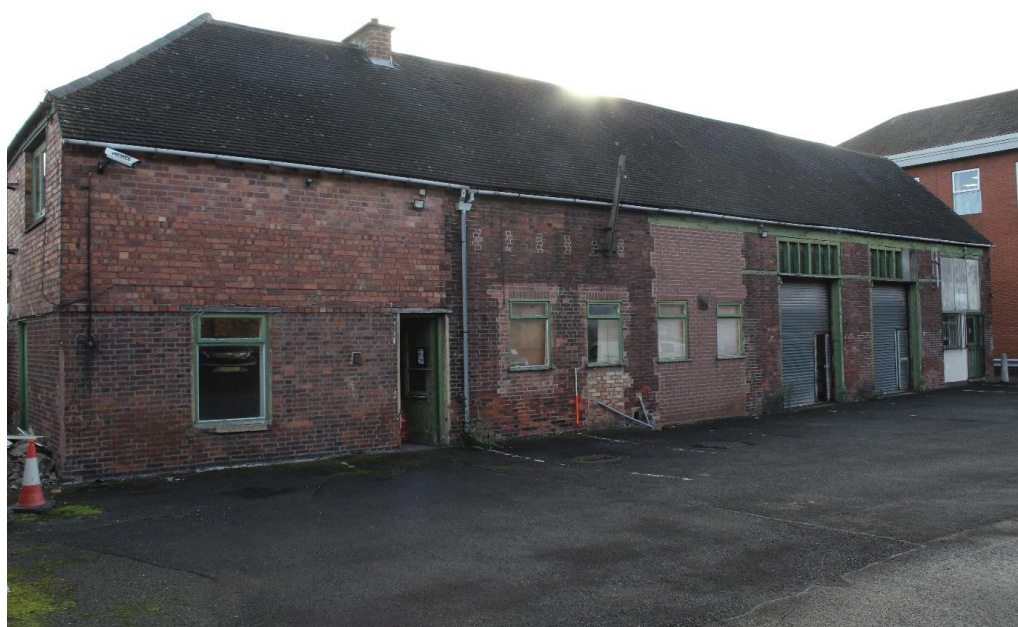
Plate 4: External view looking WSW showing the principal west-facing elevation of the western wing
