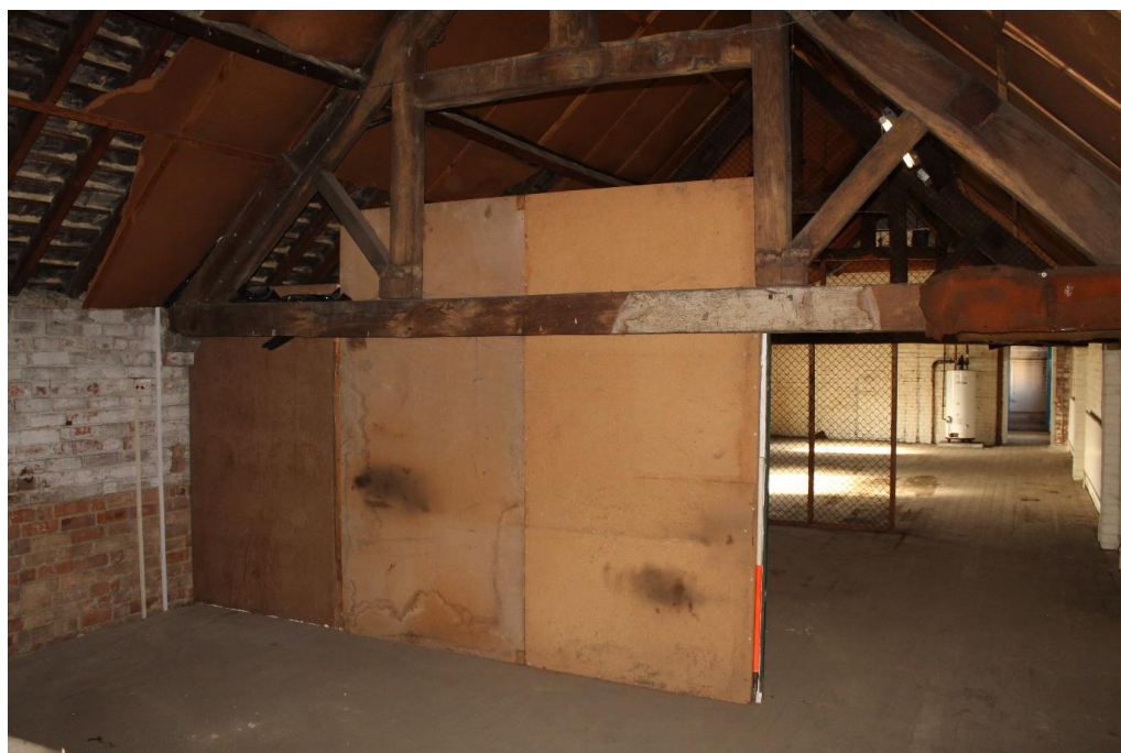
Plate 79: Internal view looking WSW within the central compartment of the first floor of the central range
