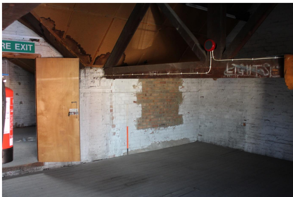
Plate 74: Internal view looking SSE within the E compartment of the first floor of the central range
