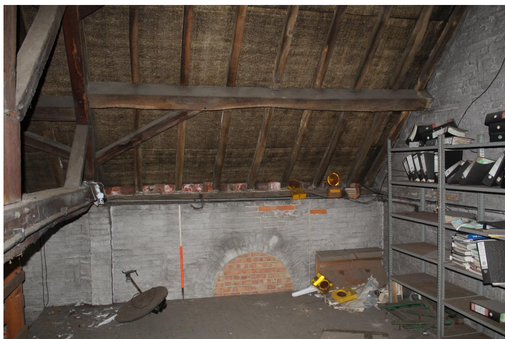
Plate 30: Internal view looking E within the mezzanine floor of the W wing
