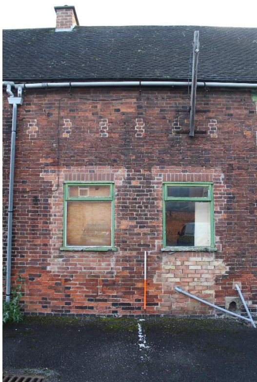
Plate 5: External view looking E towards the 5 th bay within the western wing
