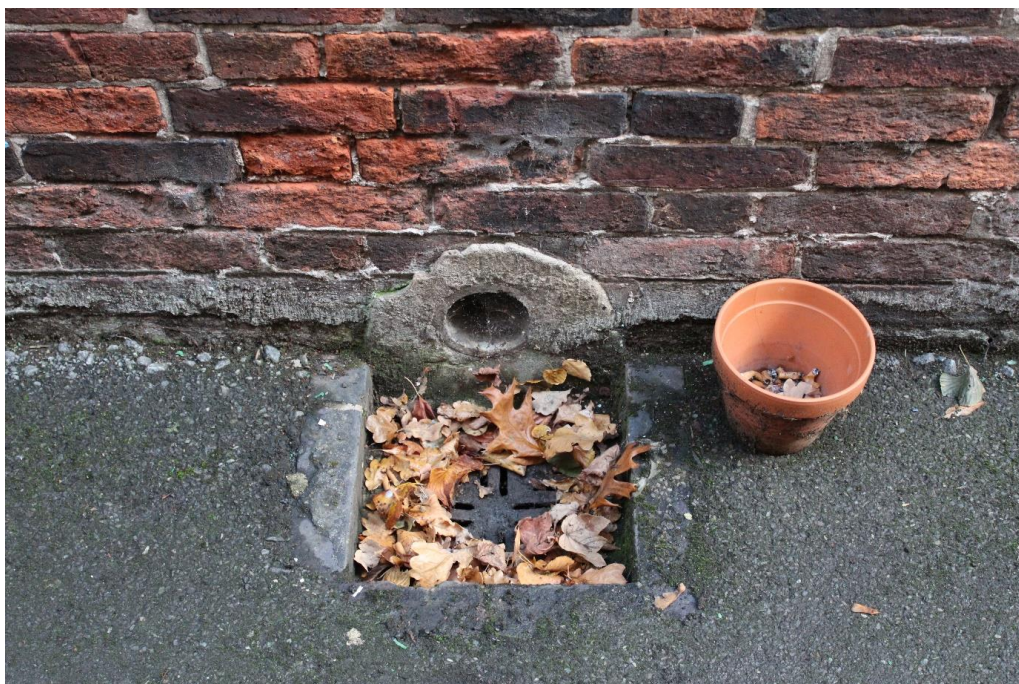
Plate 22: External view looking E towards a drain within the west-facing elevation of the E wing
