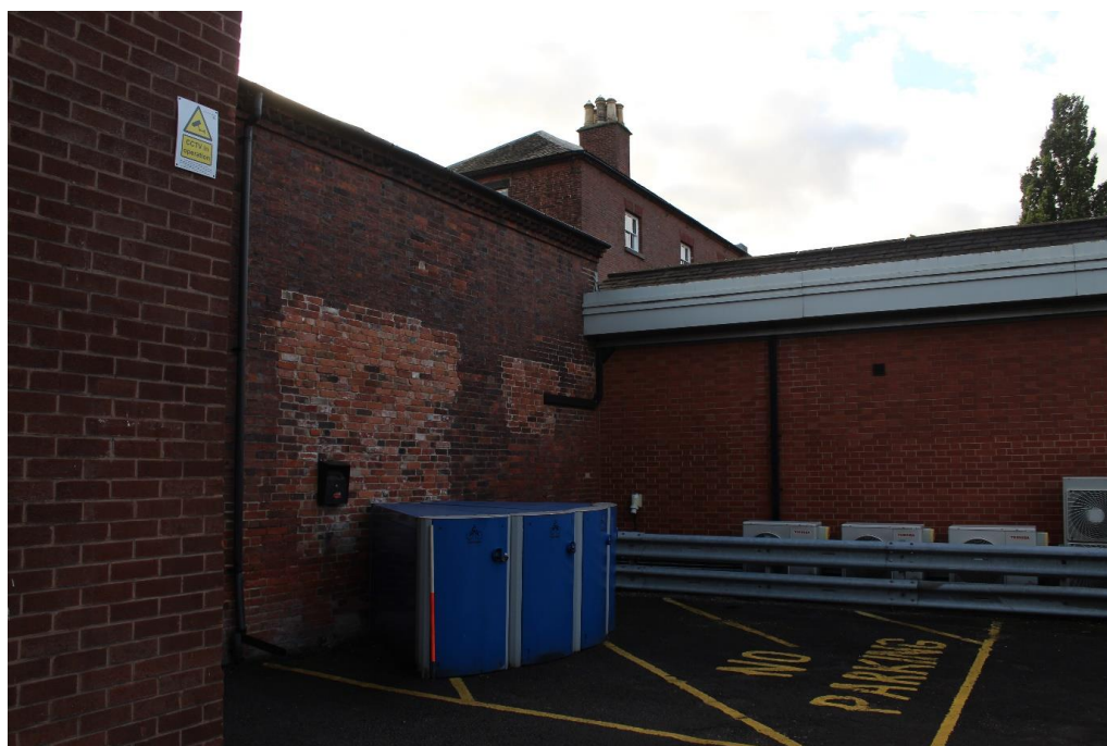
Plate 19: External view looking SE towards the adjoining modern office block on the E wing
