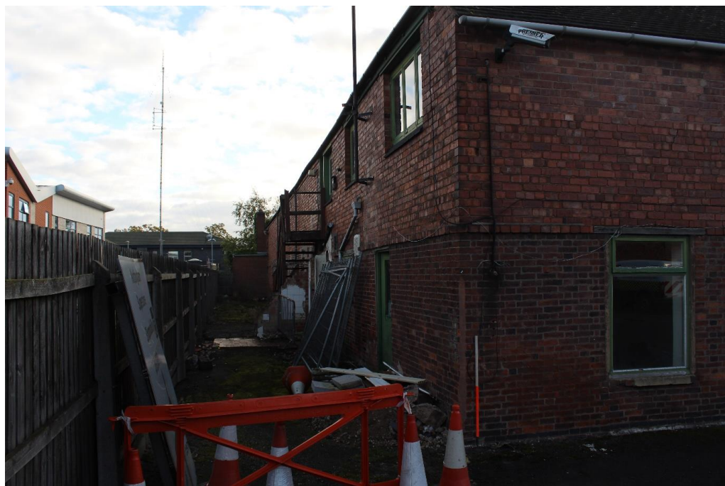
Pate 12: External view ESE of the north-facing elevation of the central range
