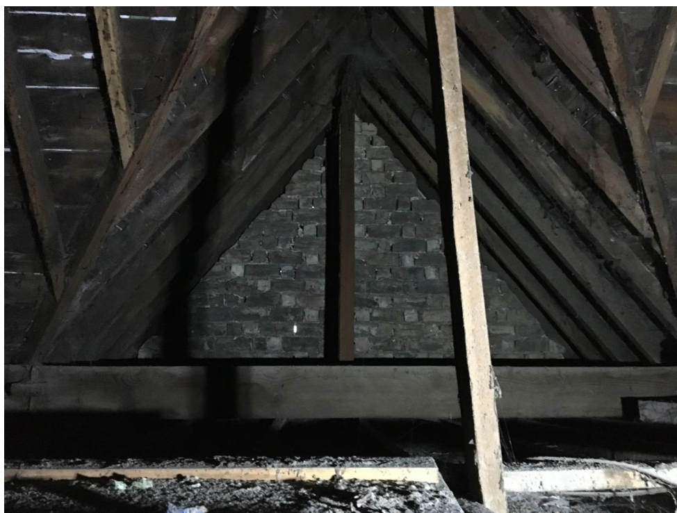
Plate 48: View W showing detail of gabled roof construction in loft above first floor
