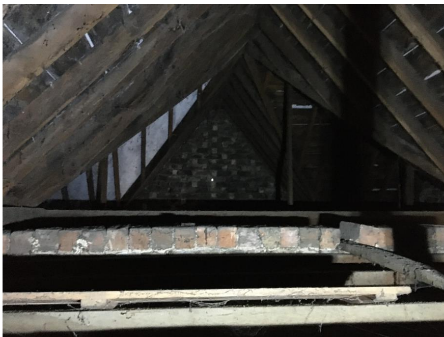
Plate 47: View S showing detail of loft space over S half of first floor
