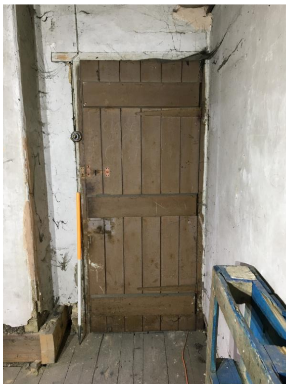
Plate 34: View N showing detail of plank and batten door leading to room to S of main compartment
