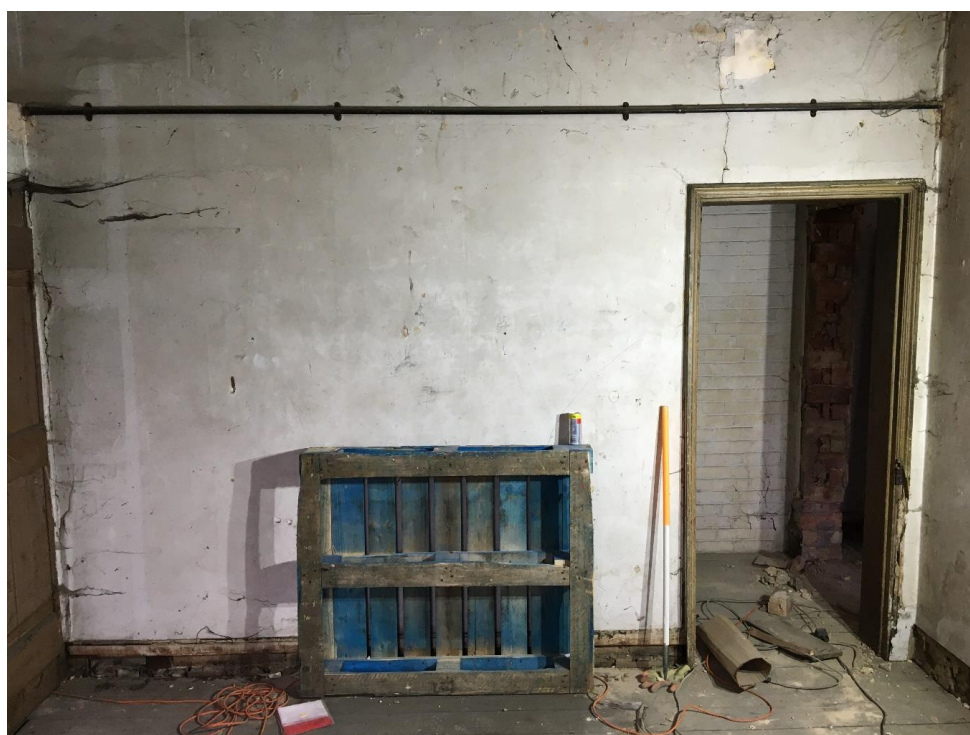
Plate 38: View looking E showing E wall of room to S of main compartment with doorway leading to room in southernmost bay (to right of picture)
