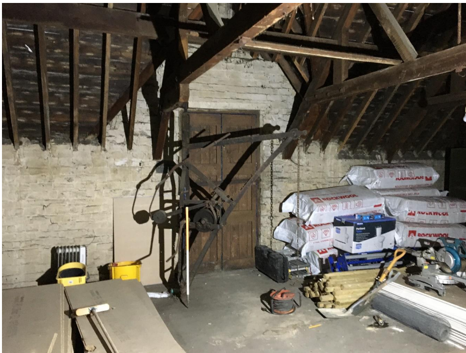
Plate 27: Internal view looking WNW showing central bay of first floor compartment with winch structure and loading bay door
