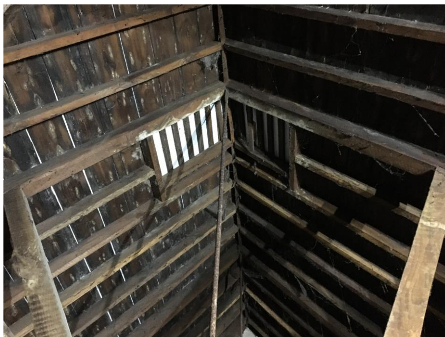
Plate 24: View showing ventilation flue in roof structure towards N end of main compartment
