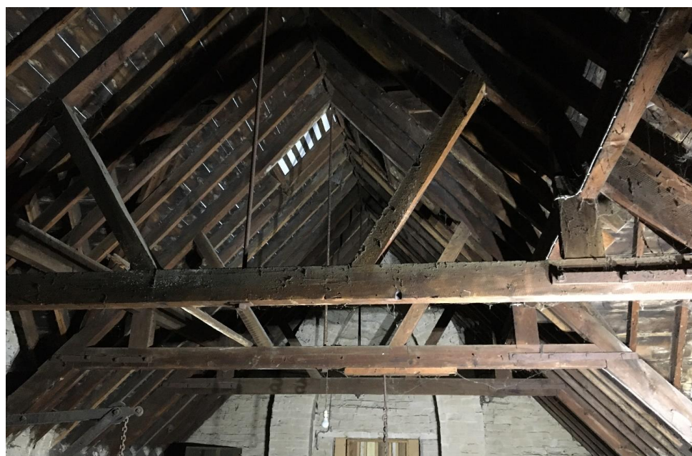
Plate 23: View NNW showing detail of queen-post trusses in central and northern bays of the main compartment on the first floor
