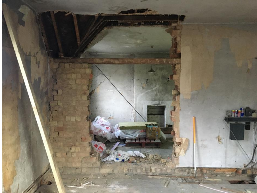
Plate 40: viewed N showing N wall of southernmost room on first floor with exposed brickwork
