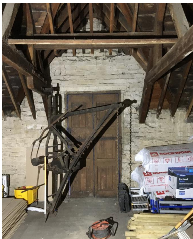
Plate 31: View looking W showing detail of winch structure within louvred central bay of first floor compartment
