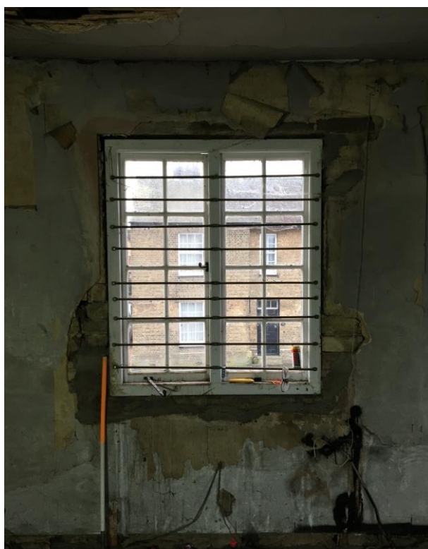
Plate 43: View S showing detail of two-light casement window in S wall of southernmost room on first floor
