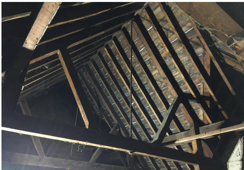
Plate 26: Internal view looking SE showing detail of queen-post roof trusses in southernmost portion of main three-bay compartment on first floor
