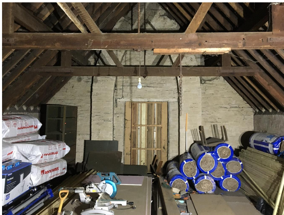
Plate 30: View looking N showing N bay of main compartment on first floor with loading bay door
