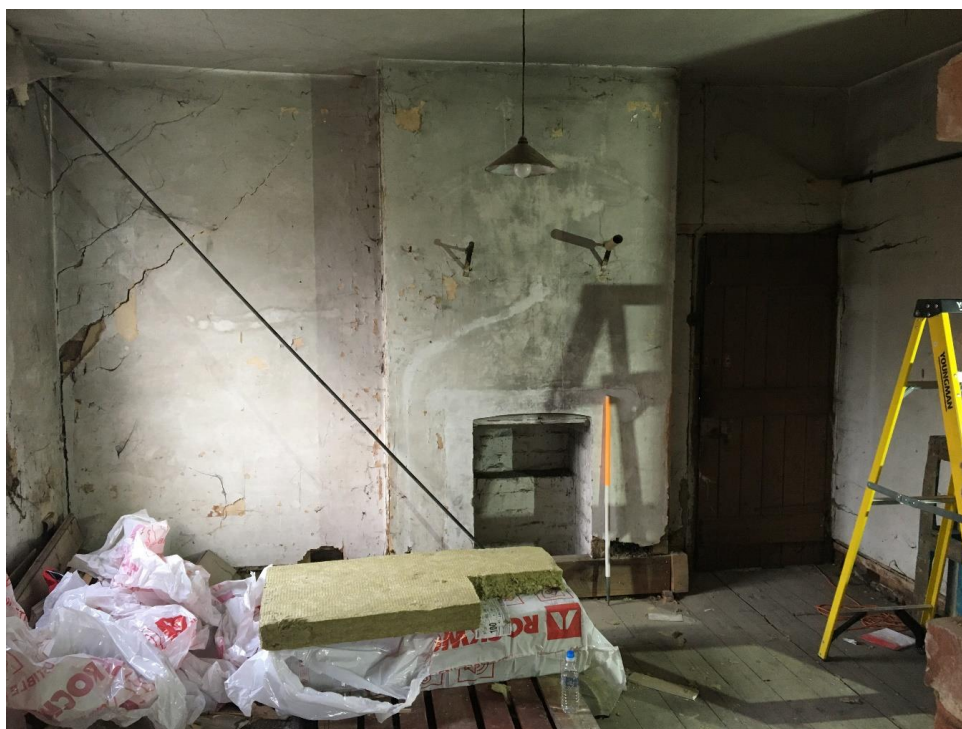
Plate 35: View N showing N wall of room to S of main compartment, showing fireplace
