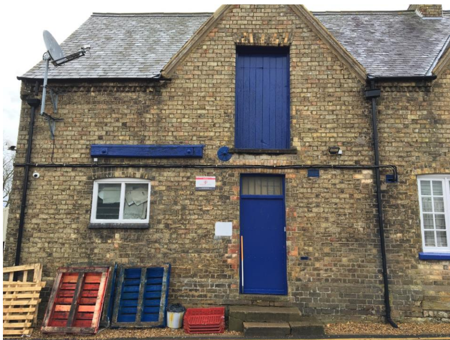
Plate 7: Viewed E showing detail of northernmost bays of W-facing elevation with loading bay door at first floor level
