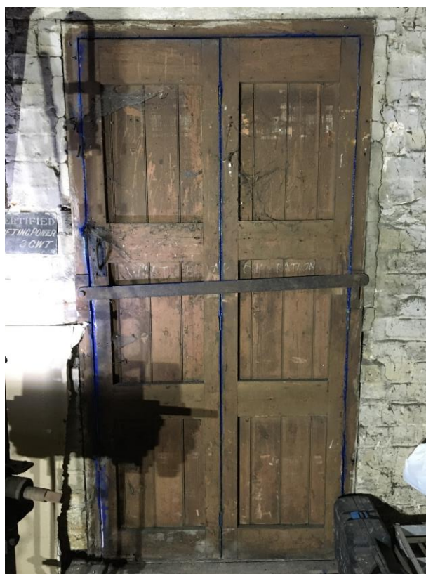
Plate 26: View W showing detail of loading bay door in W wall of central bay of main compartment (with winch to left of picture)
