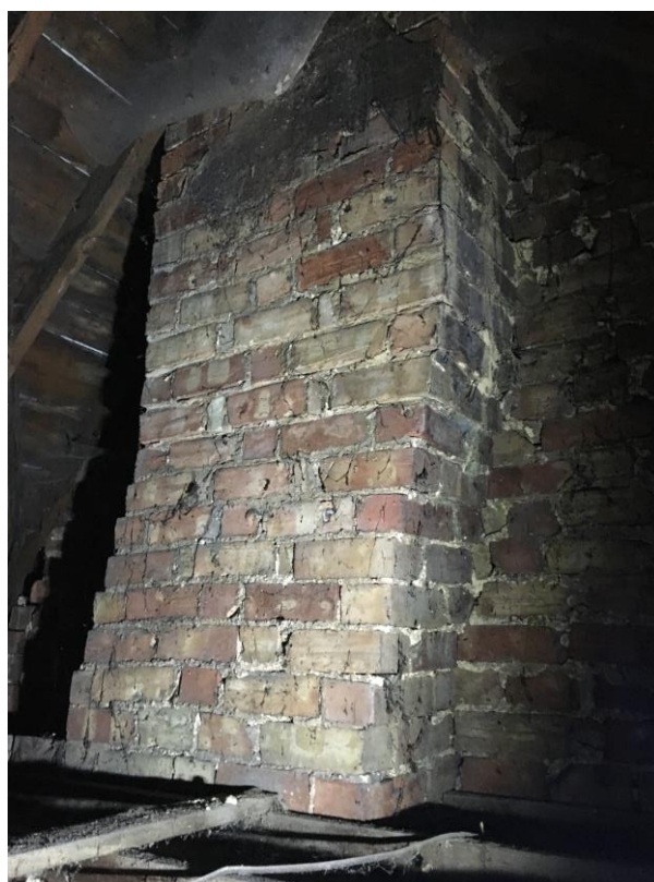
Plate 49: View NW showing detail of central chimneystack in loft over first floor
