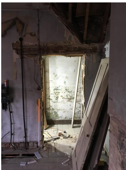
Plate 39: View N showing doorway in S wall of southernmost room on first floor
