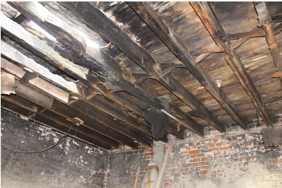
Plate 17: Internal view NW of ceiling joists and exposed floorboards within office compartment
