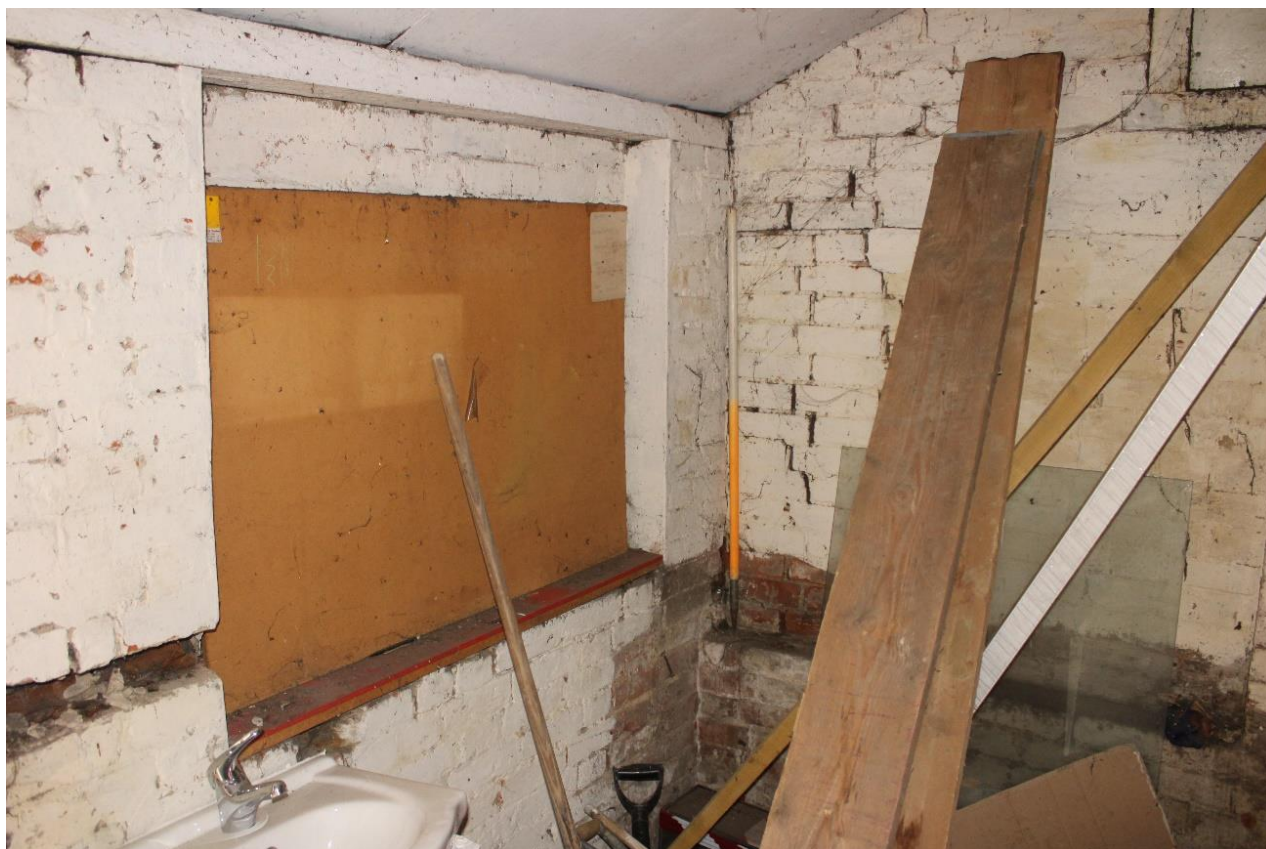
Plate 24: Internal view SW of blocked window in S wall of storage room
