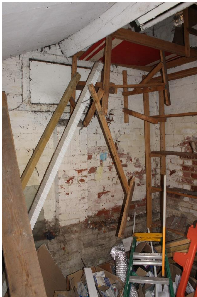
Plate 23: Internal view WNW of blocked window in W wall of storage room
