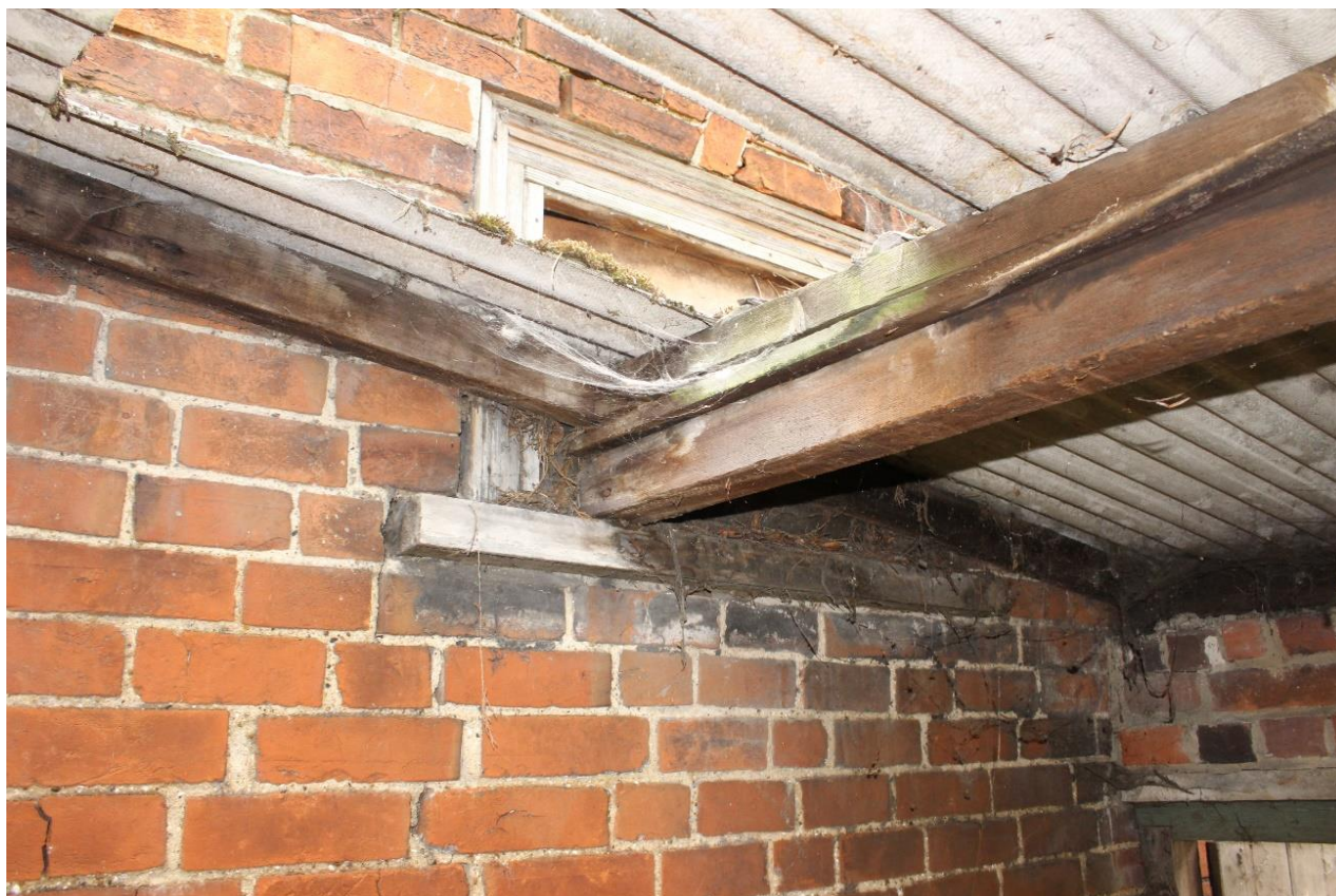
Plate 27: Internal view ESE of blocked window in E wall of storage room
