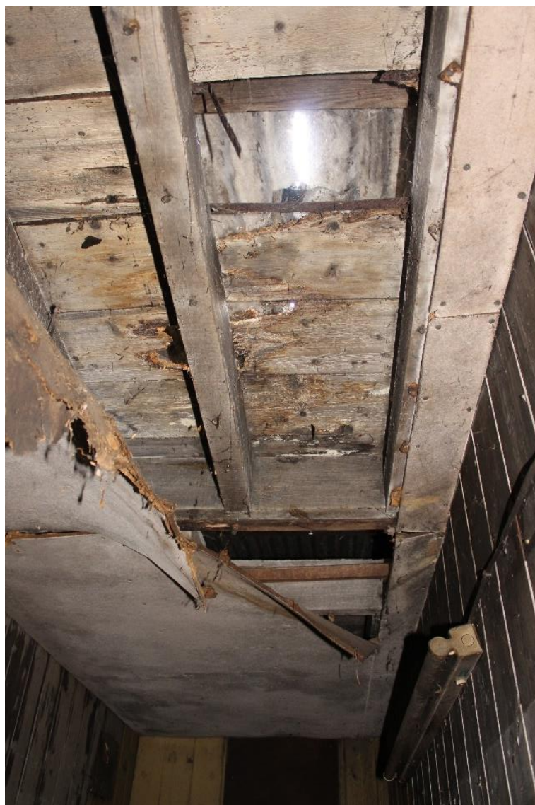
Plate 21: Internal view NNW of ceiling joists within the storage area adjoining office compartment
